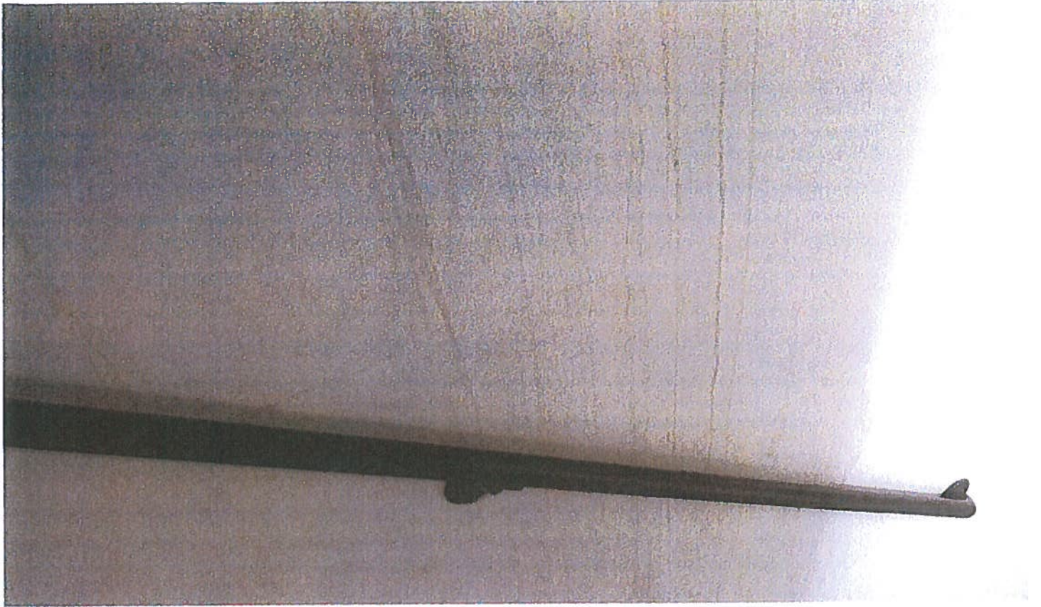
Photo 3: Apparent moisture staining on the perimeter wall of the stairwell.
