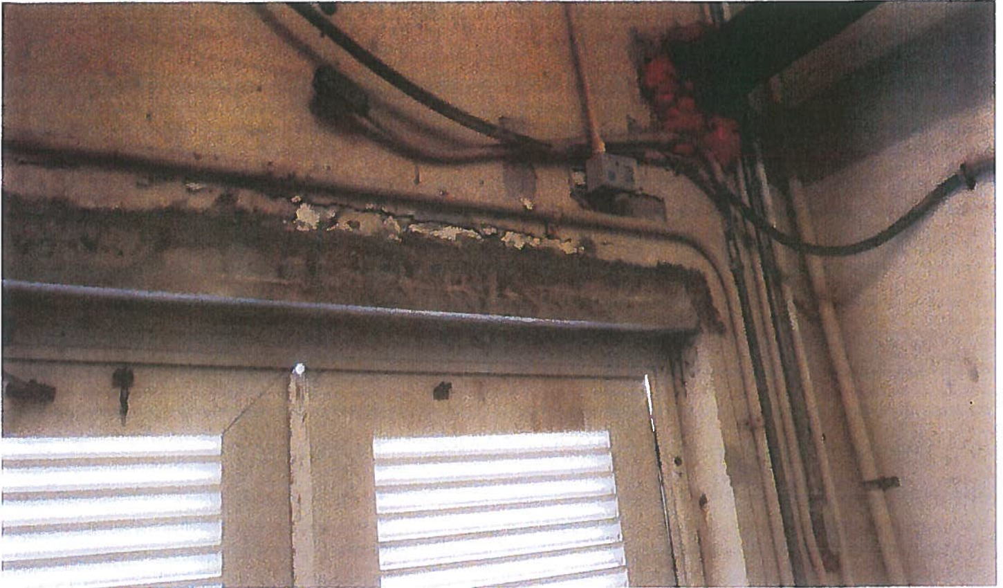
Photo 1: Cracking and spalling of the concrete header of the ground floor equipment room.
