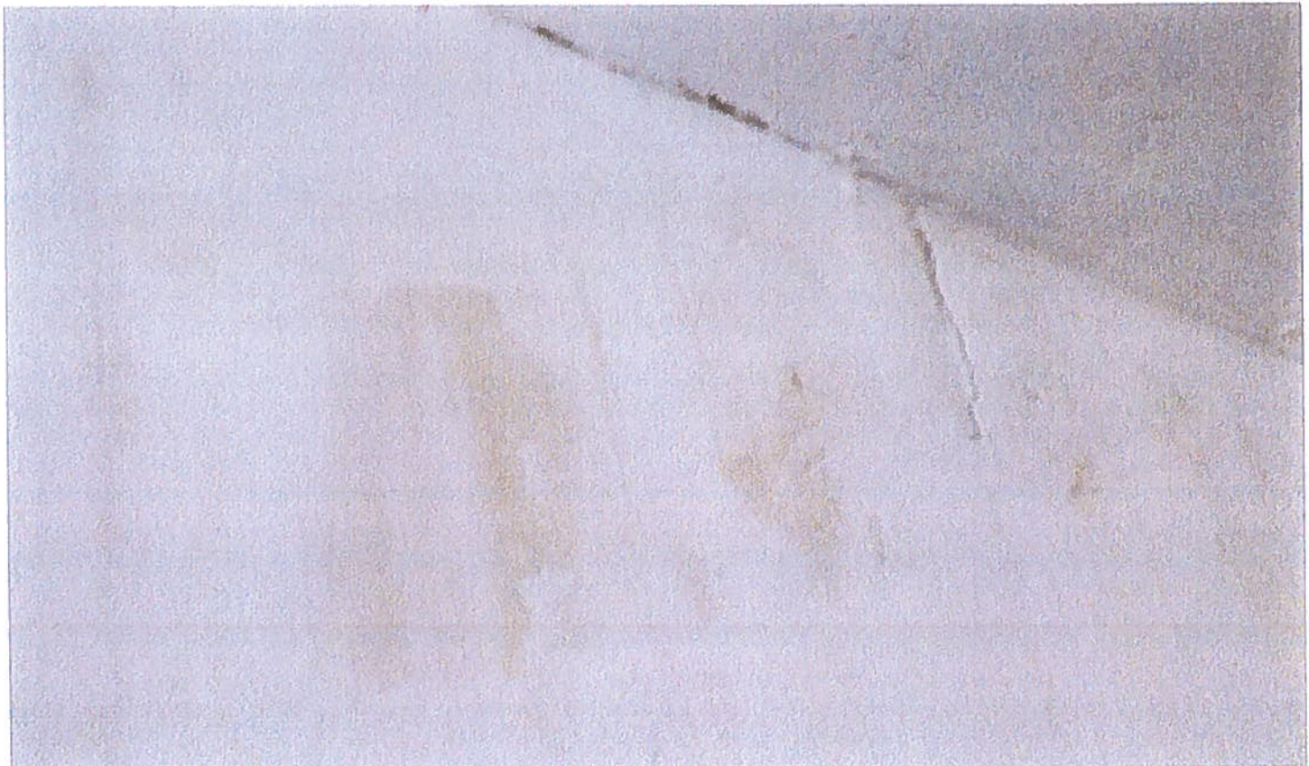
Photo 2: Apparent moisture staining on the perimeter wall of the stairwell.
