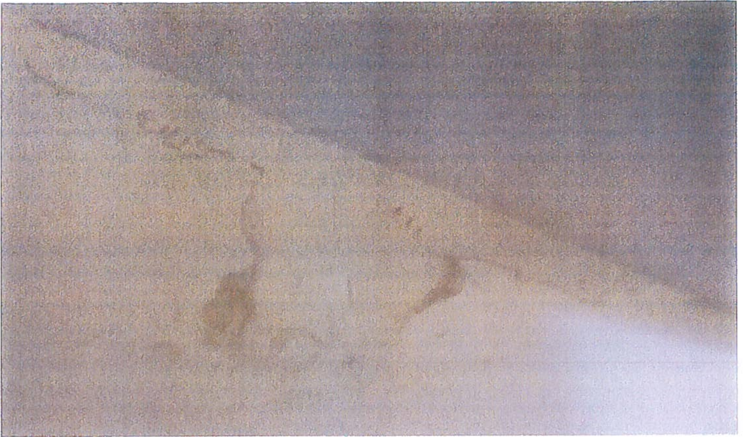
Photo 5: Apparent moisture staining on the perimeter wall of the stairwell.
