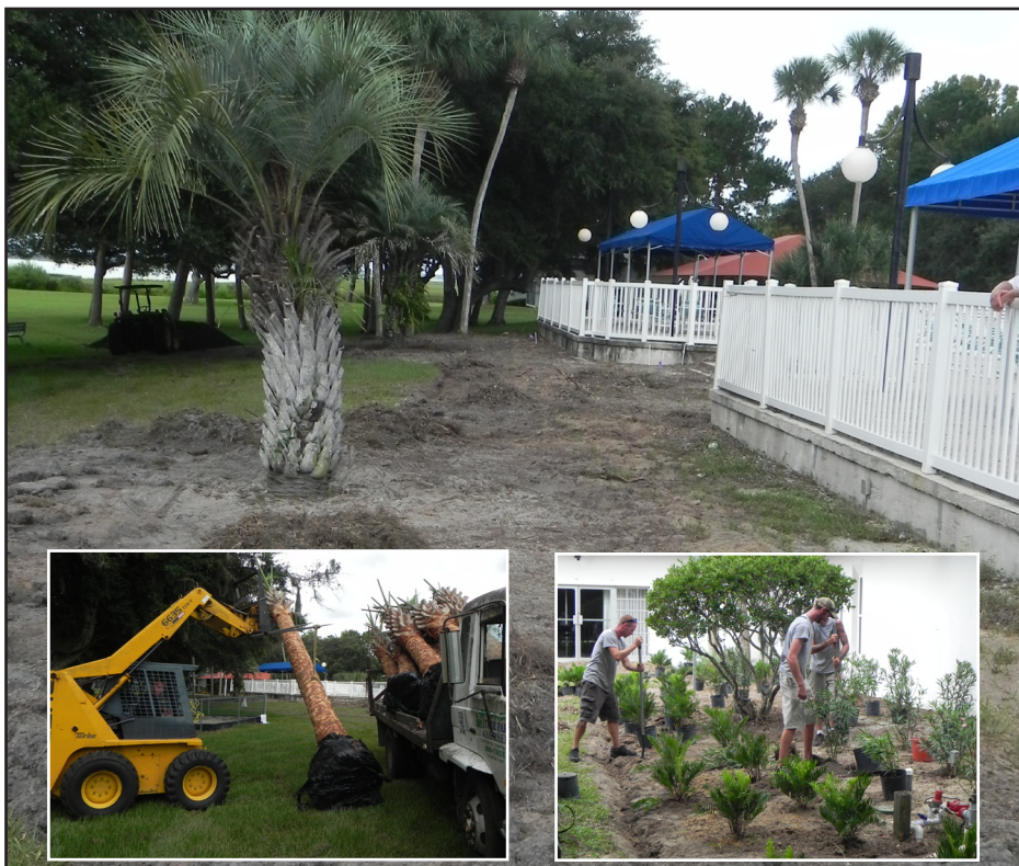
Landscaping work has begun on the Riverview Clubhouse grounds. Pictured are workers preparing the ground, planting shrubs and unloading palm trees.
