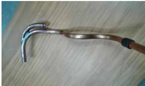
Revised pipe to ensure heater works →
