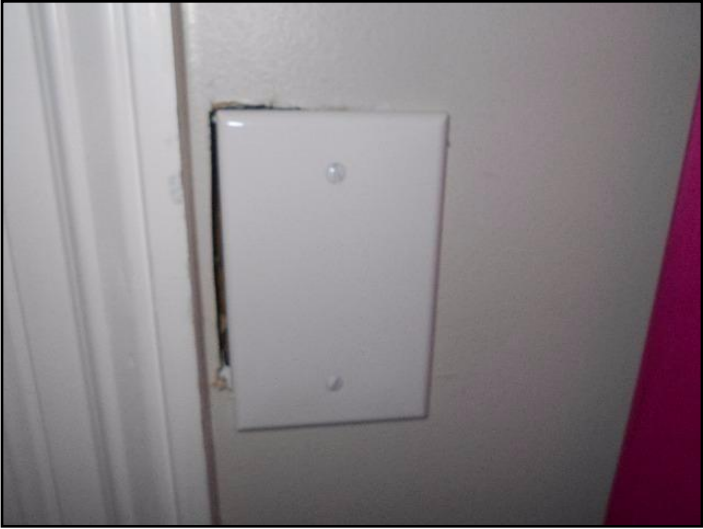
2. GFCI/GFI needed (Ground Fault Circuit...
