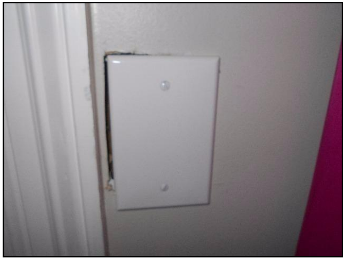
8. GFCI/GFI needed (Ground Fault Circuit...
