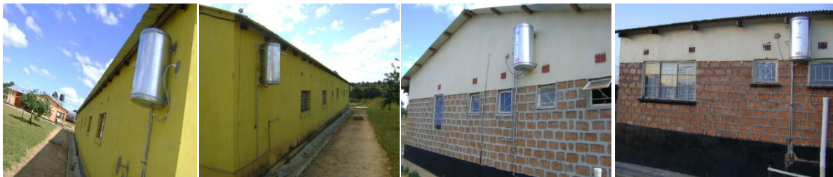
Hot water geysers fixed to four dormitories
