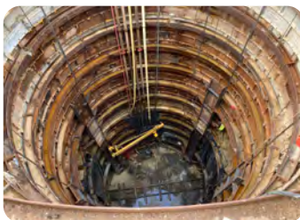
SAWS W-6 Upper Segment C, TX
