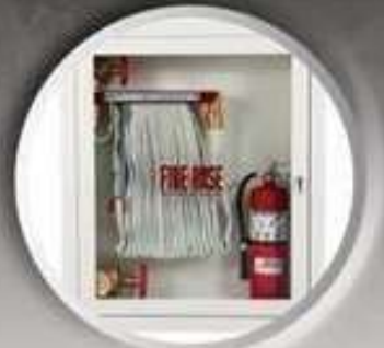
FIRE DEPARTMENT VALVE, FIRE EXTINGUISHER & FIRE HOSE CABINETS AND REELS
