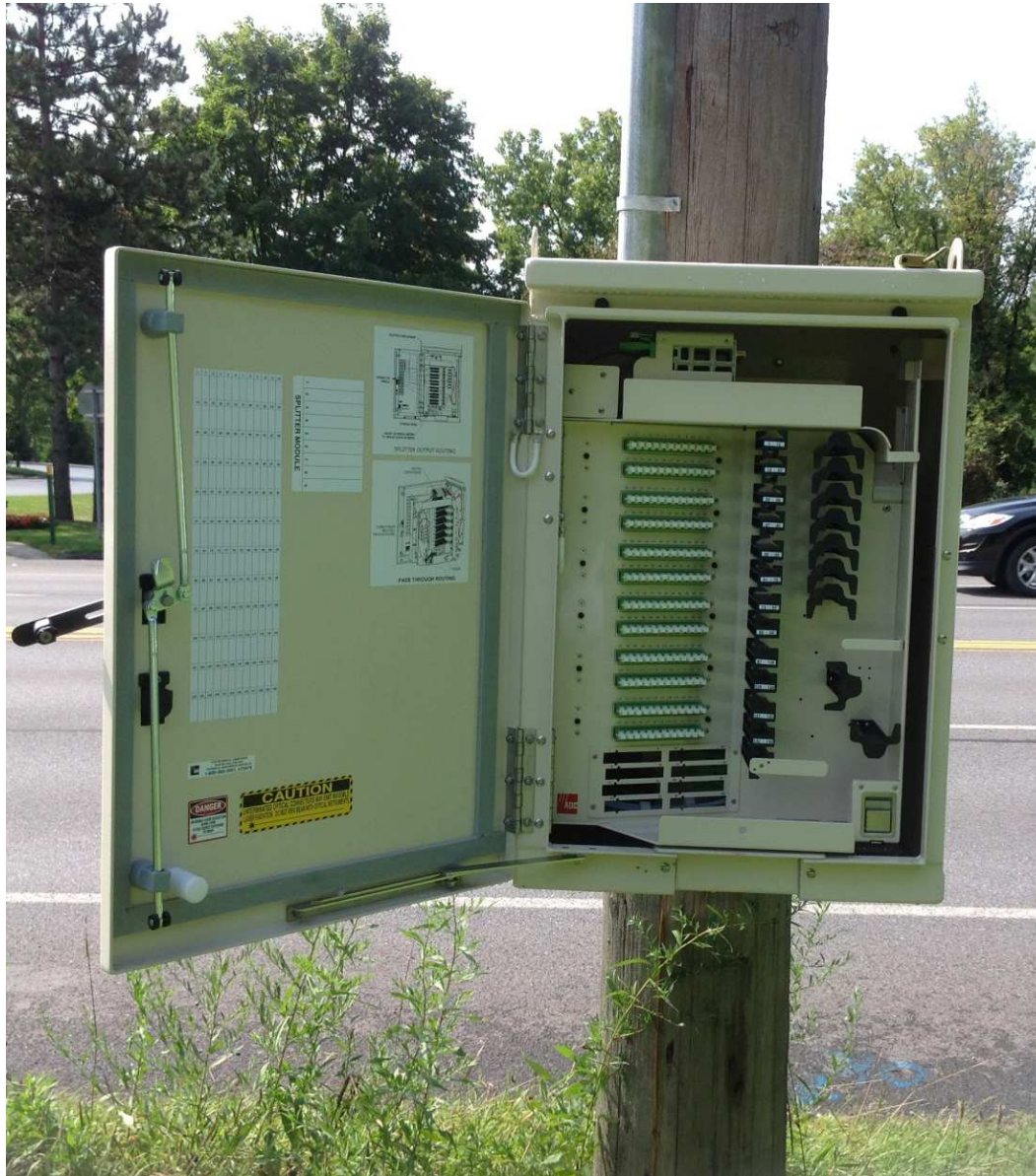
FDC 144 Fiber Cabinet Pole Mounted
