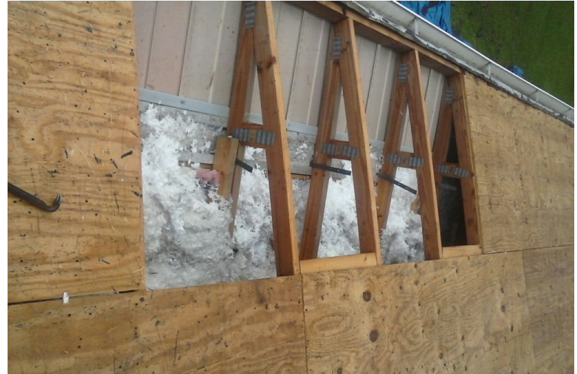
Hurricane Straps on the Trusses
