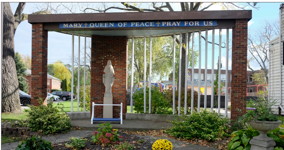
The shrine as it is now, in need of repair. (Notice the missing vertical struts.)
