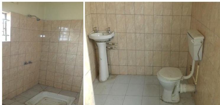
Showers and toilets in guest rooms
