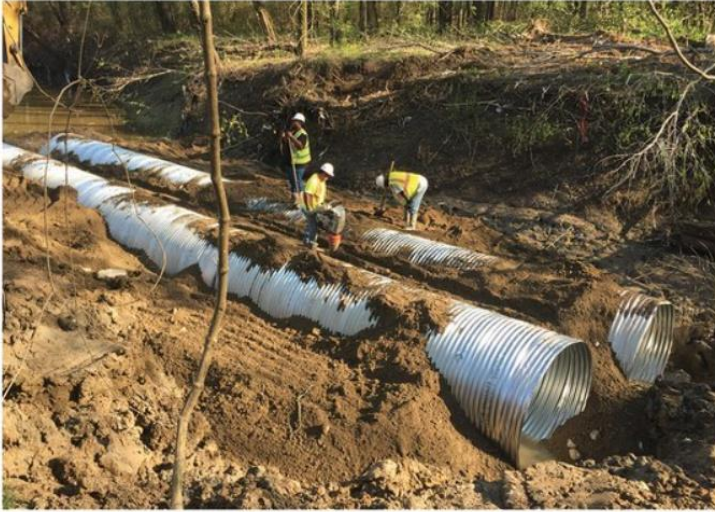
A culvert was put in place along 100 feet of the bypass line where the bypass crossed Cypress Creek.
