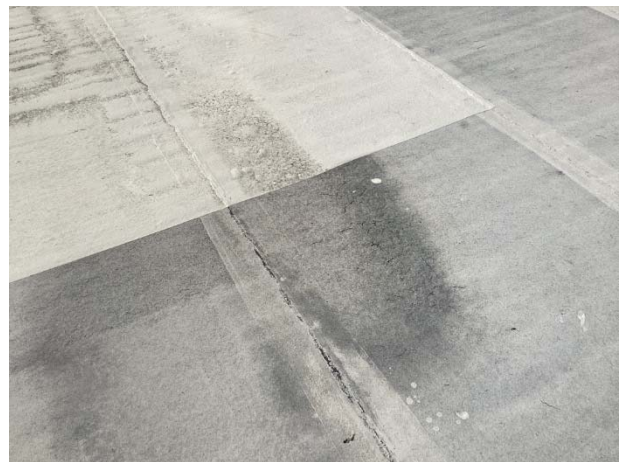
Cracks, bulges and previous repairs
