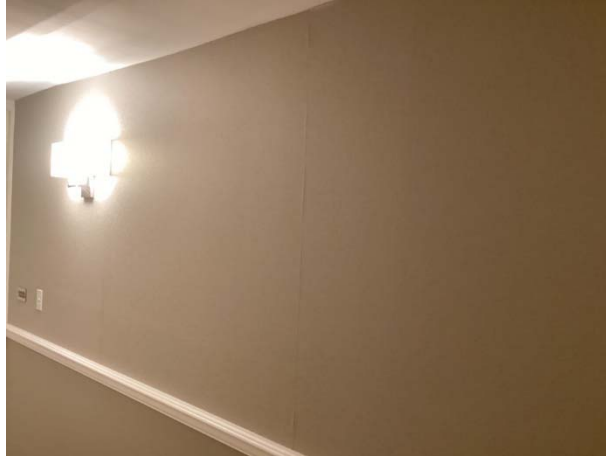
Peeling seem at floor 12
