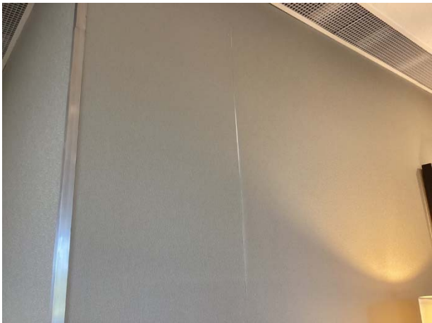
Wall covering separation at lobby
