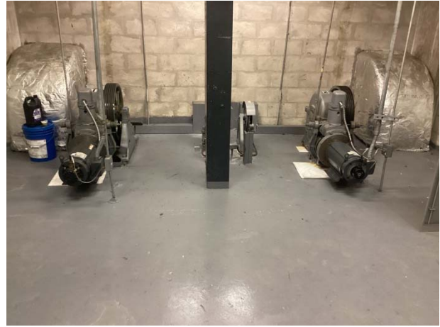
Traction elevator hoists and motors
