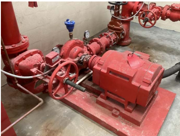
Fire suppression pump
