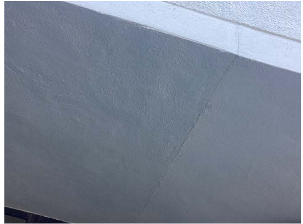
Stucco crack with minor rust stain below second floor balcony
