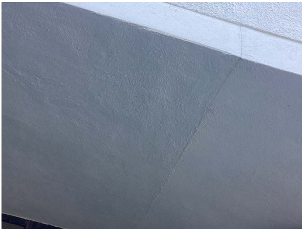
Crack with rust stain below second floor balcony
