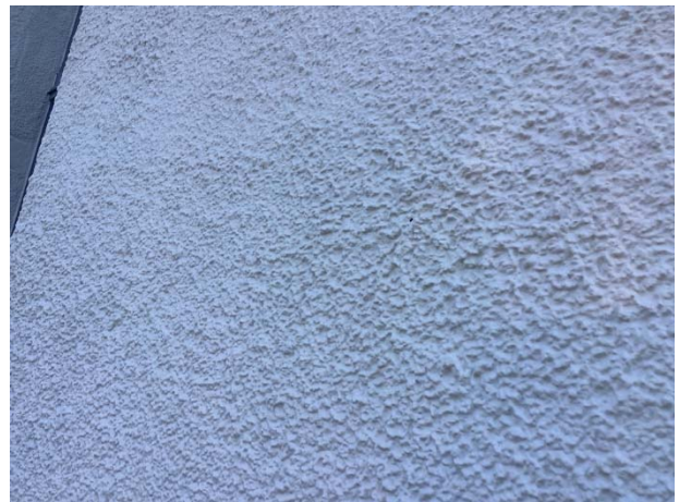
Small hole in stucco
