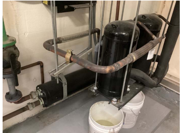
Split system condensing unit
