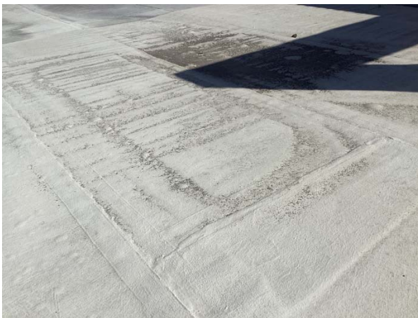
Bulges in coating
