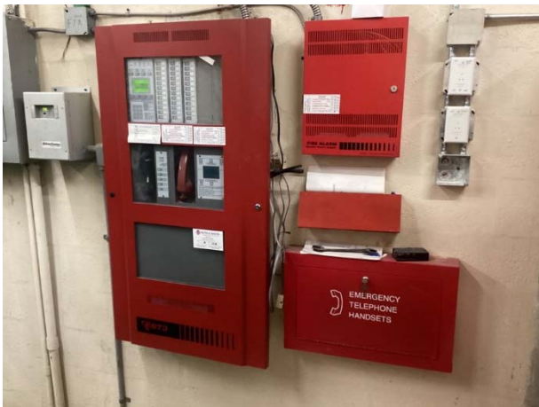
Control panel and voice communication system
