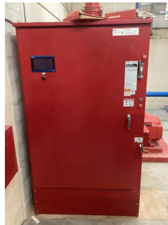
Fire suppression pump controls
