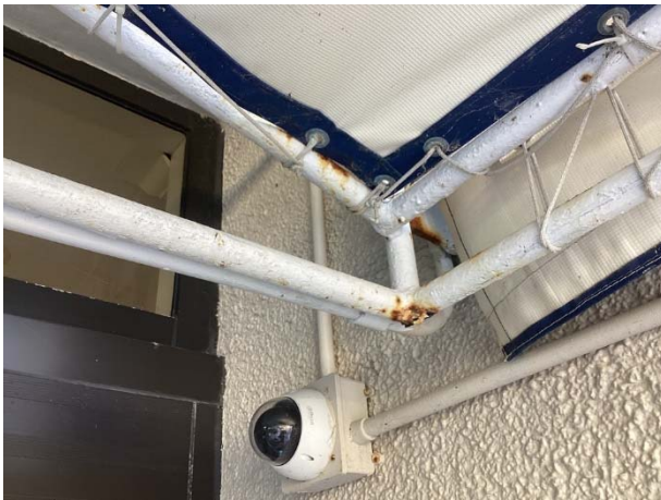
Frame rust at entrance awning
