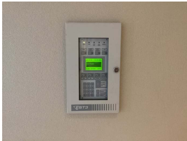
Secondary panel at lobby
