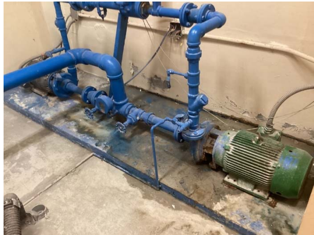
Domestic water pumps
