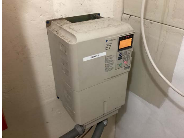
Domestic water pump control
