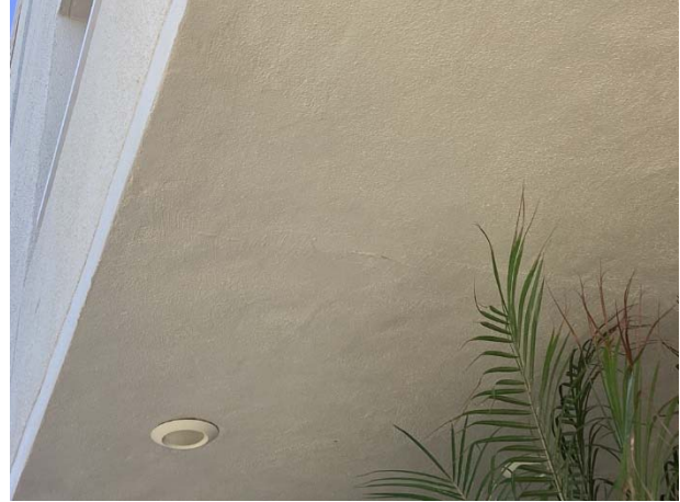
Previous repair under second floor balcony
