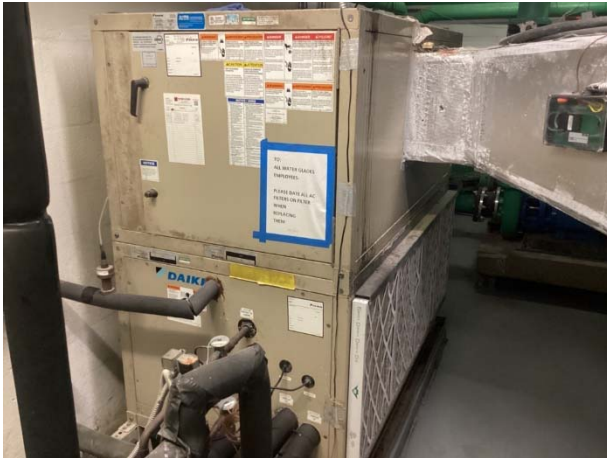
Split system air handling unit
