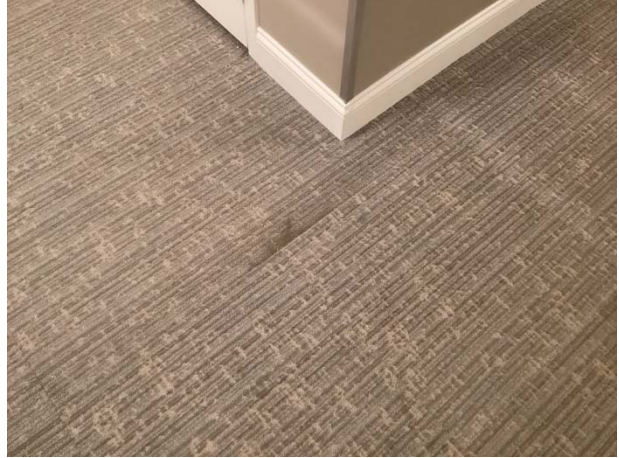
Carpet stain at floor 12
