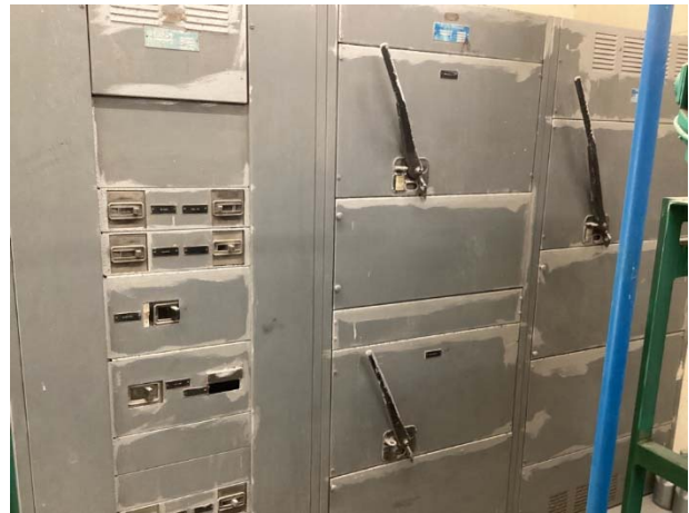
Electrical system main panels on first floor
