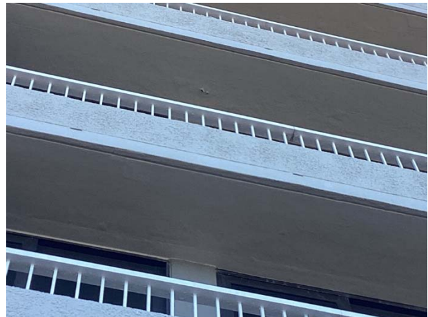
Signs of water intrusion under balconies at floors four and five
