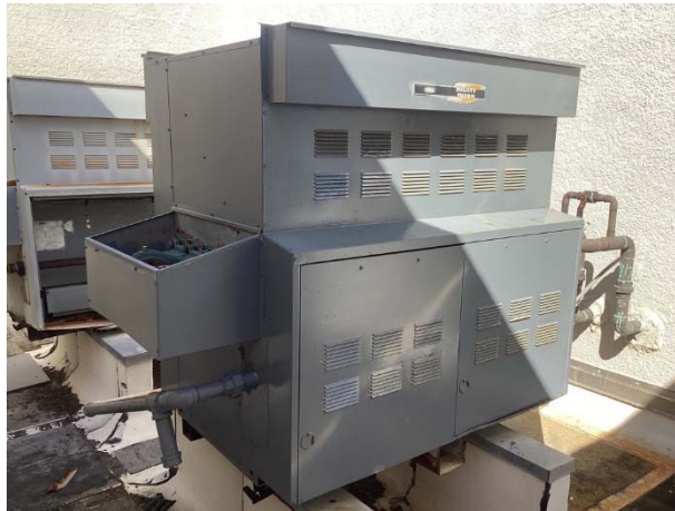
Building heat boiler
