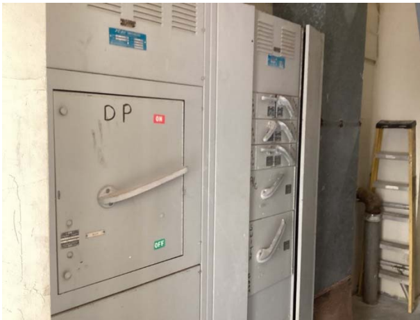
Electrical system main panels on roof
