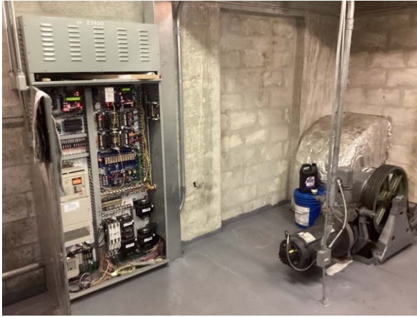
Traction elevator equipment
