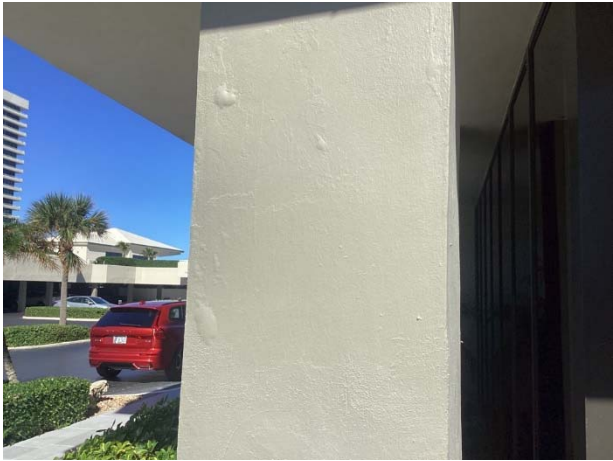
Paint bulges at first floor column
