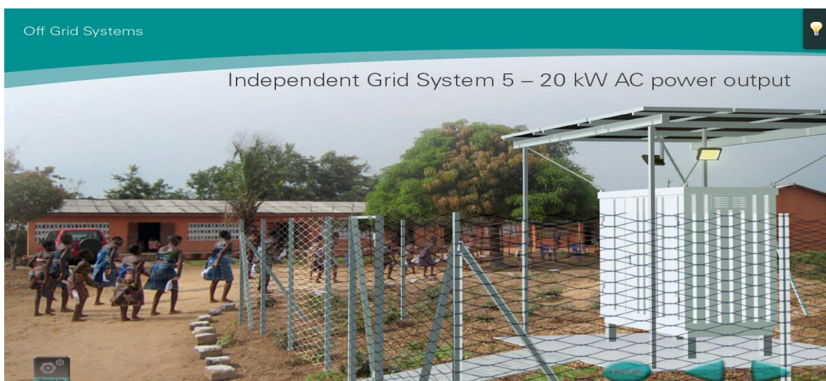
Figure 4.3 Community – School Electrification project in Tanzania - executed by Kirchner Solar Germany – Partners of Suchnetcom Solar
