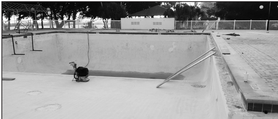
The Shores Riverview club Pool Remarcite project is underway and is planned to be completed by the end of January.
