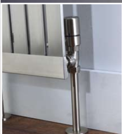
Valves are positioned behind the radiator.
