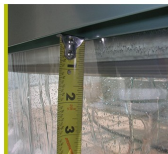
Spacer bar displacement into glazing unit obstructing view
