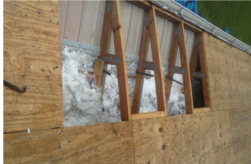
Hurricane Straps on the Trusses
