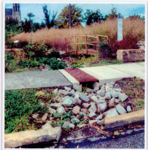
Bioswales (above) are a structural BMP that can help mitigate the effects of stormwater once a site has been developed.
