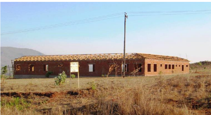
The building as it looks with the trusses...ready for a roof, windows and doors.
