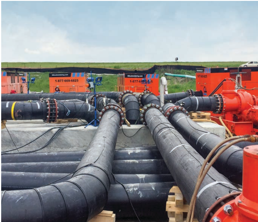
BELOW: HDPE pipes running from the Godwin Dri-Prime pumps to the splitting chamber for Phase III of the bypass. FIRST PAGE: A short distance from the taxiway, pumps and piping were placed by crane at the job site.
