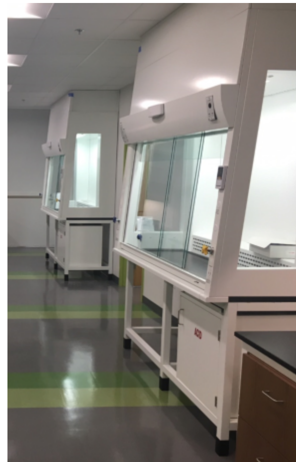
Chemical Fume Hood
