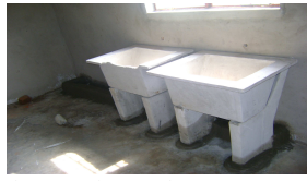
wash troughs to dry & cemented out
