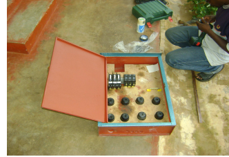
3 phase distribution meter box
