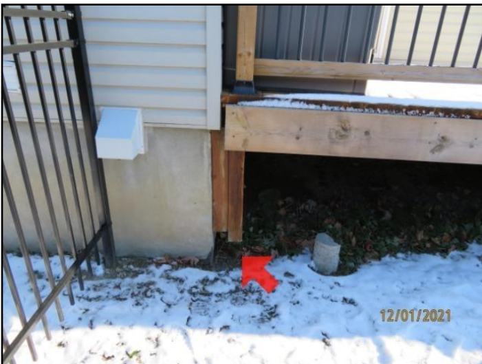
10. not secured at bottom
