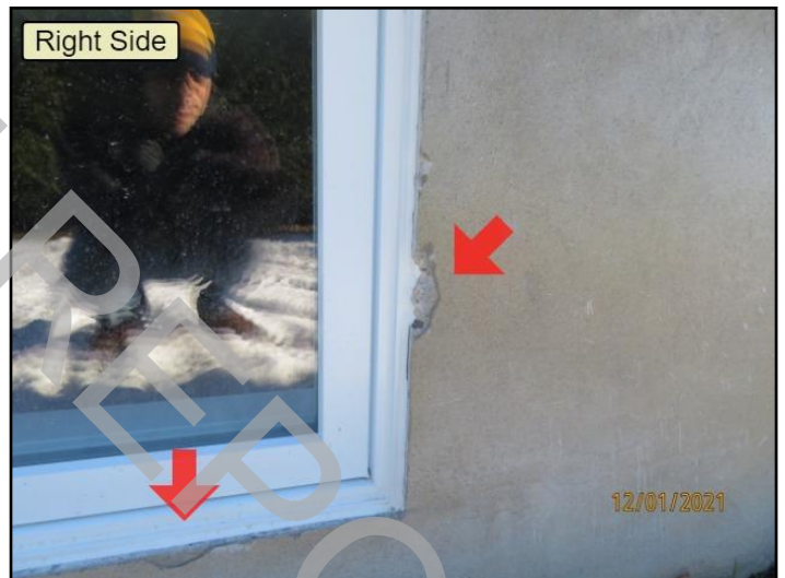
32. Parging damaged or missing
