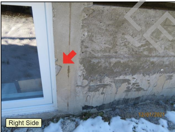
31. Parging damaged or missing
