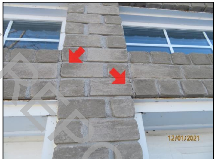
40. Typical minor cracks
