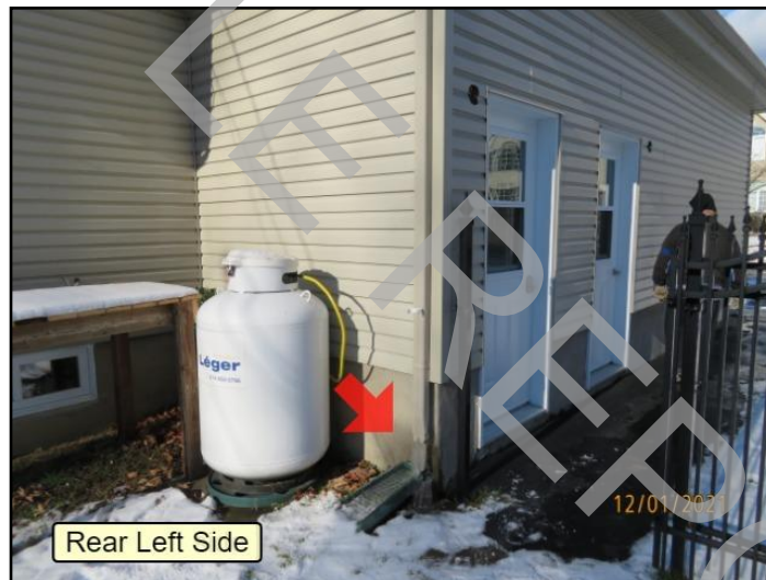
6. Discharge too close to building
