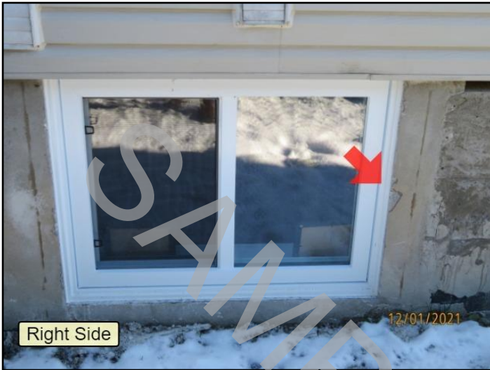
29. Parging damaged or missing
