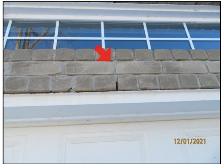
38. Typical minor cracks
