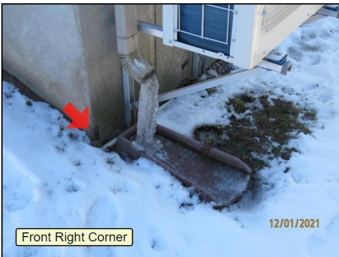
27. Plarging damaged or missing
