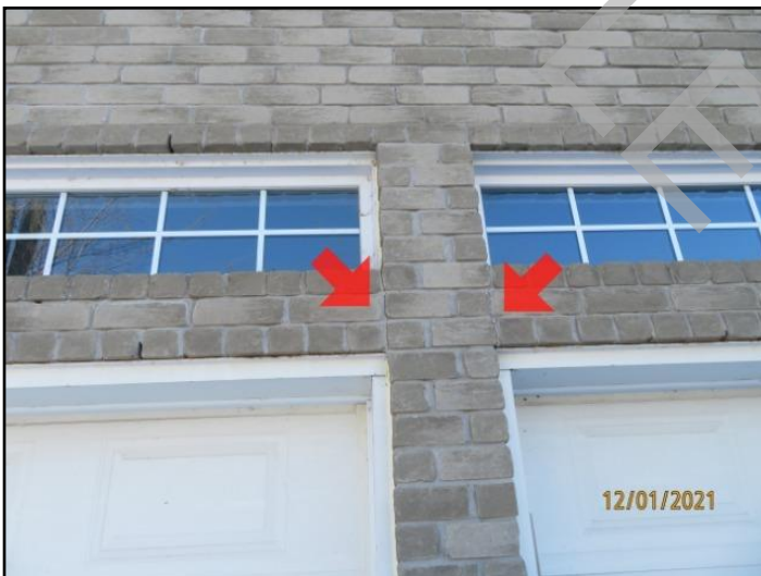
39. Typical minor cracks
