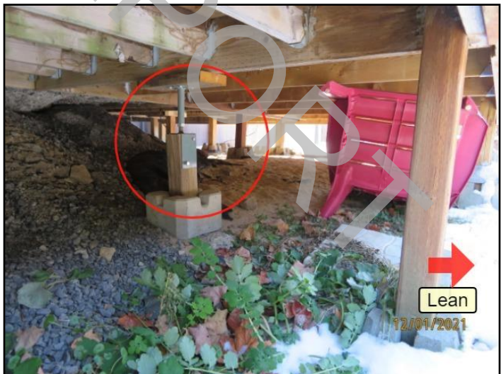
11. Poorly secured at top & bottom:At the...
