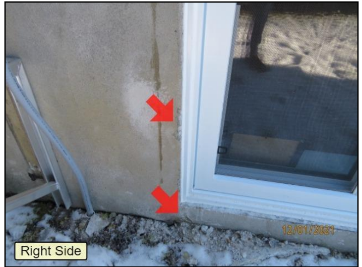
30. Parging damaged or missing
