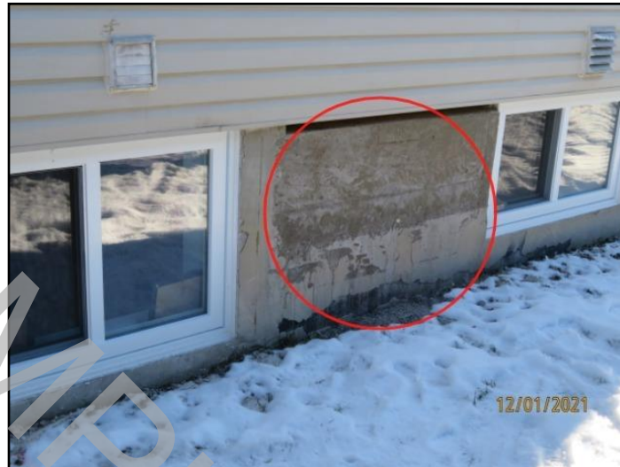
26. Plarging missing- prior repair
