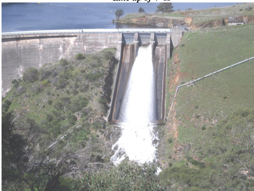
Water flowing well in the Reservoir
