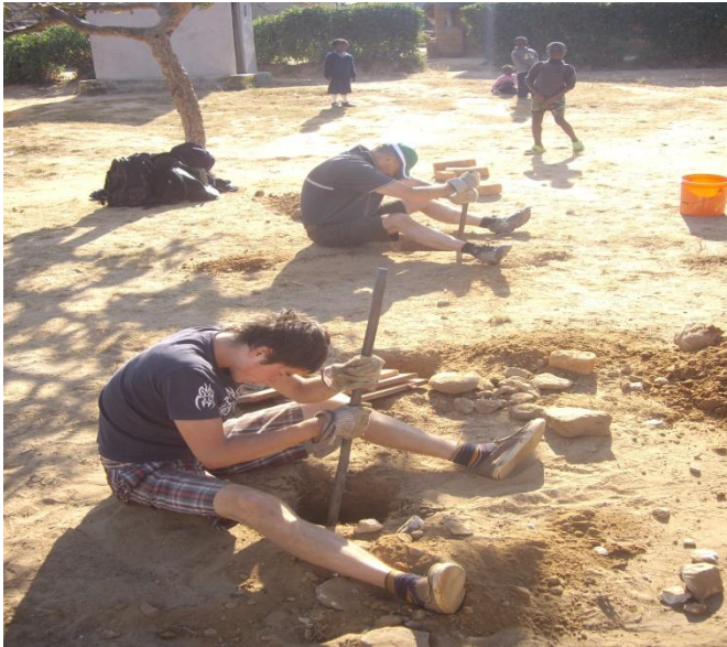
Digging in and cementing the posts for the climbing wall was tough work
