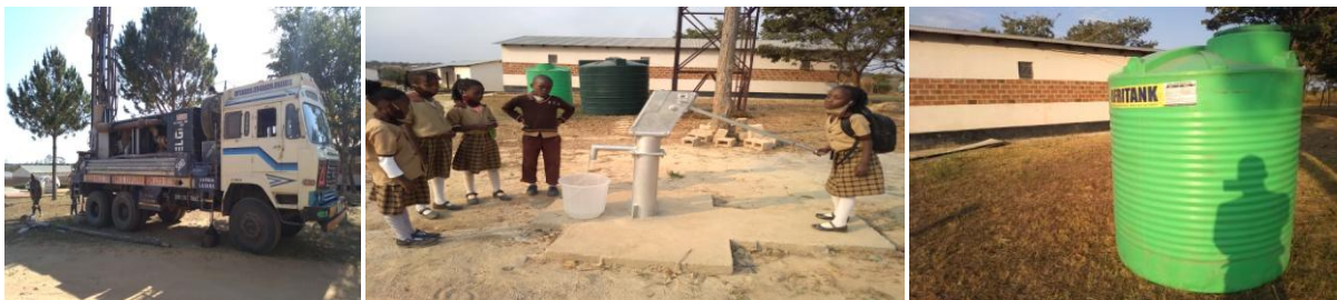
Borehole was drilled and hand pump was installed due to insufficient ground water
