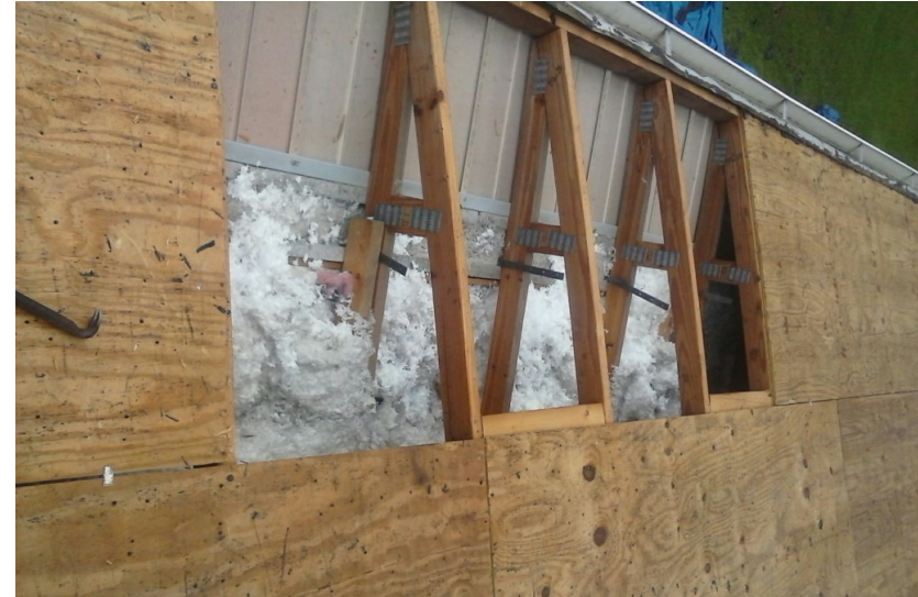
Hurricane Straps on the Trusses
