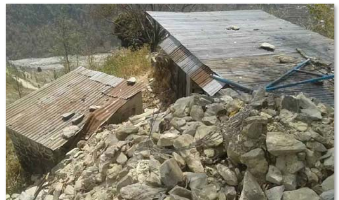
Suryodaya School after the earthquake
