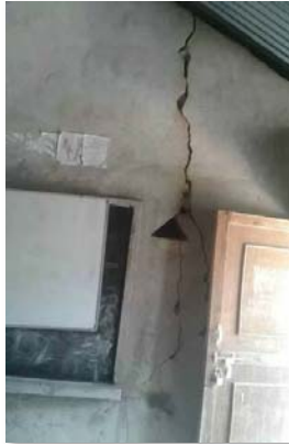
Classrooms are unsafe
