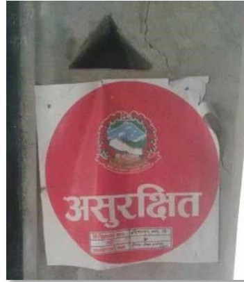
An “UNSAFE” sticker placed by the government
