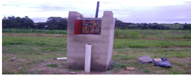
3 phase distribution point done by SOSH
