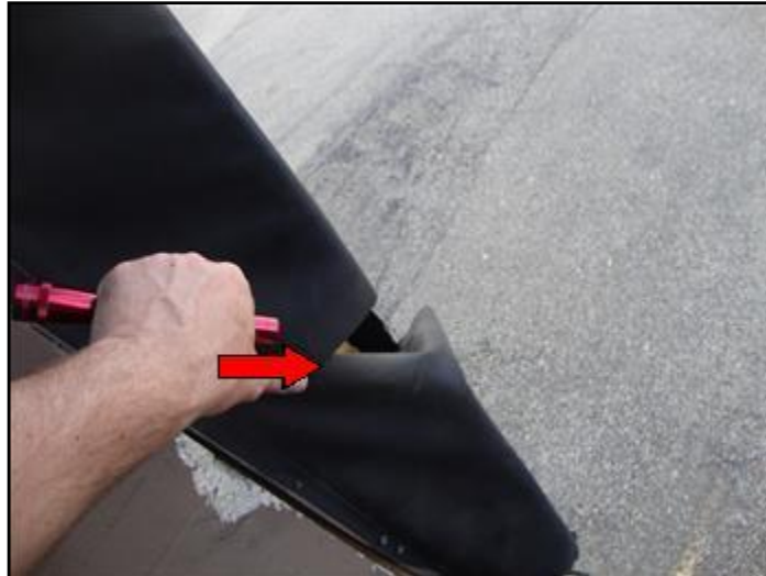
Replace damaged / missing cushions
