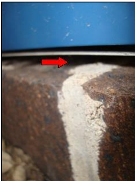
Some settling has occurred, as can be...
