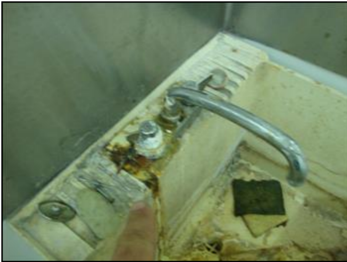
The leaking faucet requires repair
