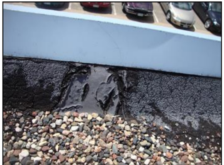
Damaged membrane due to sunlight exposure...
