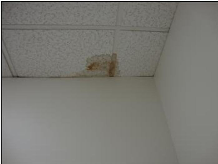
A water stain was noted
