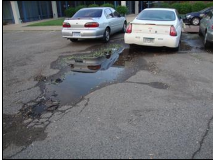
Potholes are noted
