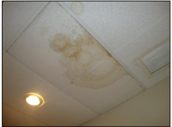
A water stain was noted
