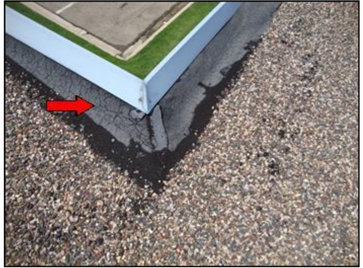
Damaged membrane on the curb mount
