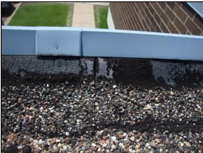
Damaged membrane due to sunlight exposure...
