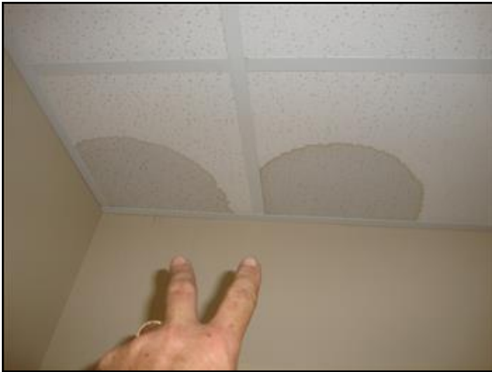
A water stain was noted
