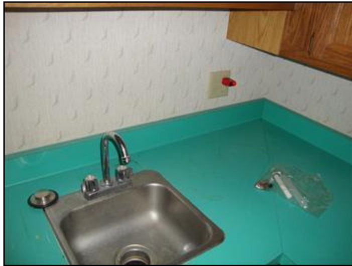
Electrical outlets in close proximity to a...
