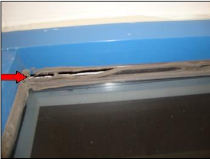
Some settling has occurred, as can be...
