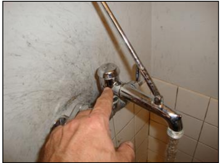
The leaking faucet requires repair
