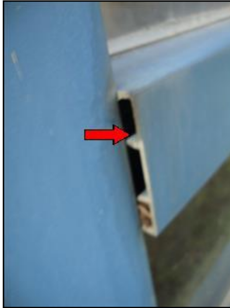
Some settling has occurred, as can be...
