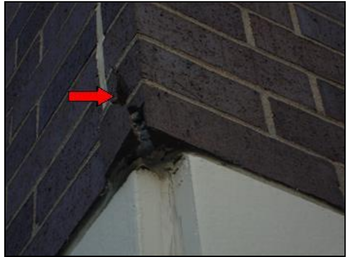
Some settling has occurred, as can be...
