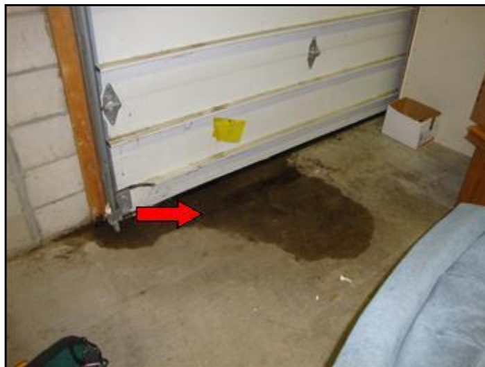
A water stain was noted
