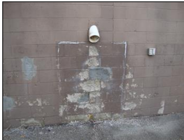
Water damage was noted
