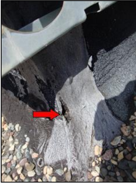
Damaged membrane on the curb mount
