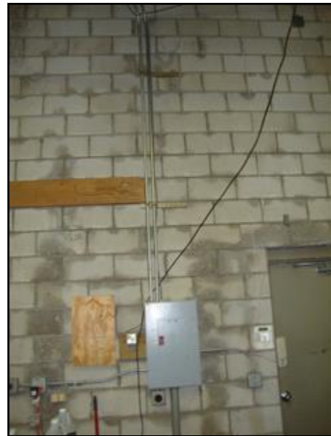
A water stain was noted
