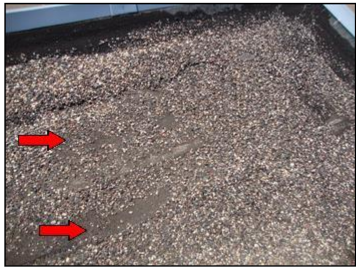
Missing gravel exposes the membrane to...
