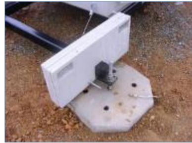
Plates Fastened Together But Not to the Frame
