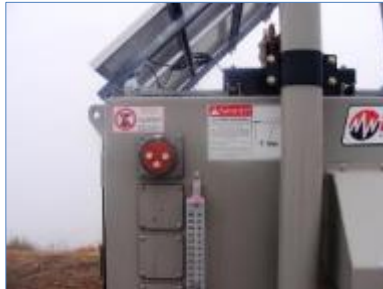
Tower Ground Bus Bar Installed Near RF Cable Entrance
