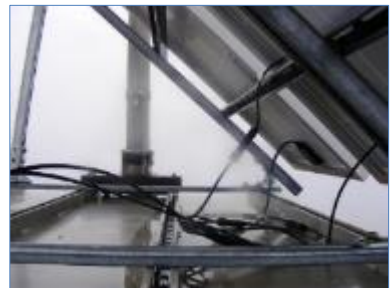
Solar Panels and Framework Not Grounded
