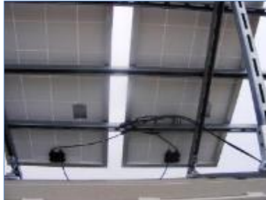
Solar Panel Wiring Not Properly Fastened to Framework
