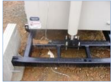
Tower Ground Bus Bar Grounded to Ground Ring
