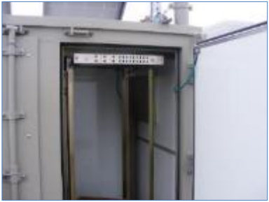
Door Grounded to Cabinet Unibody Structure
