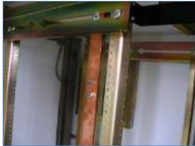
Rack Ground Bus Bar #1
