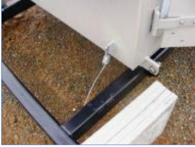
Pass-Through Bar Grounded to Ground Ring
