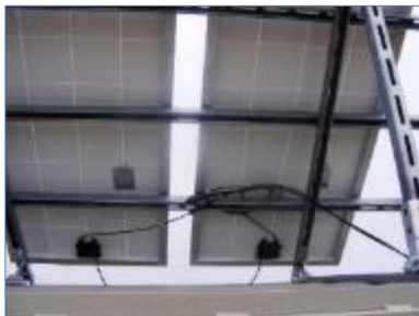
Two Solar Panels Not Grounded
