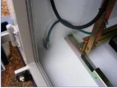
Rack Ground Bus Bar #2 Grounded to Pass-Through Bar
