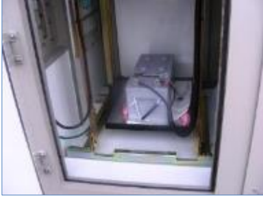
Battery Installed and Connected to Solar Charger/Controller
