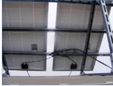
DC Wiring Not Adequately Fastened to Framework
