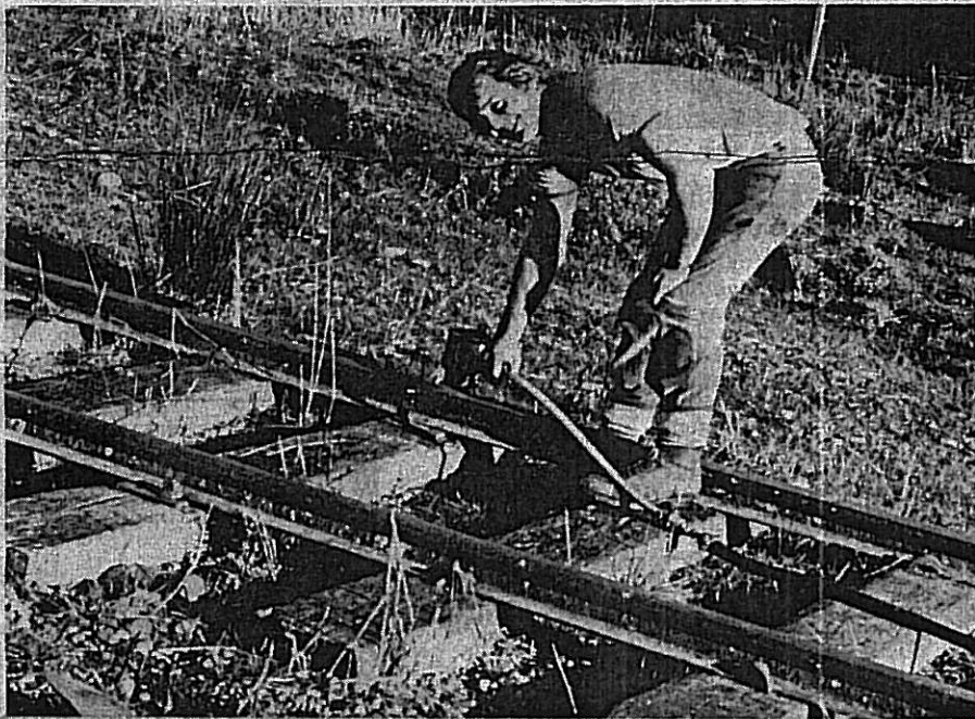
GRAHAM HOLGATE using a compressor to remove bolts from the railway track near Conical Hill. He is one of the workers employed by Timaru contractor Mr Pat Heffernan taking up the Heriot-Waipahi railway line.
