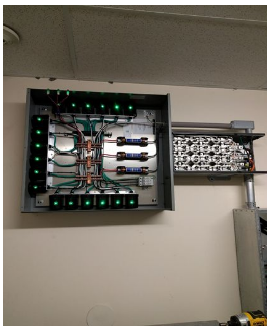
480 Volt / 100 KVAR unit opened to expose the heart of the unit, the metal oxide Varistors shown above
