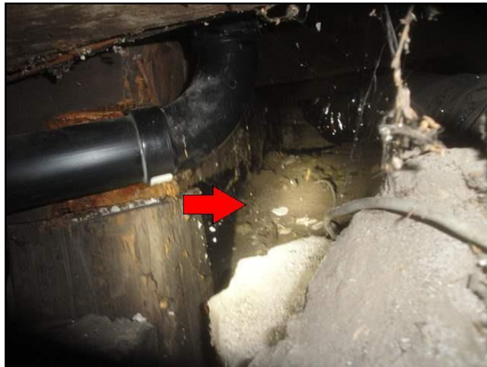
72. No vapor barrier
