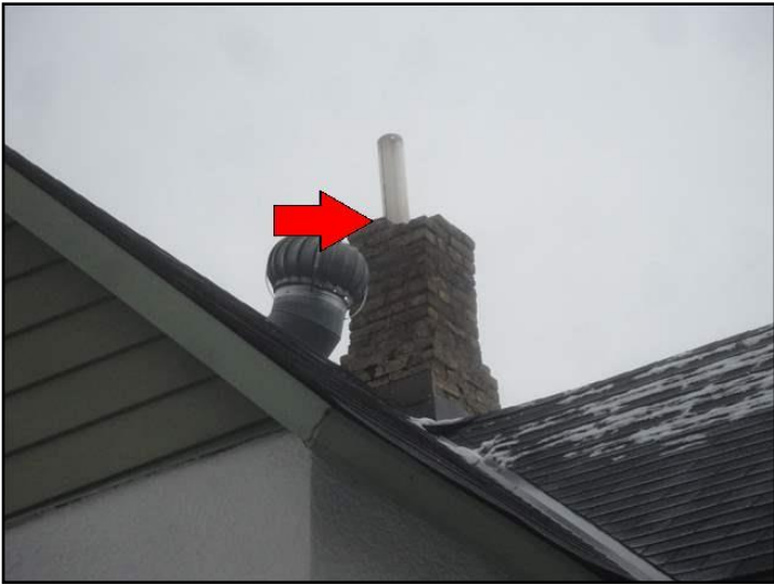
71. Loose, missing or deteriorated mortar
