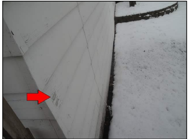
15. Paint or stain - needed
