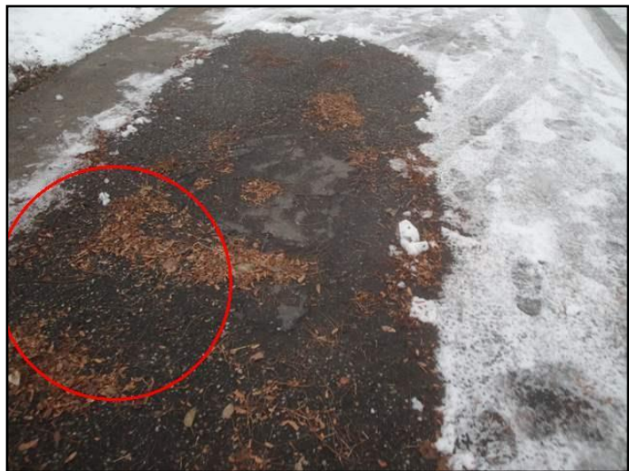
30. Cracked or damaged surfaces
