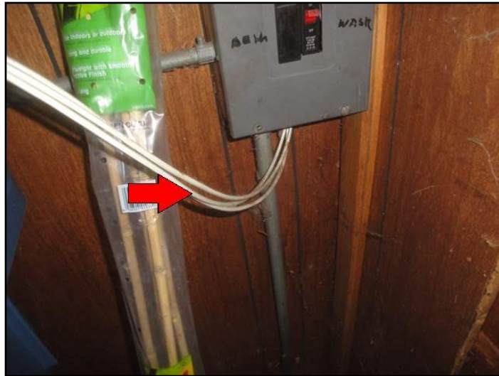
62. Flexible conduit needed
