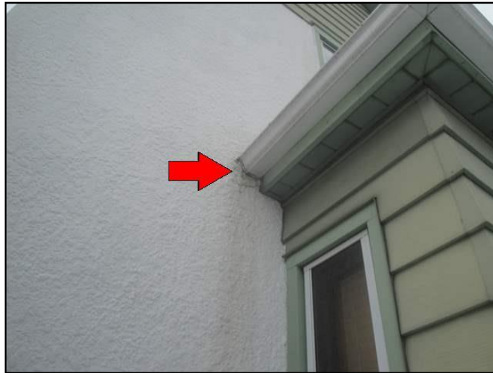
4. No kickout flashing
