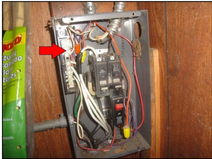
53. Neutral bonded to ground downstream of box
