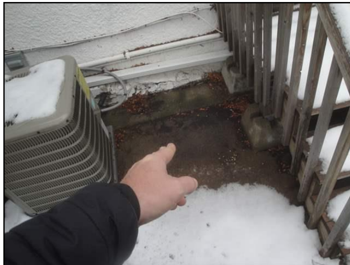
33. Improper slope or drainage
