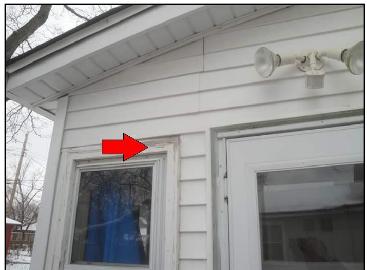
7. Paint or stain needed
