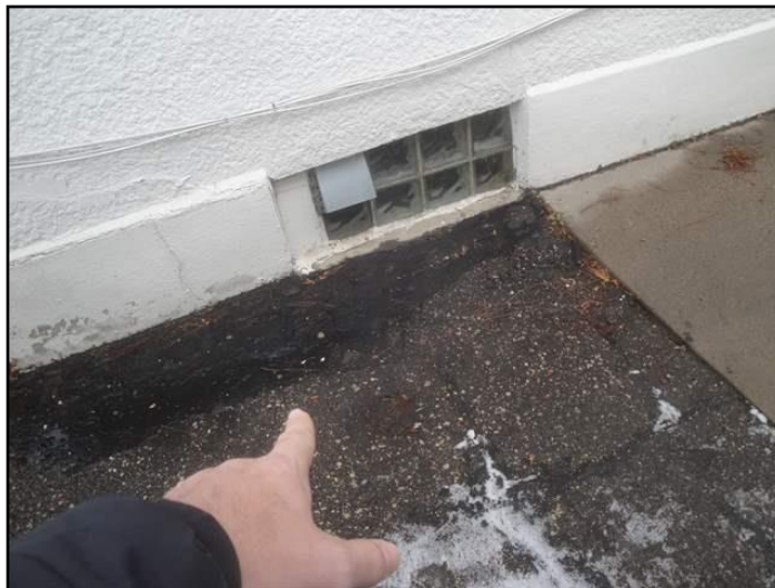
31. Improper slope or drainage
