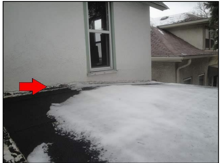
9. Caulking missing or ineffective
