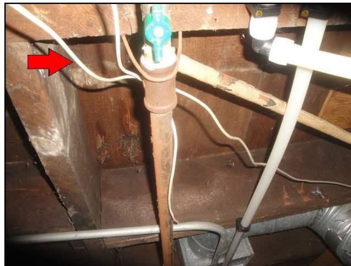
61. Not well secured
