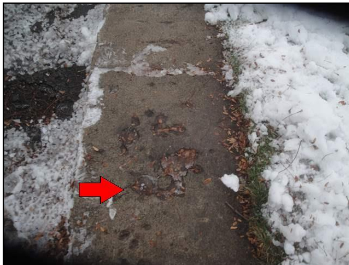
32. Cracked or damaged surfaces
