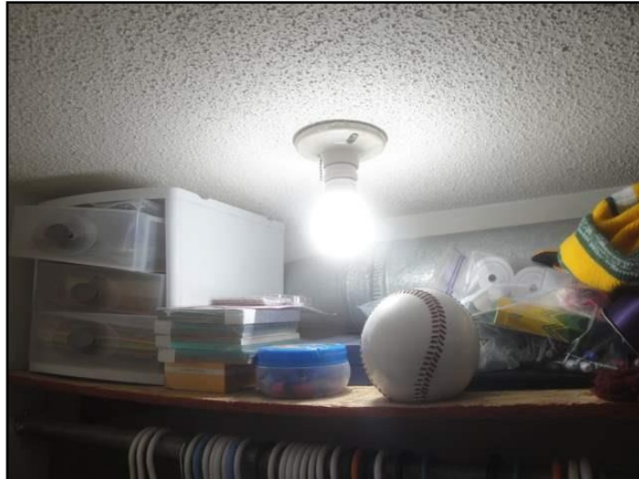
63. Improper closet lighting
