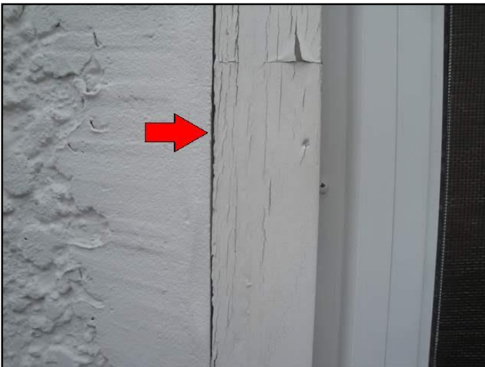
10. Caulking missing or ineffective
