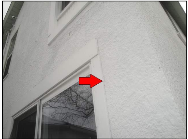
13. Caulking missing or ineffective
