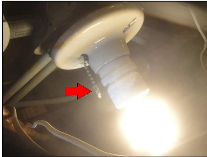
64. Isolating links needed on pull chains
