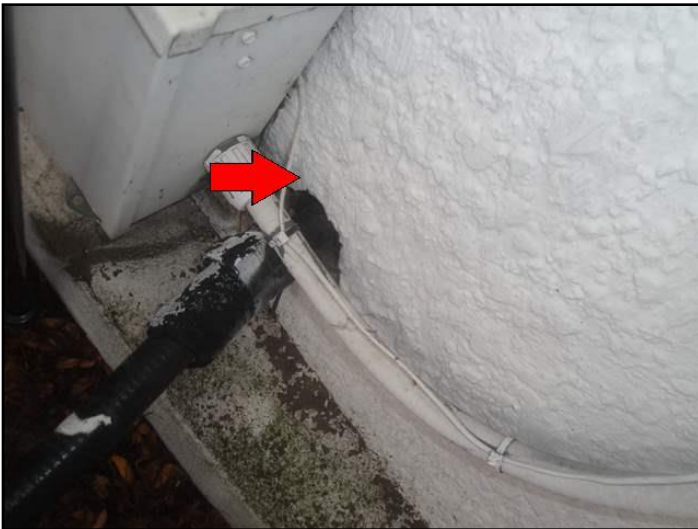
8. Caulking missing or ineffective
