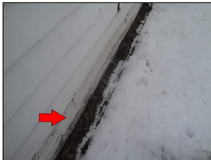
16. Too close to grade
