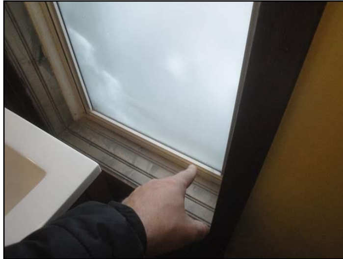
79. Safety glass not installed
