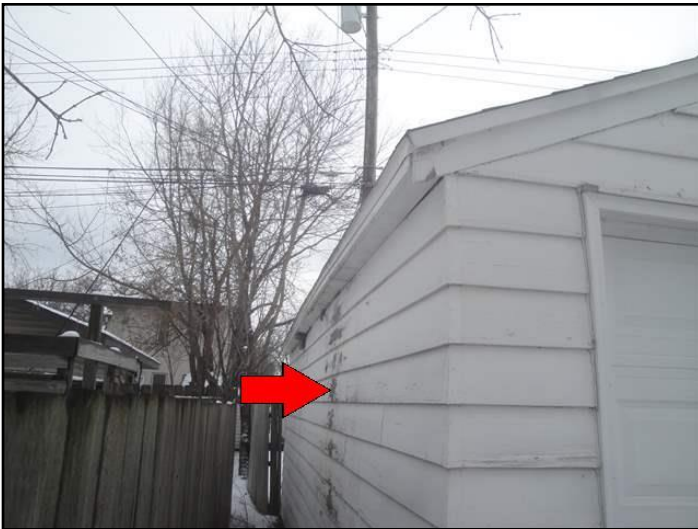
14. Paint or stain - needed
