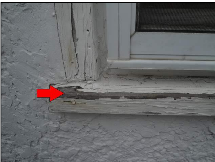
6. Paint or stain needed
