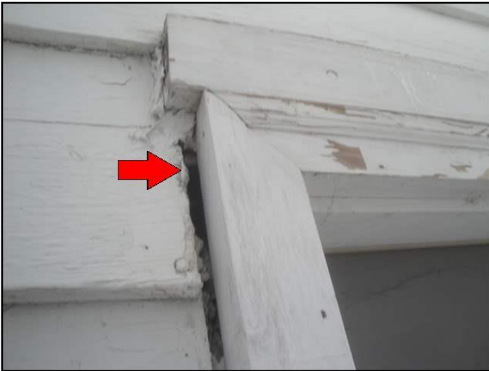
12. Caulking missing or ineffective
