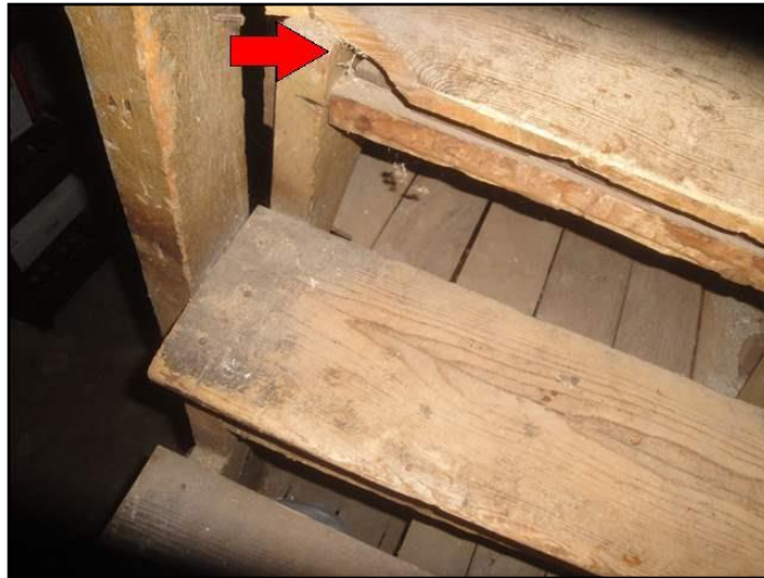
86. Worn or damaged
