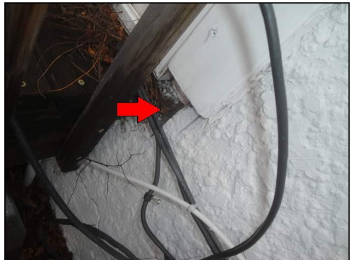
11. Caulking missing or ineffective
