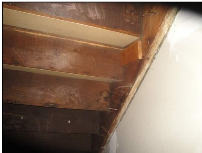
85. Drywall missing or incomplete on underside...
