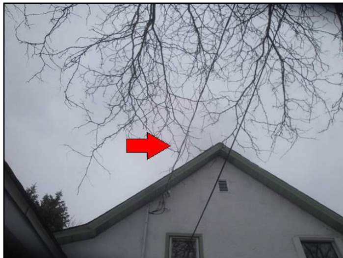
52. Branches, vines interfering with wires
