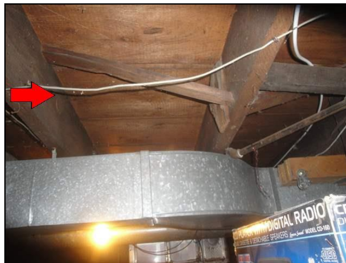
49. Ineffective blocking, bracing or bridging
