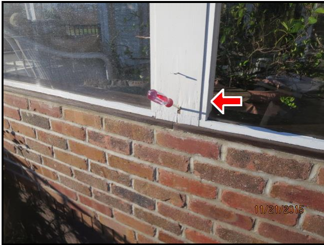
2.0 Item 1(Picture) Wood Rot
