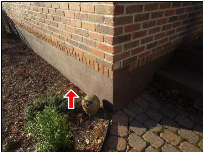
6.0 Item 3(Picture) Wall cracks
