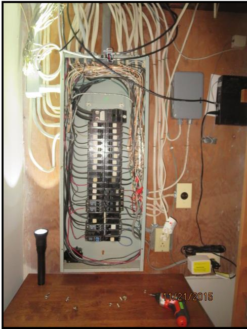
3.6 Item 1(Picture) Main Panel Box
