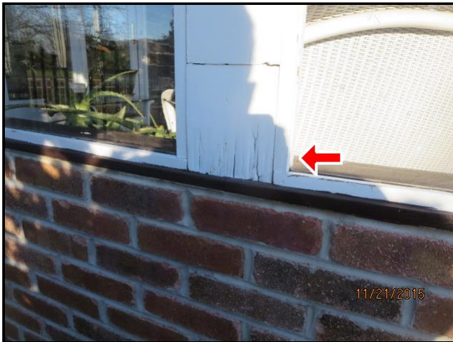
2.0 Item 3(Picture) Wood Rot
