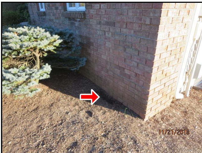
2.0 Item 4(Picture) Missing or buried weep holes
