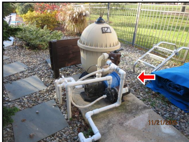
11.0 Item 1(Picture) Pump & Filter
