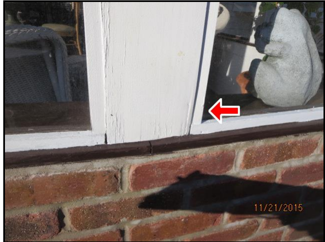
2.0 Item 2(Picture) Wood Rot
