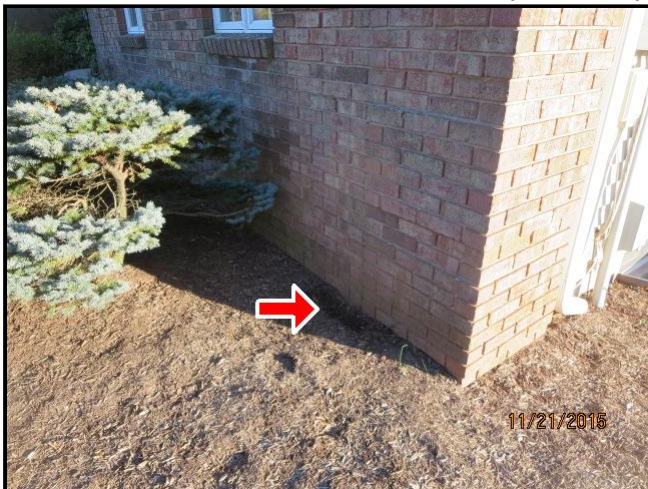
2.0 Item 4(Picture) Missing or buried weep holes
