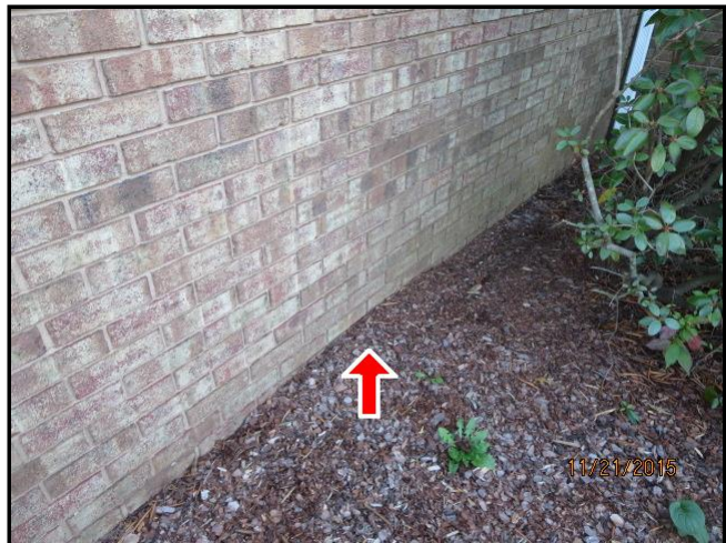
2.0 Item 5(Picture) Missing or buried weep holes
