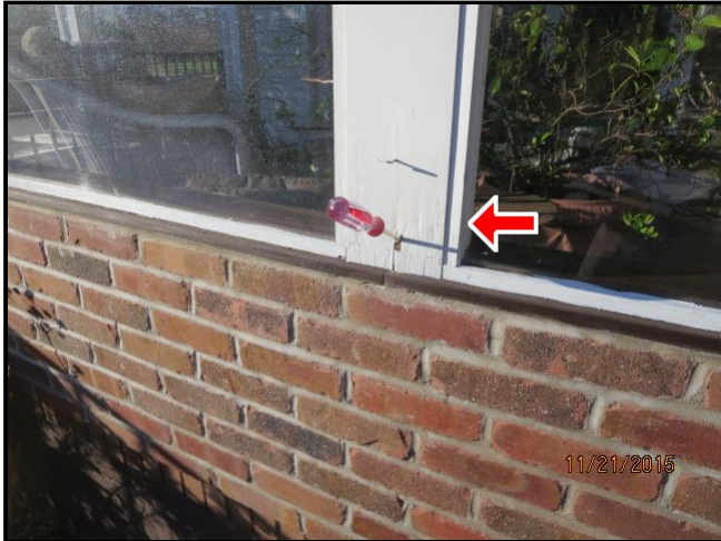
2.0 Item 1(Picture) Wood Rot
