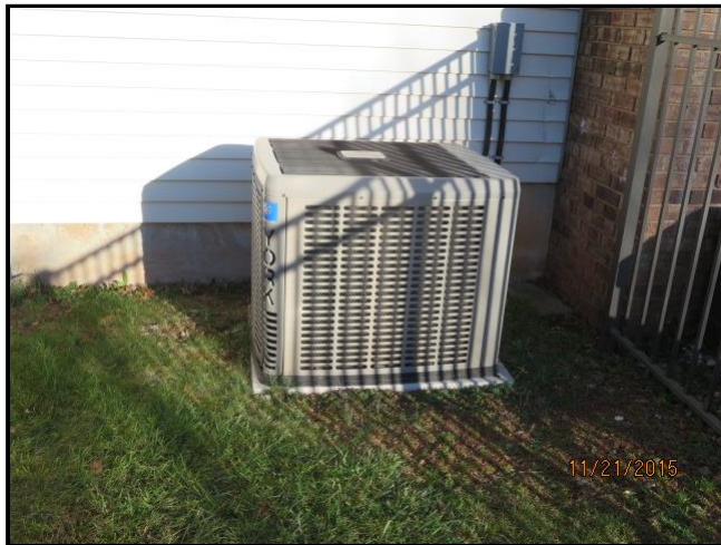
4.8 Item 1(Picture) 2005 condenser
