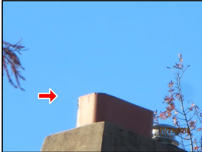
4.5 Item 1(Picture) Missing Rain Cap
