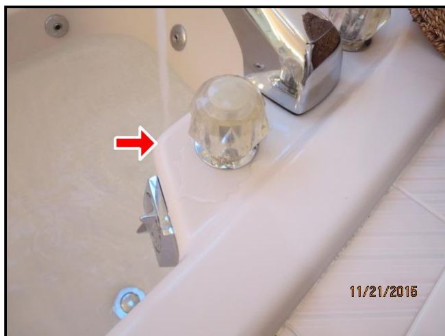
5.1 Item 4(Picture) Valve leak
