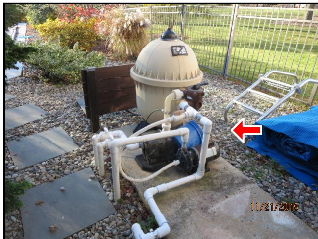
11.0 Item 1(Picture) Pump & Filter
