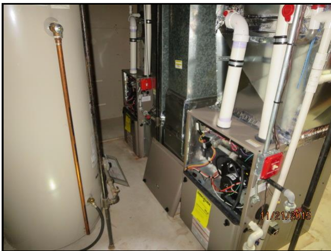
4.0 Item 1(Picture) Furnaces
