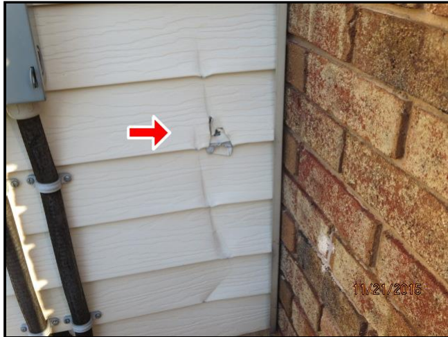
2.0 Item 6(Picture) Damaged siding
