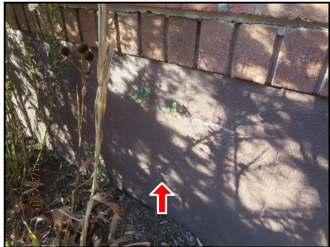
6.0 Item 4(Picture) Wall cracks
