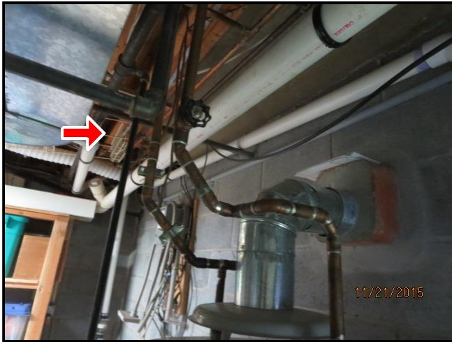
5.2 Item 1(Picture) Missing bond wire
