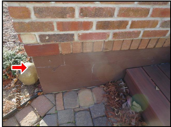
6.0 Item 2(Picture) Wall cracks
