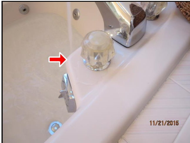
5.1 Item 4(Picture) Valve leak
