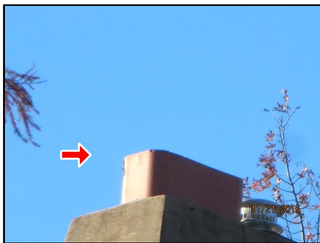
4.5 Item 1(Picture) Missing Rain Cap
