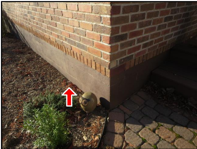
6.0 Item 3(Picture) Wall cracks
