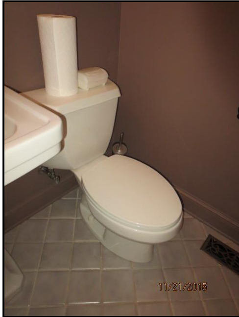
5.1 Item 3(Picture) Loose toilet
