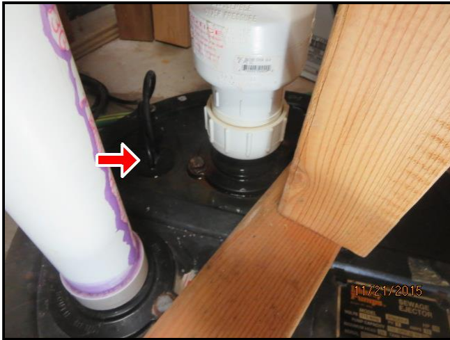
5.1 Item 1(Picture) Pump up system leak
