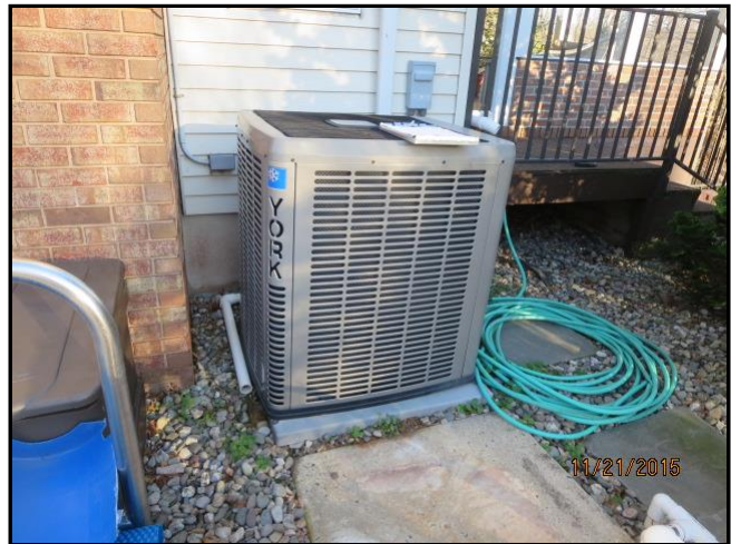
4.8 Item 2(Picture) 2008 Condenser
