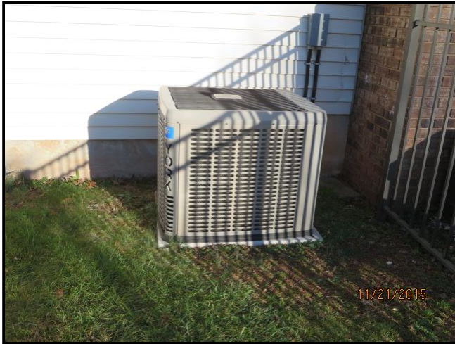
4.8 Item 1(Picture) 2005 condenser
