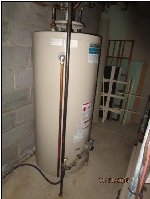
5.2 Item 2(Picture) Water heater
