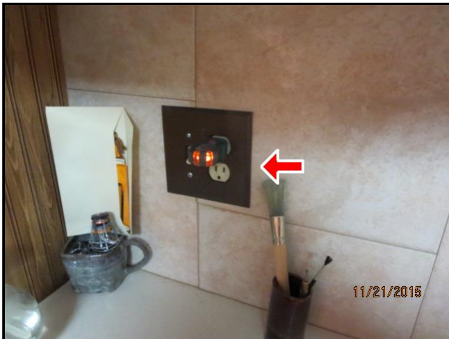
3.4 Item 1(Picture) Non GFCI outlet
