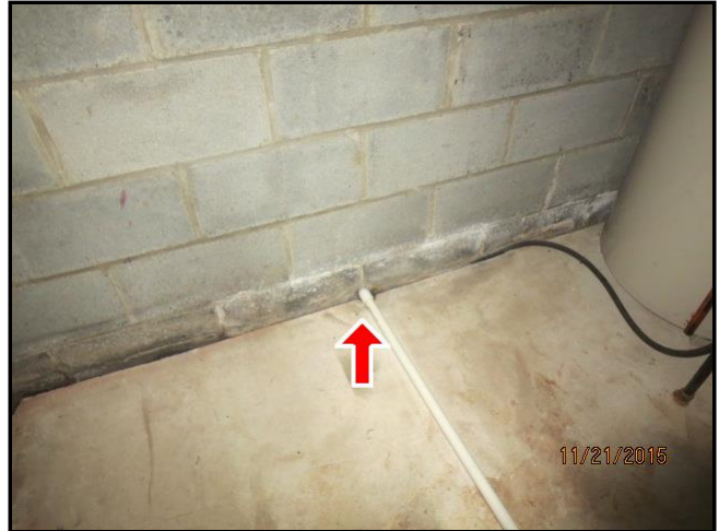
6.0 Item 6(Picture) Efflorescence
