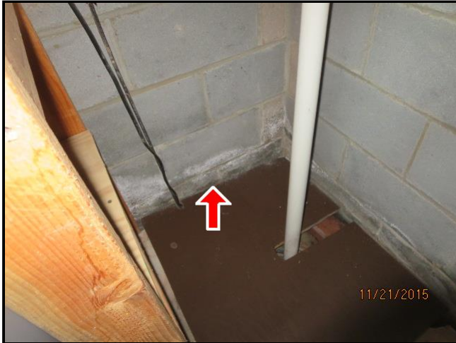
6.0 Item 5(Picture) Efflorescence
