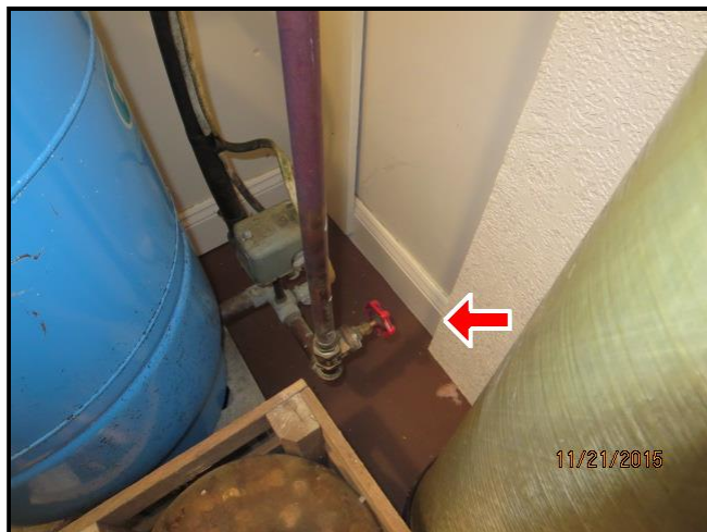
5.3 Item 1(Picture) Main Water shut off
