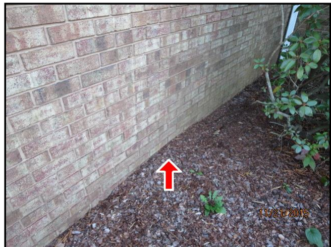
2.0 Item 5(Picture) Missing or buried weep holes
