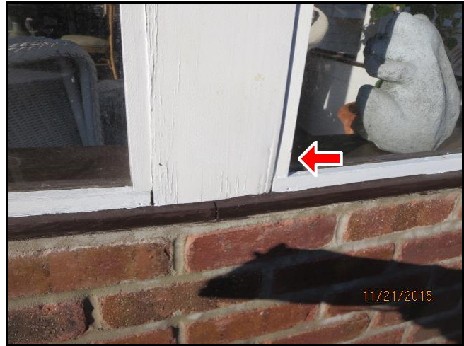
2.0 Item 2(Picture) Wood Rot
