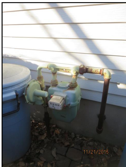
5.5 Item 1(Picture) Gas meter
