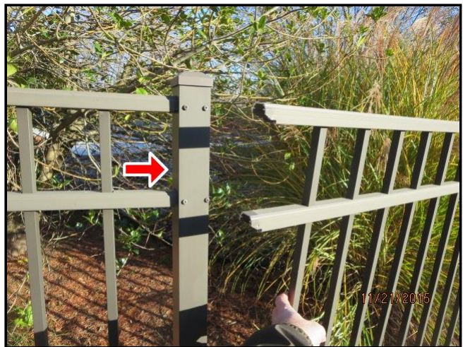
11.15 Item 4(Picture) Damaged section
