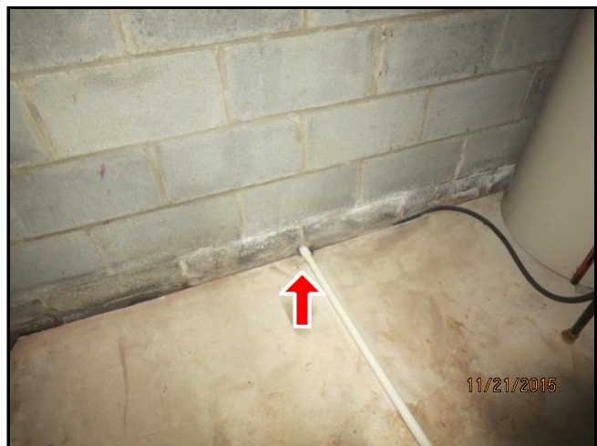
6.0 Item 6(Picture) Efflorescence
