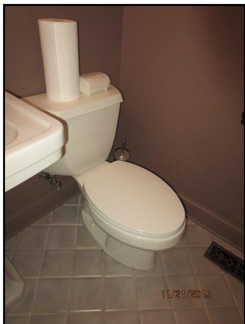
5.1 Item 3(Picture) Loose toilet
