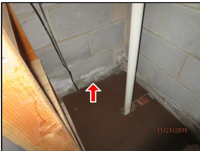
6.0 Item 5(Picture) Efflorescence
