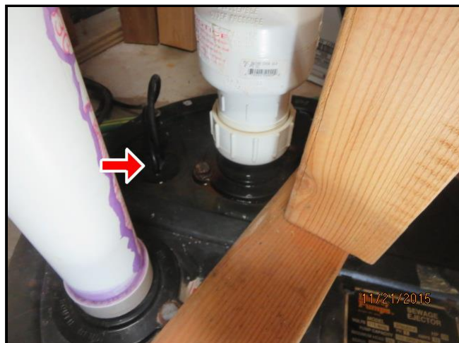
5.1 Item 1(Picture) Pump up system leak
