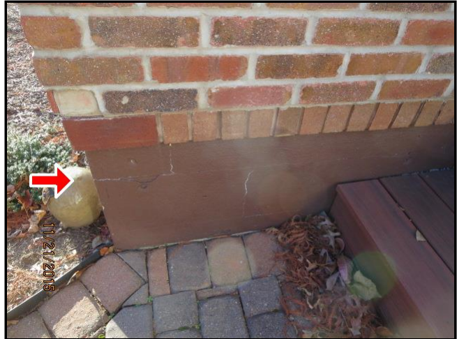
6.0 Item 2(Picture) Wall cracks
