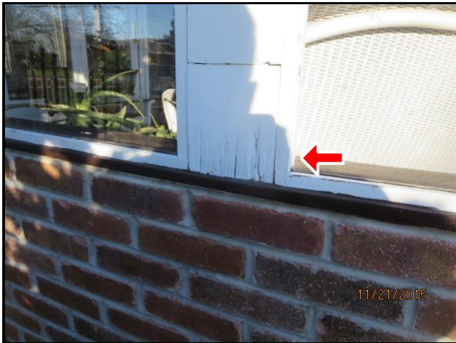
2.0 Item 3(Picture) Wood Rot
