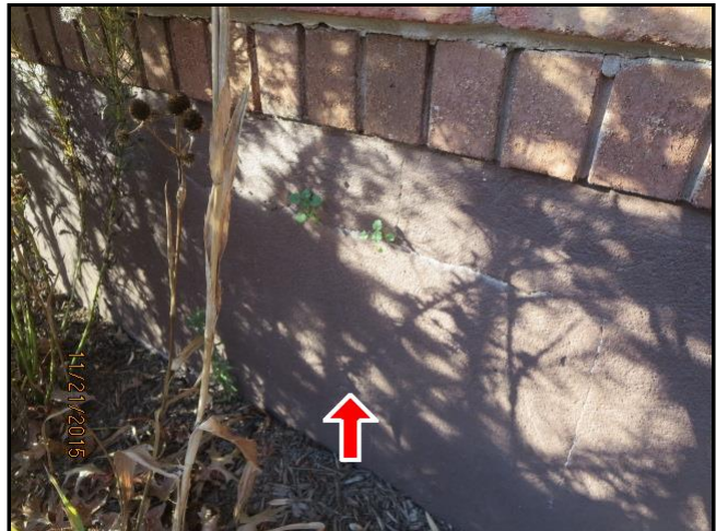
6.0 Item 4(Picture) Wall cracks
