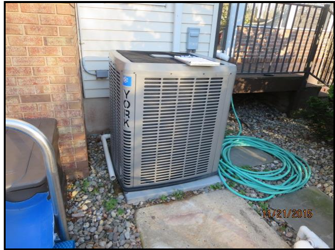
4.8 Item 2(Picture) 2008 Condenser
