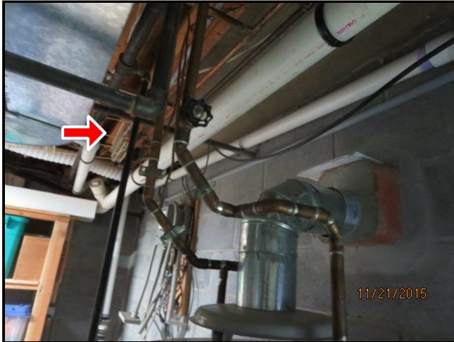
5.2 Item 1(Picture) Missing bond wire
