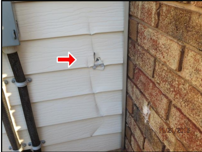
2.0 Item 6(Picture) Damaged siding
