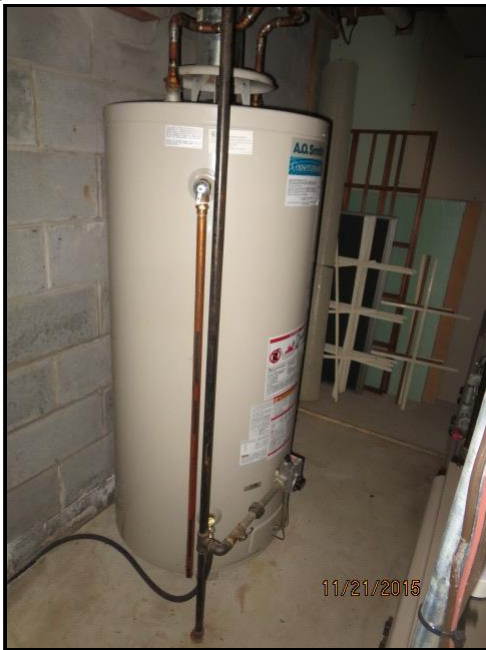
5.2 Item 2(Picture) Water heater
