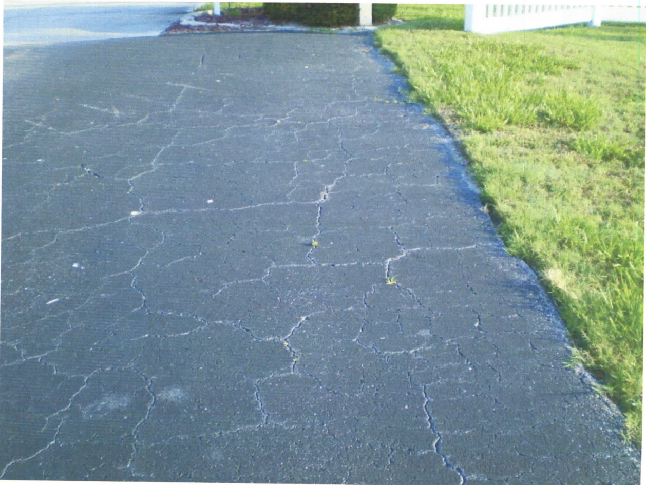
Photo#2- Typical Random Block Type Cracking
