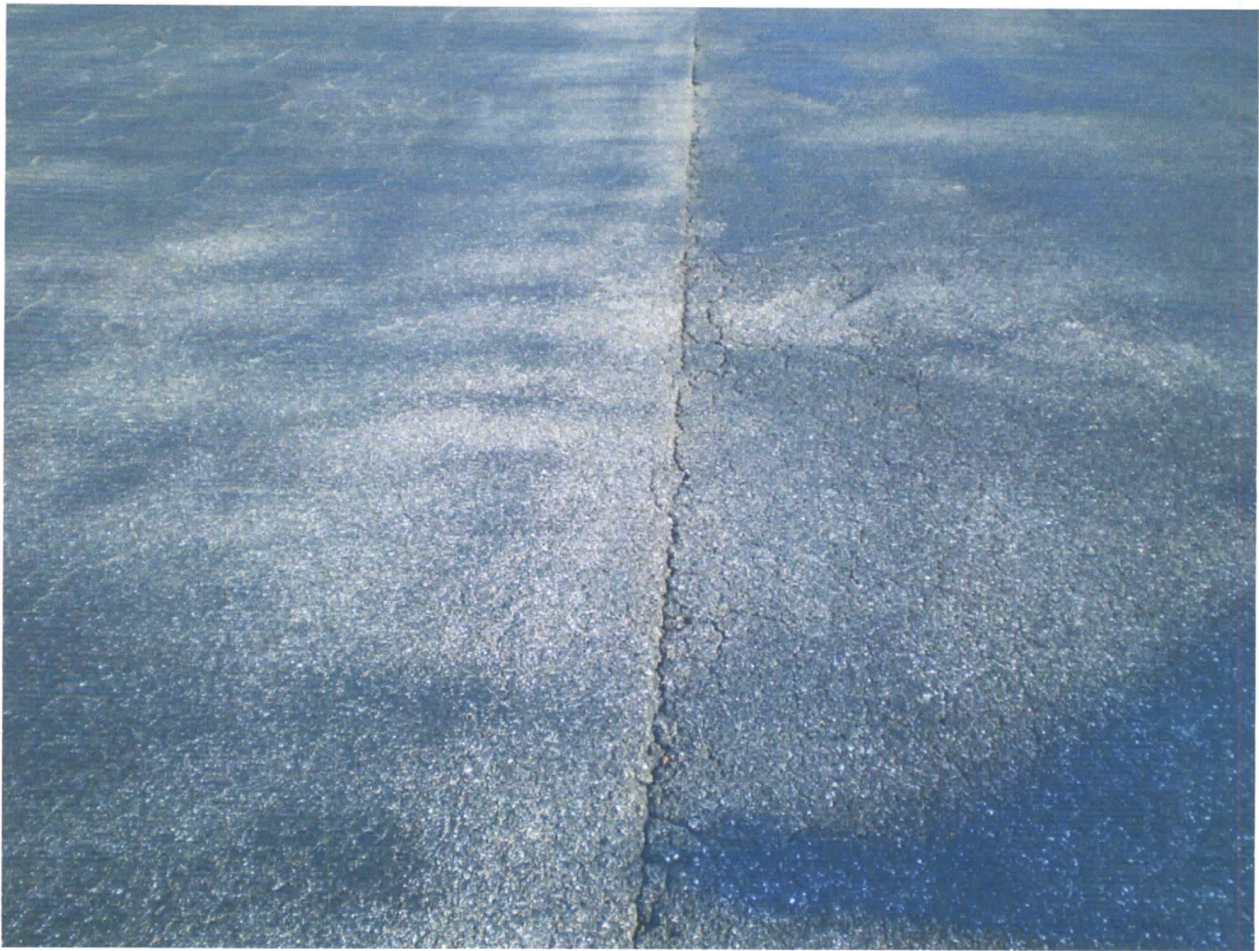
Photo#3- Typical Open Pavement Joint
