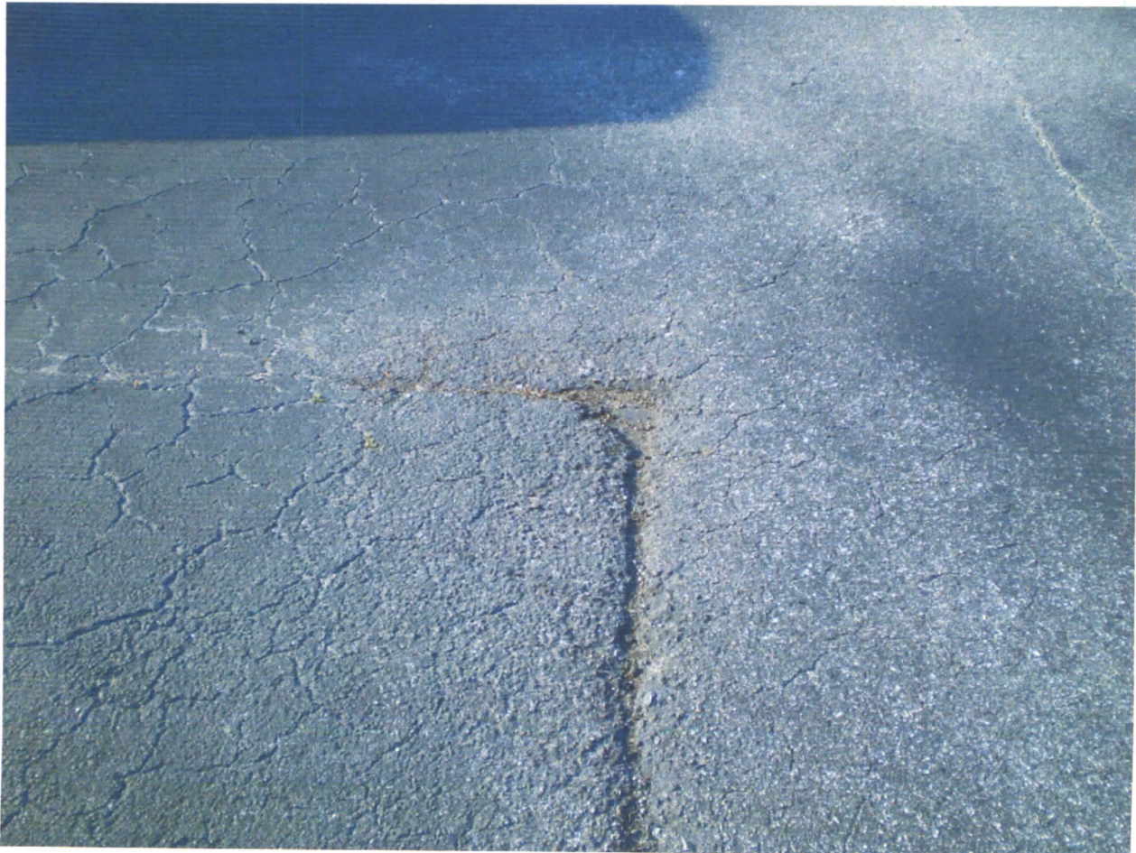
Photo#4- Typical Open Pavement Joint
