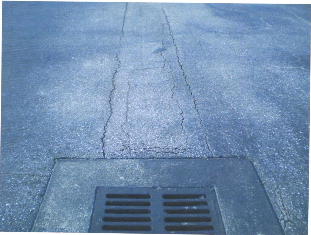
Photo#6- Cracking Near Low Point in Pavement Next to Grate Inlet
