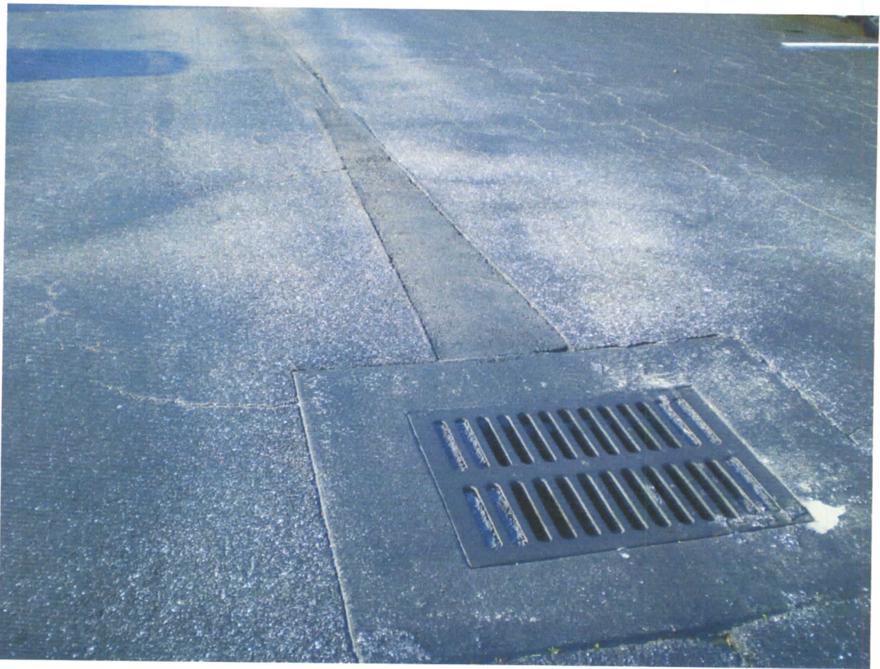
Photo#5- Patch in Low Point in Pavement Adjacent to Grate Inlet
