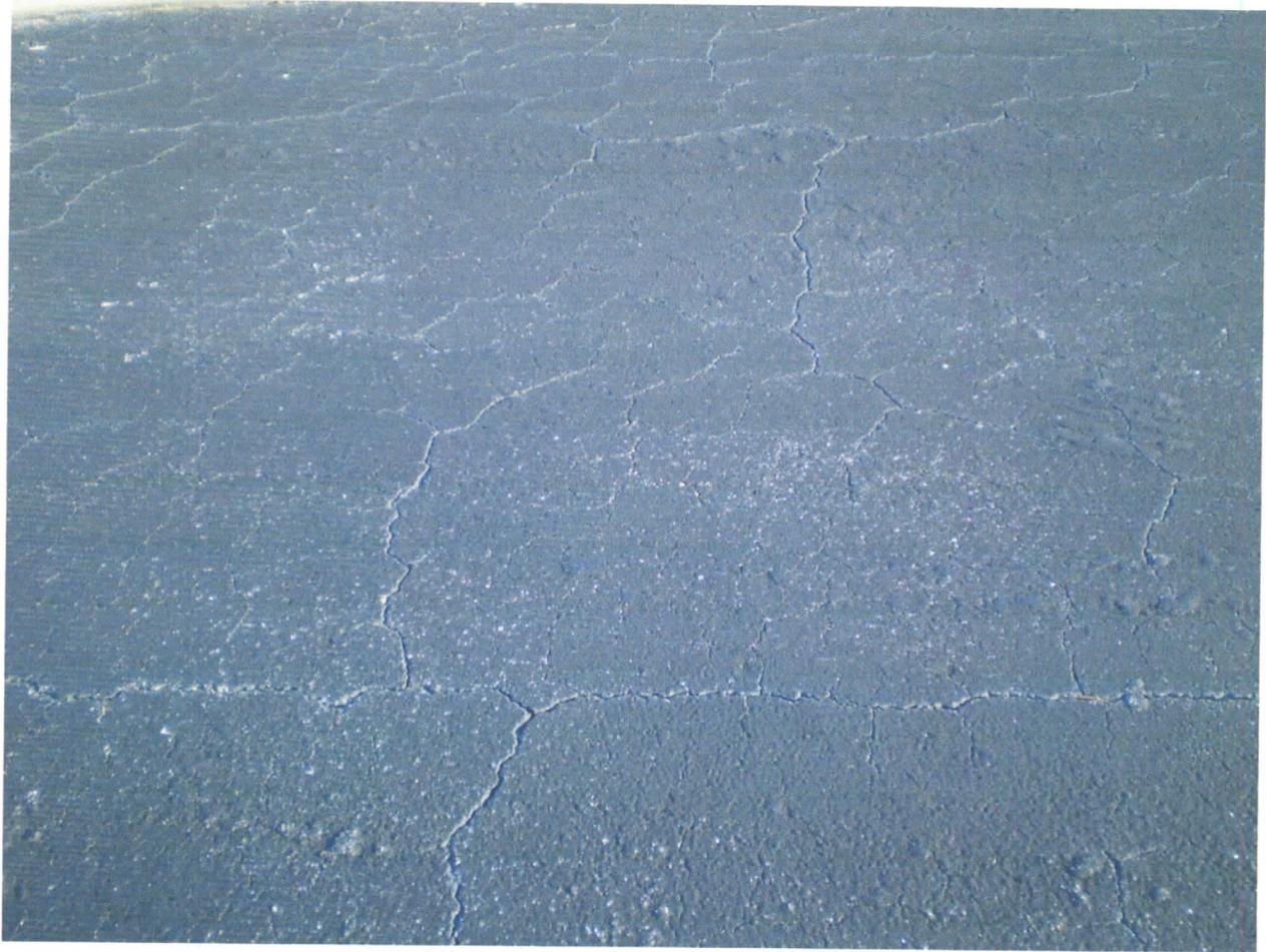
Photo#1- Typical Random Block Type Cracking
