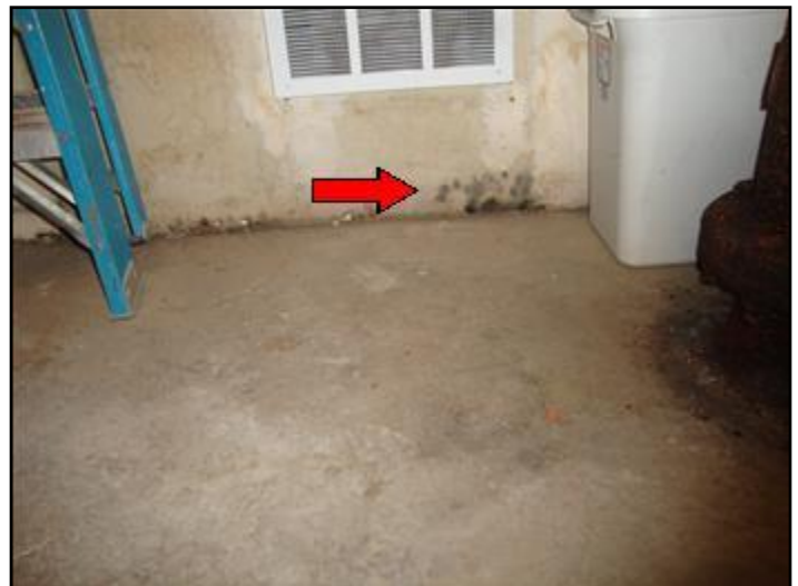
33. A water stain was noted. Refer to the...
