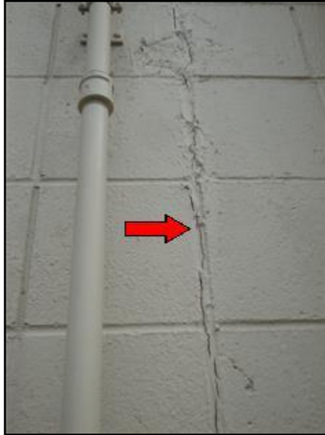
49. Deteriorated caulking wall expansion joints
