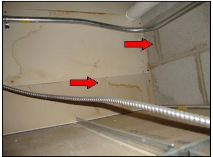
35. A water stain was noted. Refer to the...
