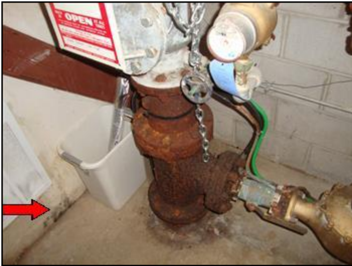
34. A water stain was noted. Refer to the...
