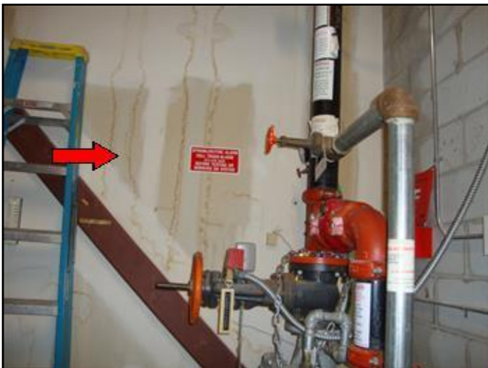
32. A water stain was noted. Refer to the...
