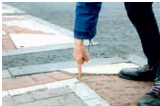
Fig. 2.8 Damage to a speed cushion
