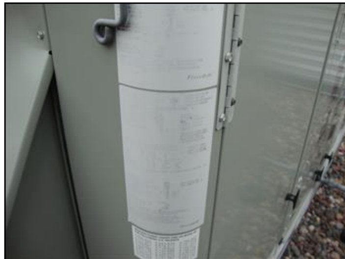
Illegible - heating capacity and age could...
