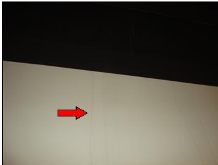
A water stain was noted
