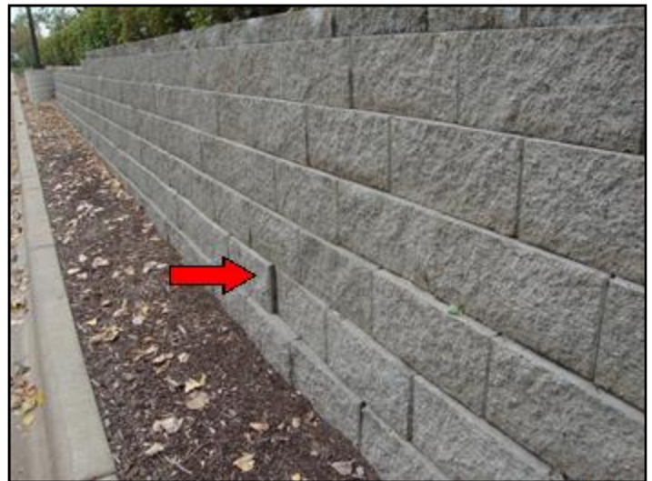
Minor impact damage
