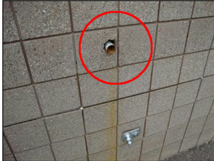
Unknown drain pipe?
