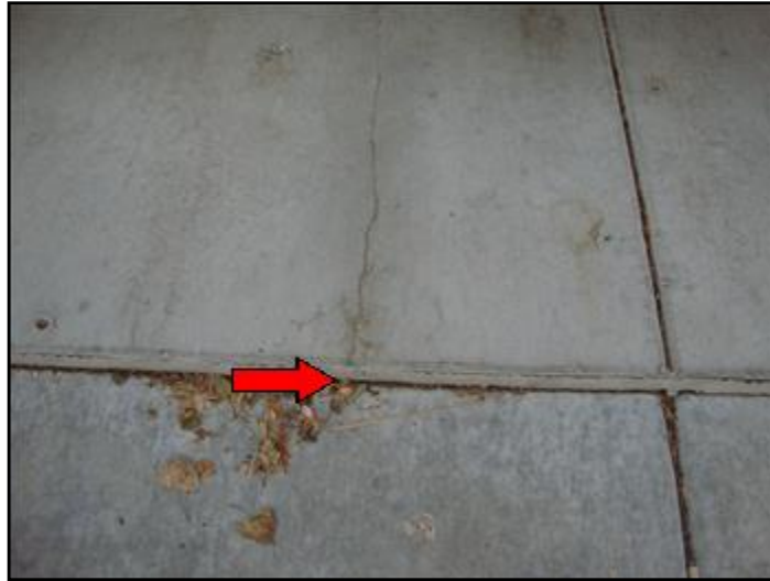
The sidewalk has settled
