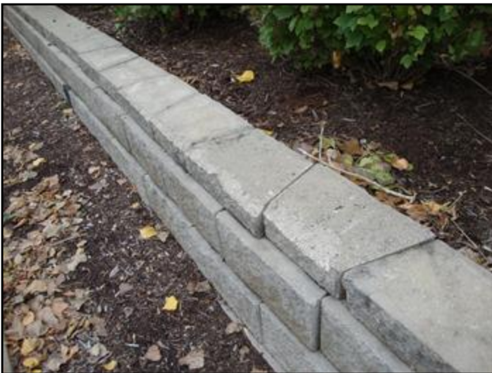
Minor impact damage
