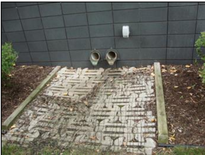
Discharging too close to building structure...
