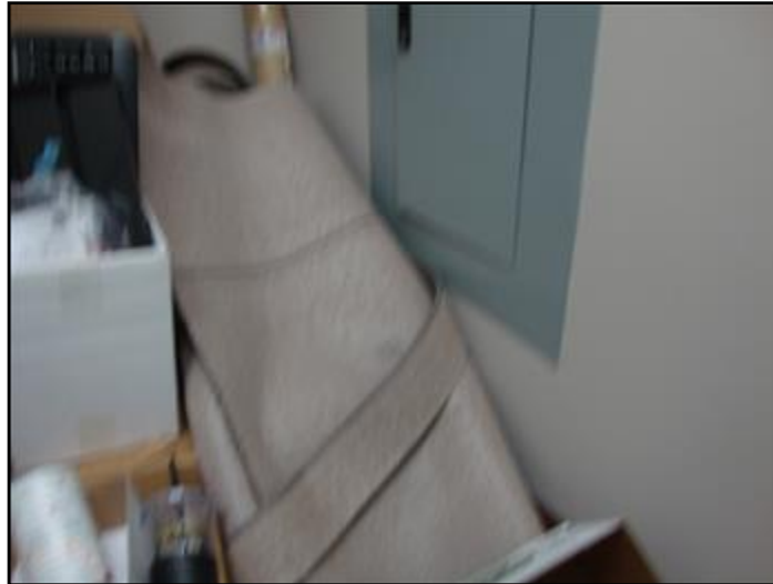
Storage within one meter of electrical...
