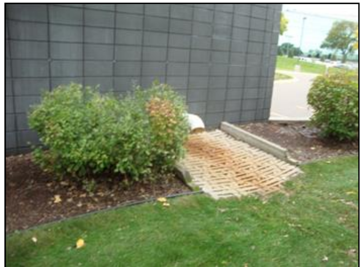
Discharging too close to building structure...
