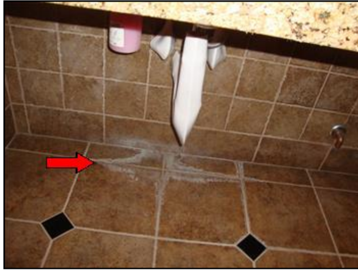
Evidence of past leakage noted
