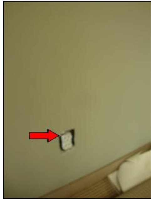
Missing on switches, outlets and junction...
