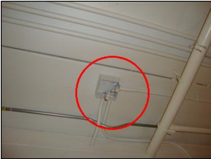
Missing on switches, outlets and junction...
