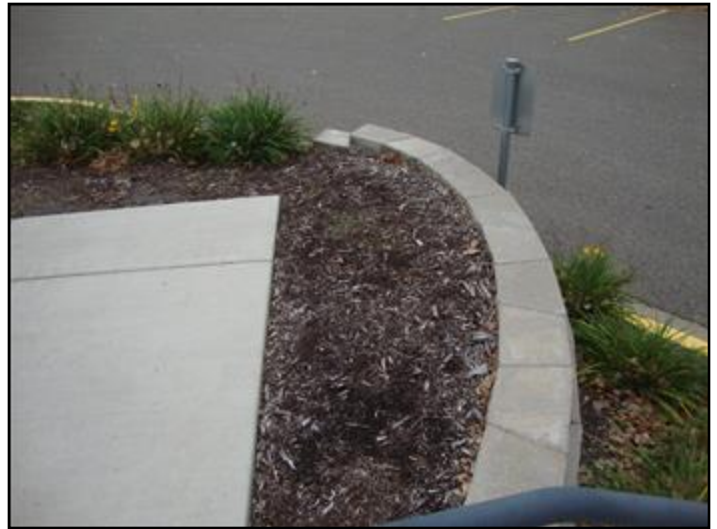
Dead and missing
