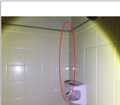
Recommend caulk/grout as needed
