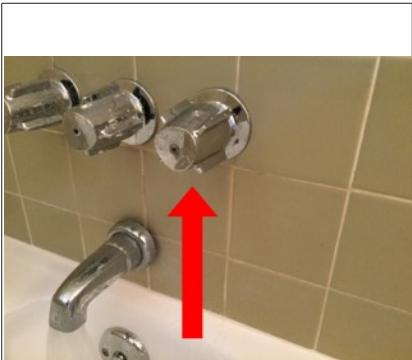
Water leaks from cold water handle during operation. Recommend consulting a licensed plumber for evaluation / repair. see photo.
