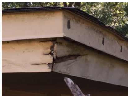
Wood rot on Fascia
