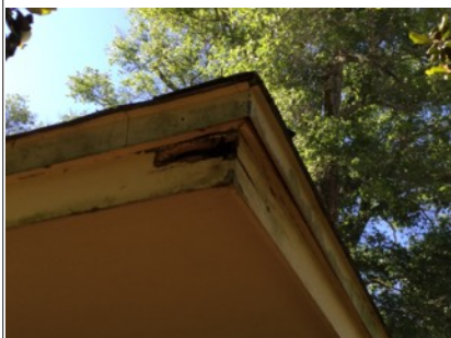
Wood rot on Fascia on South West corner
