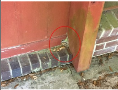
Wood rot on wood siding adjacent to front porch
