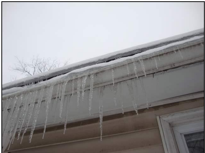
8. Vulnerable to ice damming
