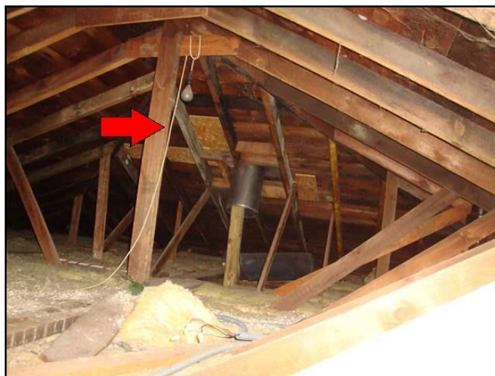
53. Extension cord used as permanent wiring
