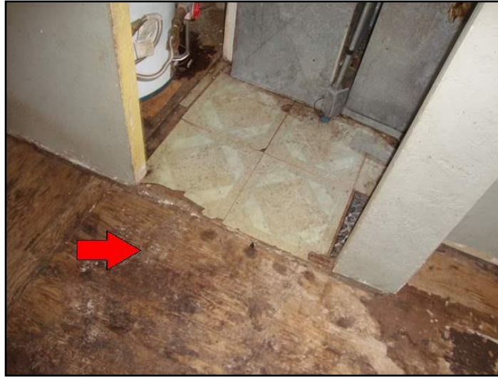
96. Loose or missing pieces
