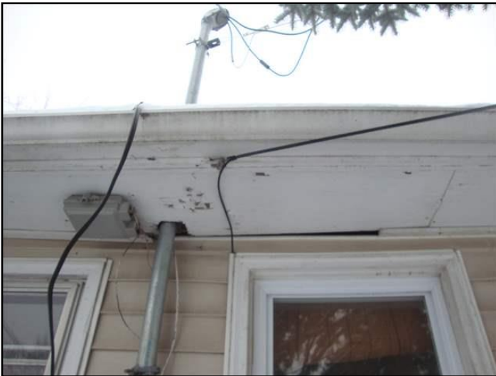
13. Paint or stain needed
