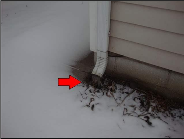
11. Downspouts end too close to building
