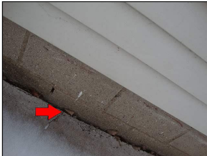
28. Unsealed gap at building
