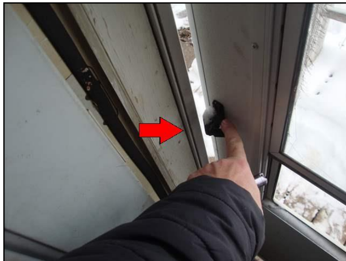
109. Latch not effective on exterior door
