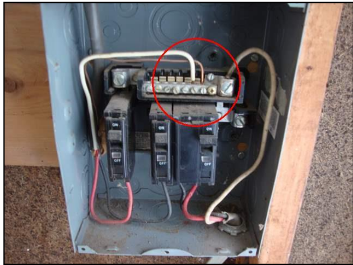
43. Neutral bonded to ground downstream of box
