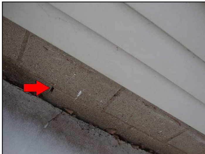
34. Mortar deteriorating or missing
