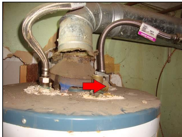
82. Discharge tube missing
