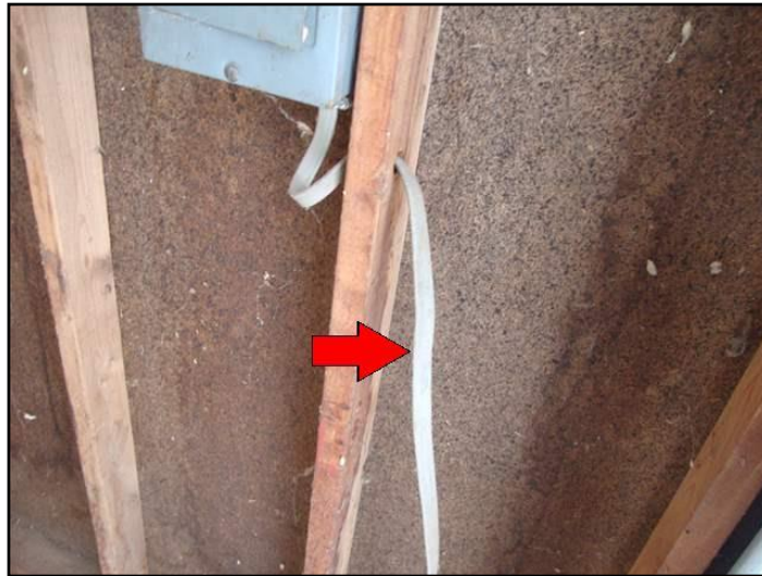
49. Not well secured
