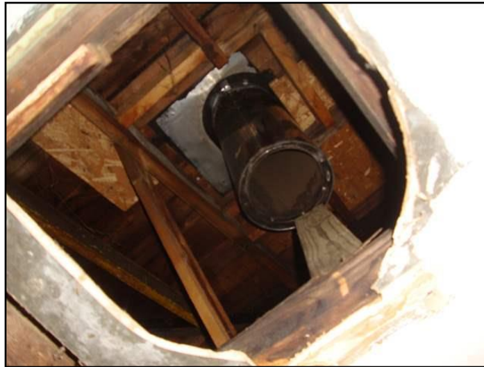
74. Gaps or voids
