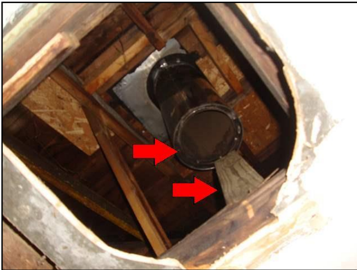
72. Sections not well secured
