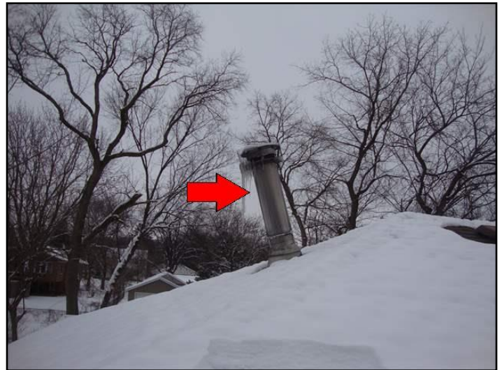
73. Sections not well secured
