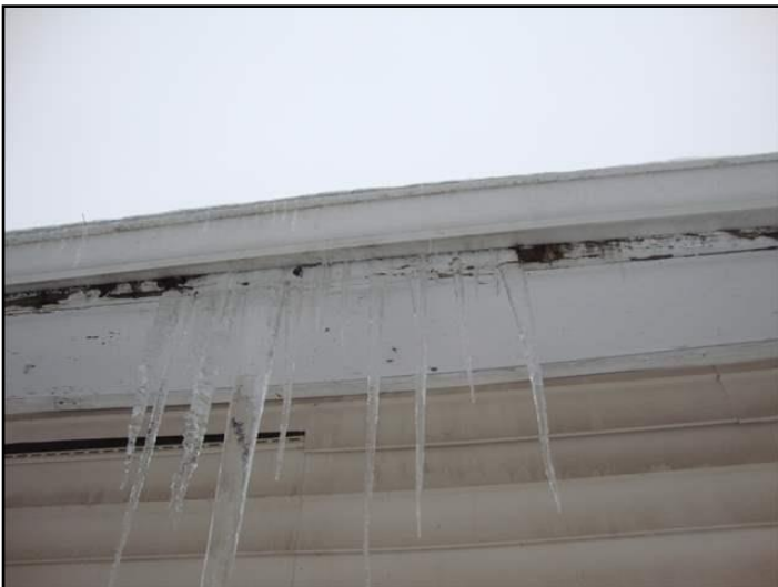
7. Vulnerable to ice damming
