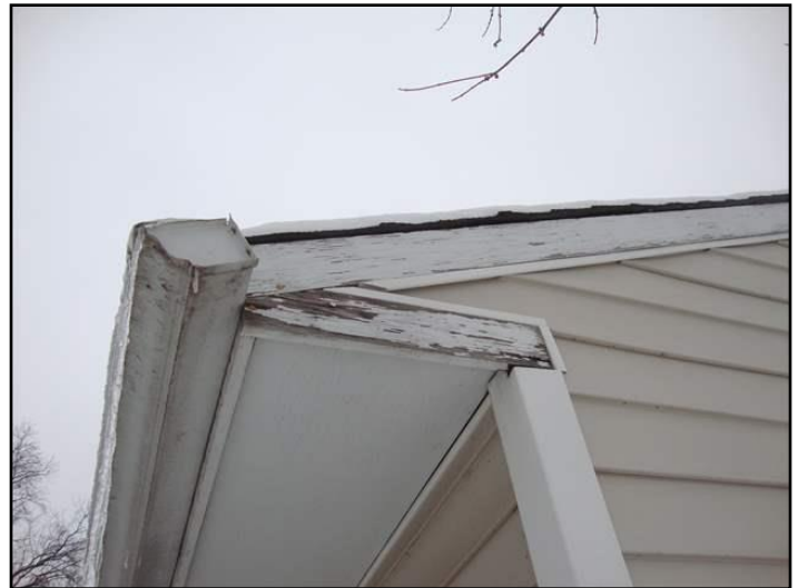
14. Paint or stain needed
