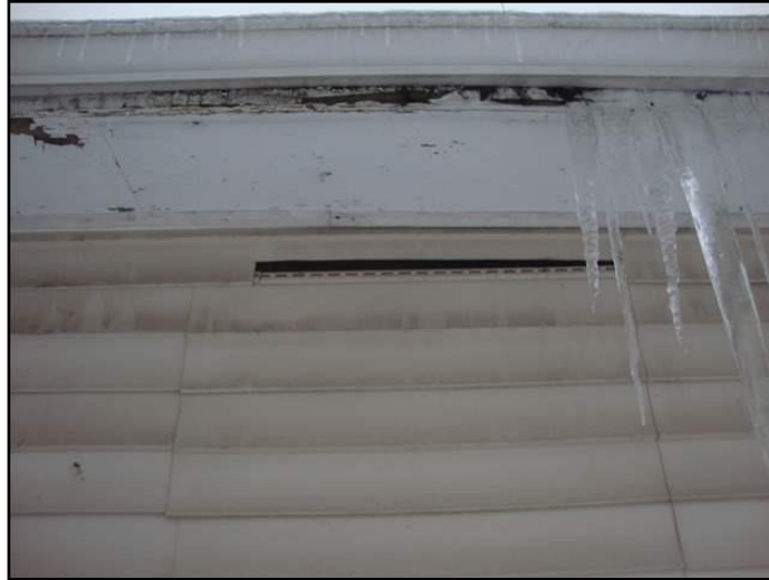
19. Loose or missing pieces
