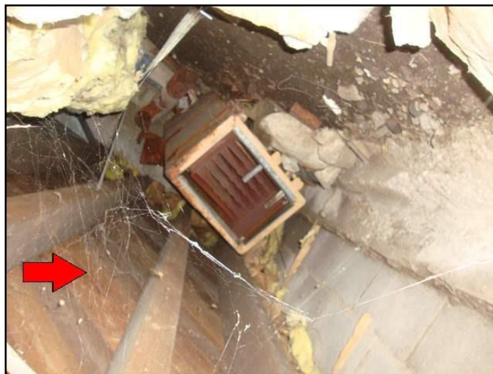
77. Too little insulation
