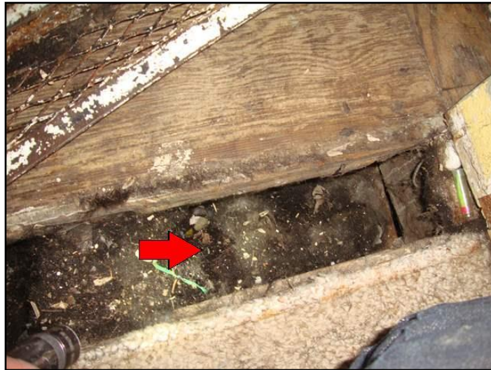
67. Dirty, obstructed or collapsed
