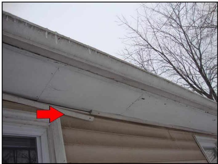
12. Loose or missing pieces
