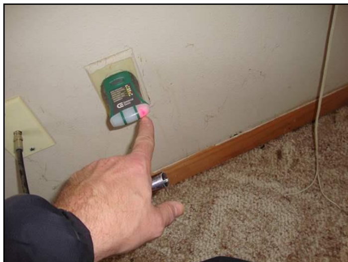
57. Ground needed for 3-slot outlet
