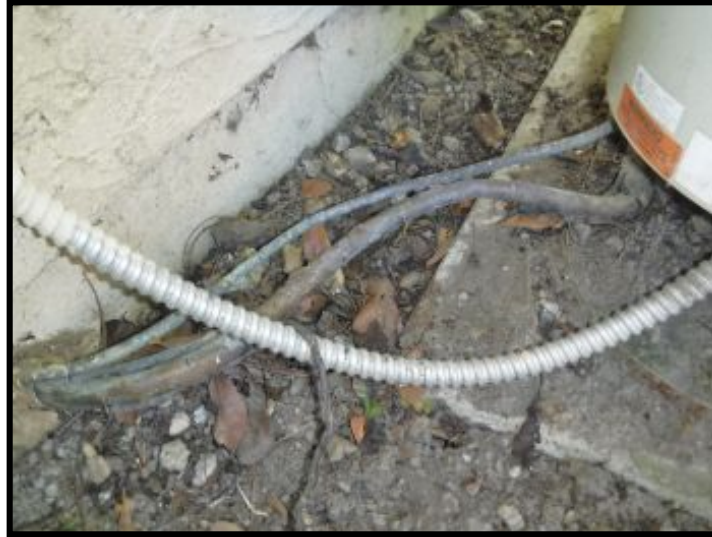
Missing insulation noted.
