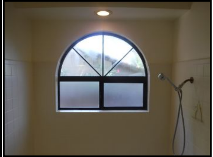
Loss of seal/condensation.
