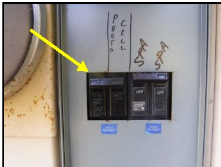
Main electrical shut off.
