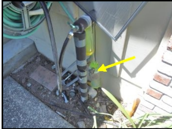
Main water shut off.
