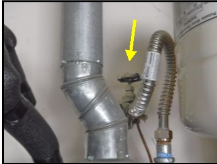
Water heater water shut off.
