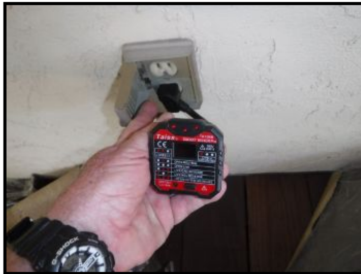
Outlet not operational at deck area.
