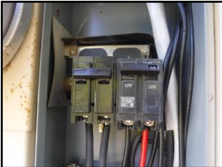
Main electrical panel.
