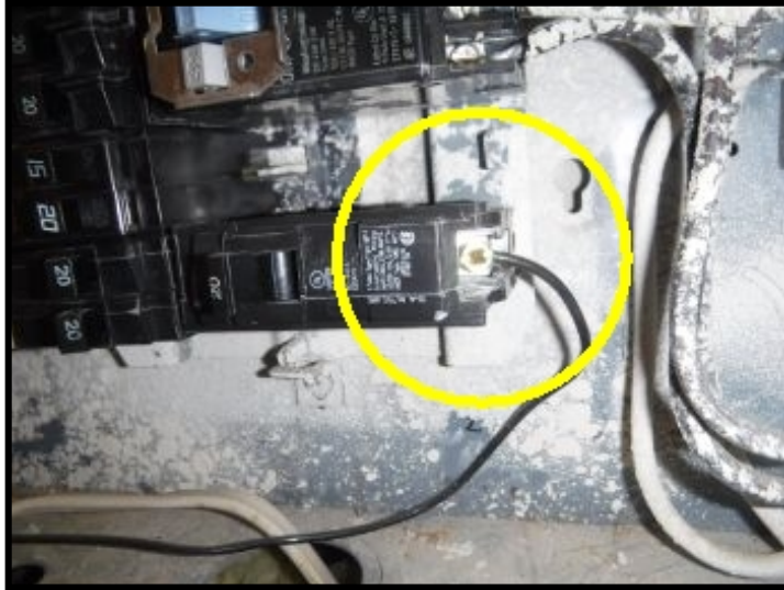
Wire size insufficient for breaker.
