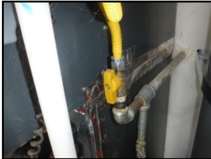
Furnace gas shut off.
