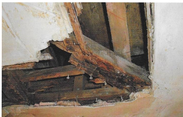
Figure 4 - wet rot due to water ingress due to aged roof covering
