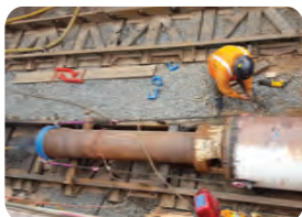
The Foundry, CO
