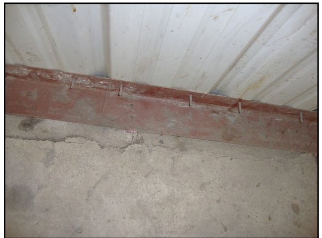
144 : Interior Defects - Loose Fasteners at Mezzanine Wall
