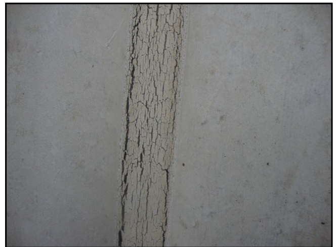
102 : Exterior - Deteriorated Expansion Joint 4
