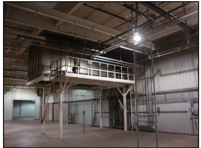
136 : HVAC - Make Up Air Unit
