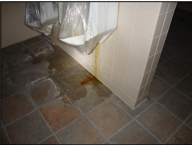
33 : Plumbing - Leak @ 2nd Floor Office 1
