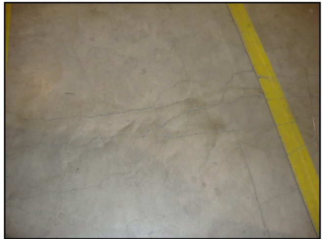
142 : Interior Defects - Floor Cracks
