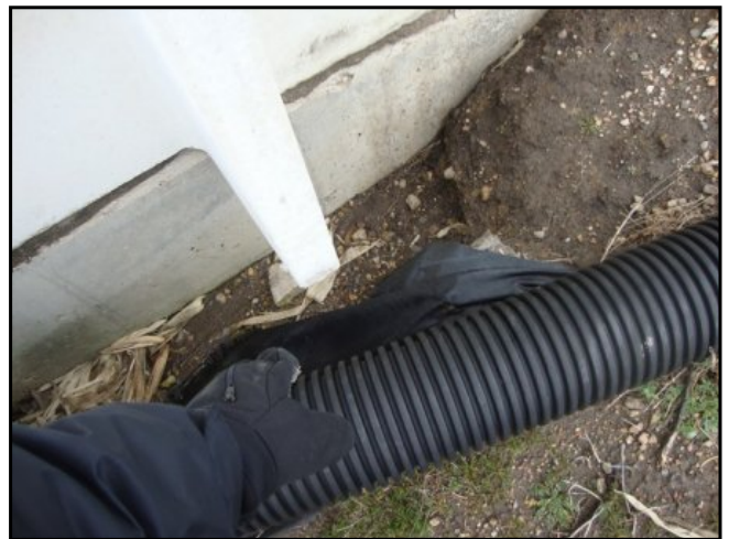
54 : Site - Erosion at SW Docks
