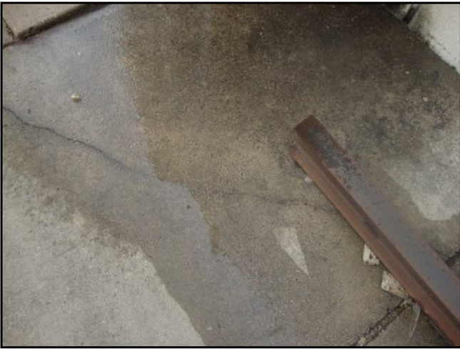
127 : Flatwork - Settled - Poor Drainage 2 Near S5
