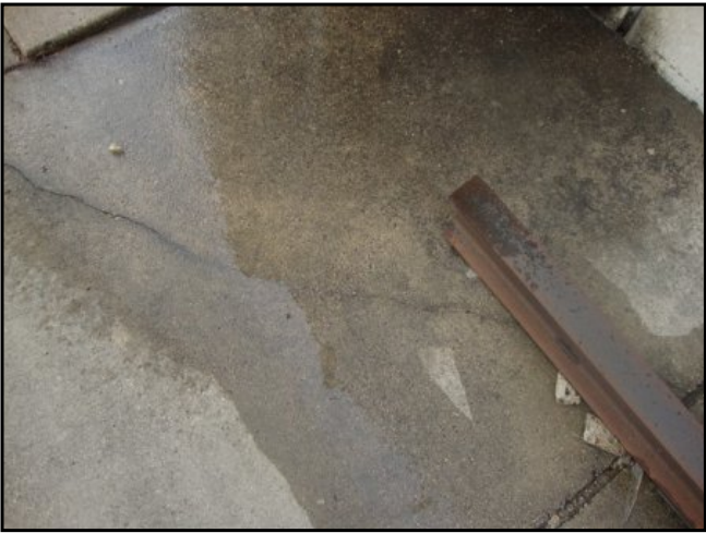
61 : Site - Poor Drainage - Settled Sidewalk 2
