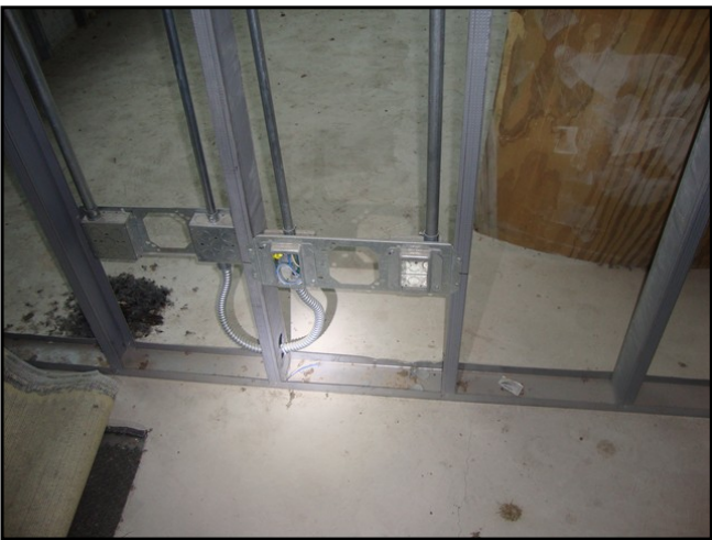
11 : Electrical - Missing Cover Plate 3
