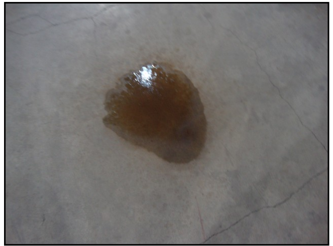
46 : Roof - Leak @ Mezzanine Manufacturing
