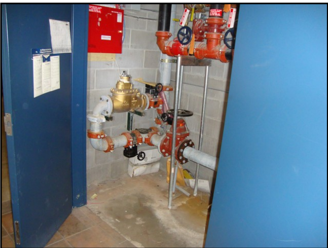
41 : Plumbing - Water Meter
