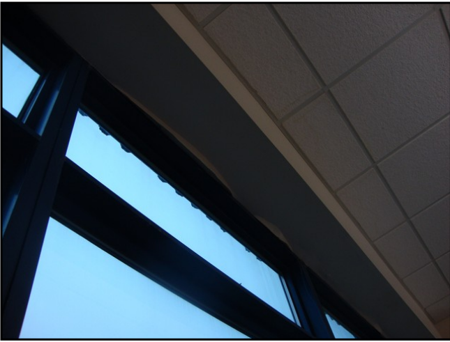
151 : Interior Defects - Office Water Damage 4
