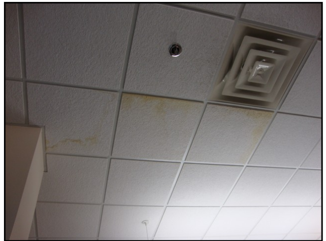
154 : Interior Defects - Office Water Damage 7
