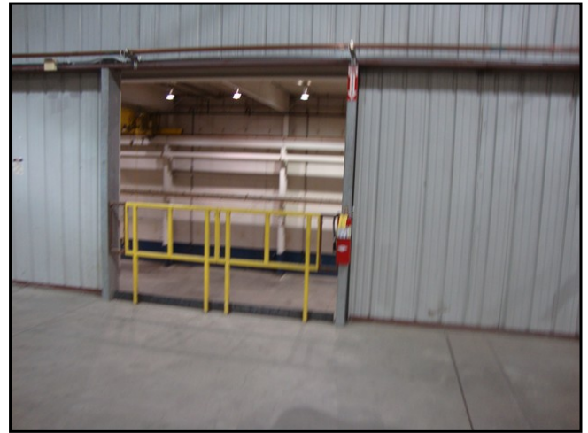
146 : Interior Defects - Missing Filler At Guard Rail 2
