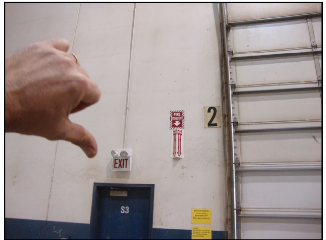
22 : Electrical - Inoperable Exit Light S3
