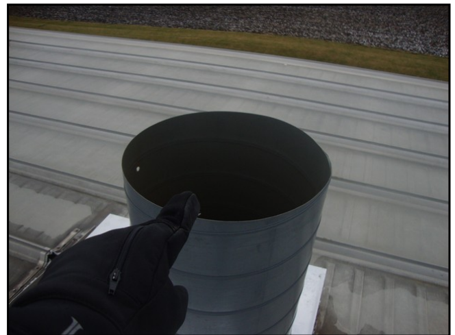
138 : HVAC - Recommend Capping or Removing Abandoned Exhaust Duct 1
