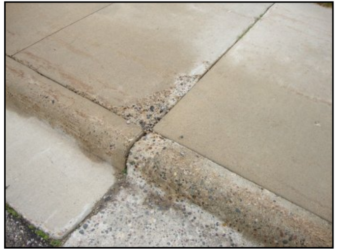
128 : Flatwork - Spalling or Mechanical Damage
