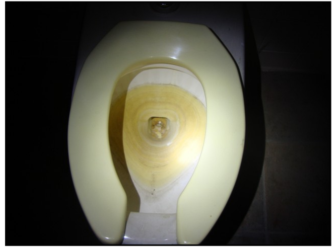
32 : Plumbing - Dry Traps
