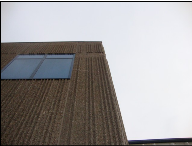
75 : Structure - Cracks Repaired With Sealant @ Office 4
