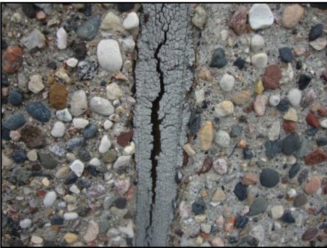
99 : Exterior - Deteriorated Expansion Joint 1
