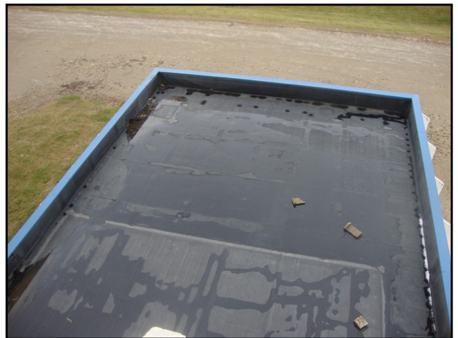
42 : Roof - Debris on Roof
