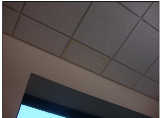
150 : Interior Defects - Office Water Damage 3
