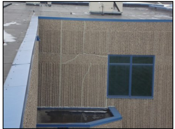
76 : Structure - Cracks Repaired With Sealant @ Office 5
