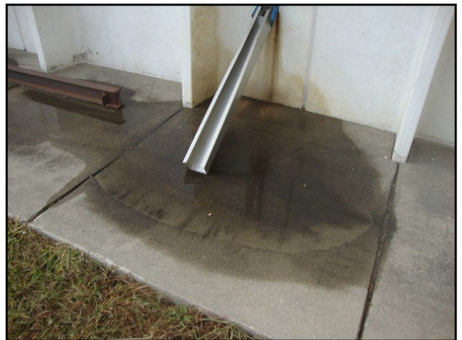
60 : Site - Poor Drainage - Settled Sidewalk 1
