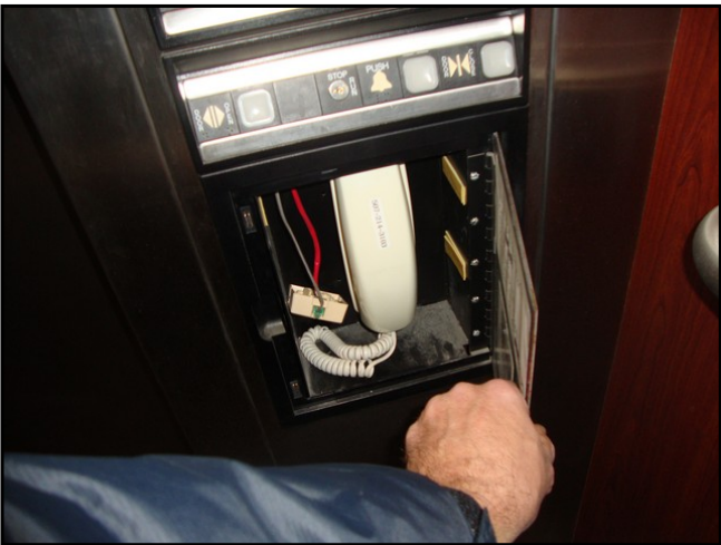
93 : Vertical Transportation - Communications
