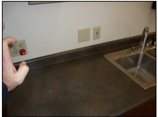
16 : Electrical - No GFCI Near Sink 2
