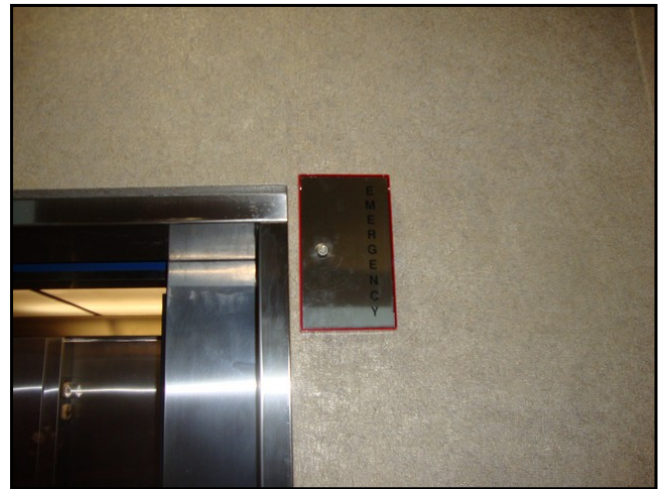
94 : Vertical Transportation - Emergency Key Box
