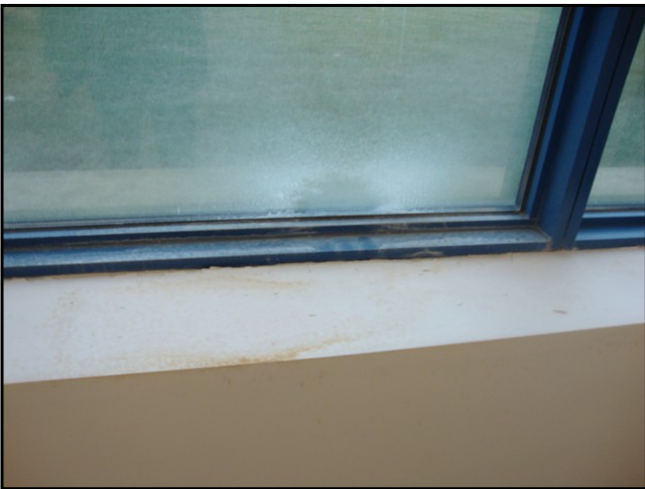
153 : Interior Defects - Office Water Damage 6
