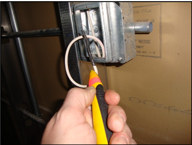
27 : Electrical - Missing Cover Plate 1
