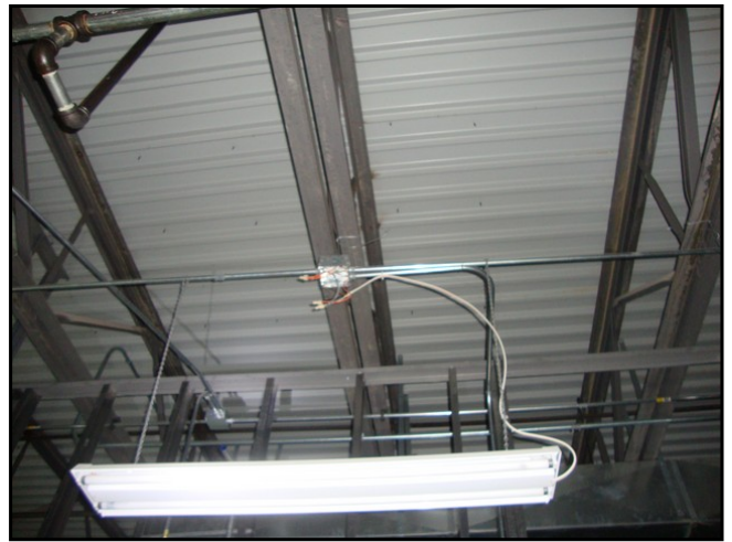
10 : Electrical - Missing Cover Plate 2
