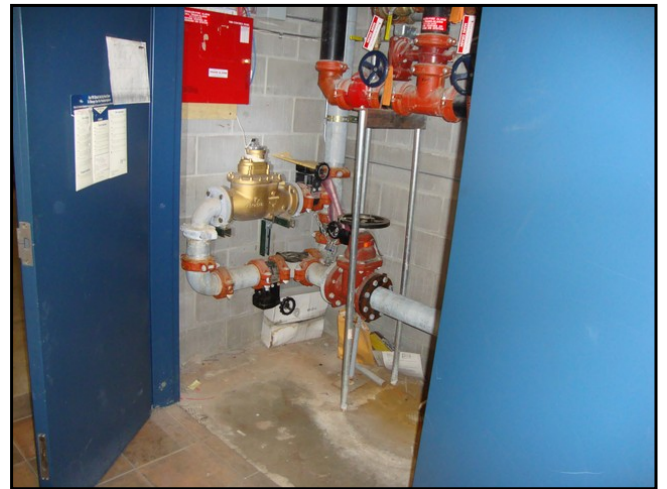
118 : Fire Protection - Sprinkler Riser Room
