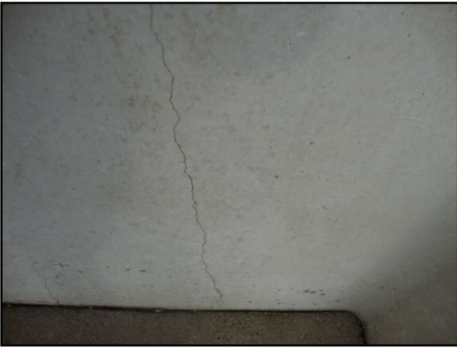
79 : Structure - Minor Cracks @ Warehouse 2
