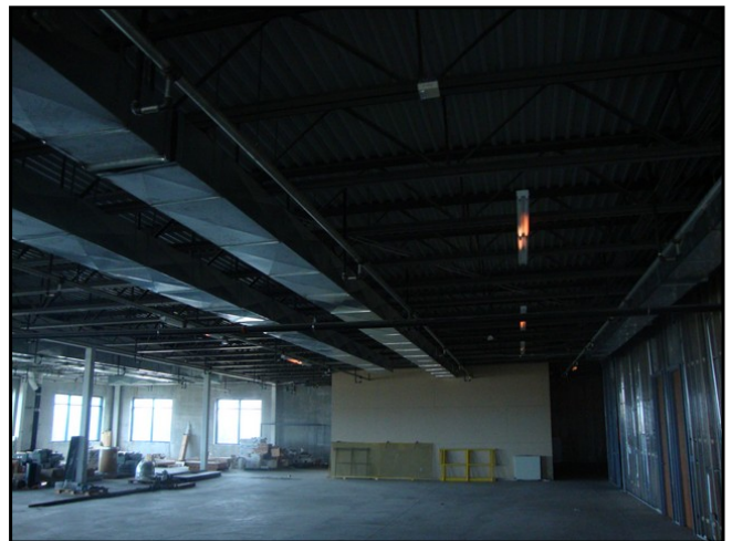
24 : Electrical - Inoperable Lights in Unfinished Office 2
