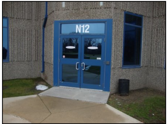
58 : Site - Missing downspout Extension
