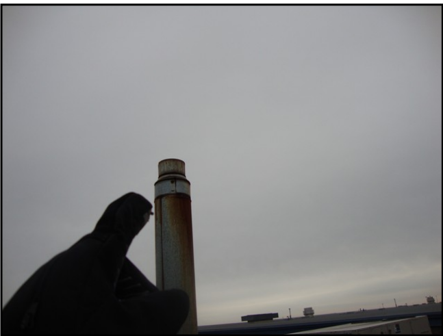
47 : Roof - Missing Rain Cap Suspect Source of Leak
