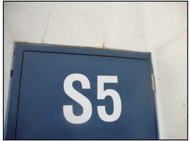
80 : Structure - Minor Cracks @ Warehouse 3
