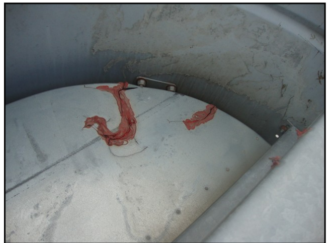
132 : HVAC - Cracked PRV Hood
