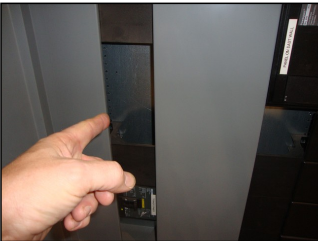
17 : Electrical - Opening @ Panel H4A - East Side Gantry
