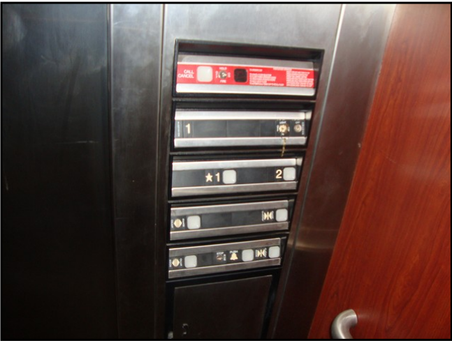
91 : Vertical Transportation - Cab Controls
