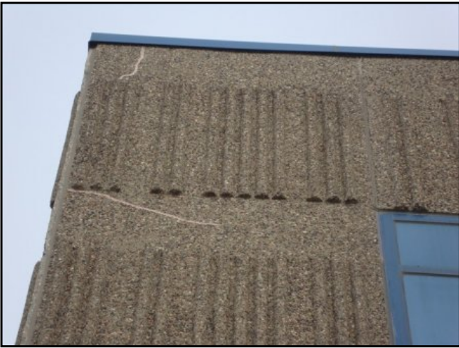
73 : Structure - Cracks Repaired With Sealant @ Office 2
