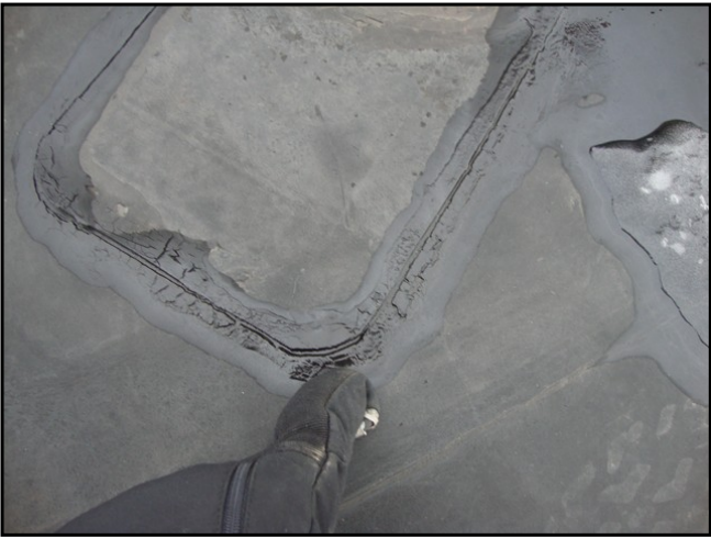
43 : Roof - Failing Seams 1
