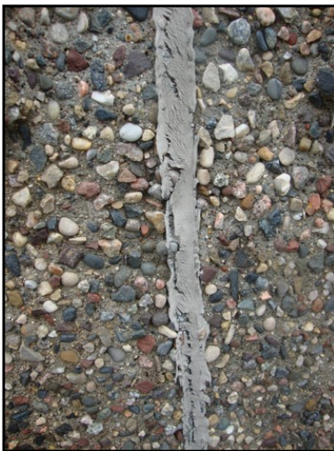
101 : Exterior - Deteriorated Expansion Joint 3
