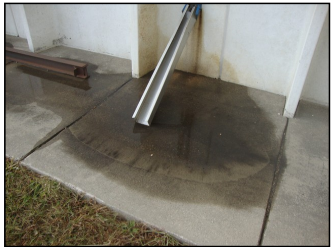
126 : Flatwork - Settled - Poor Drainage 1 Near S5
