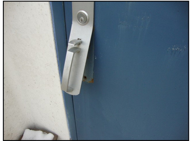
98 : Exterior - Damaged Door Hardware S5
