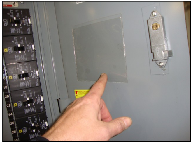
14 : Electrical - Missing Panel Index
