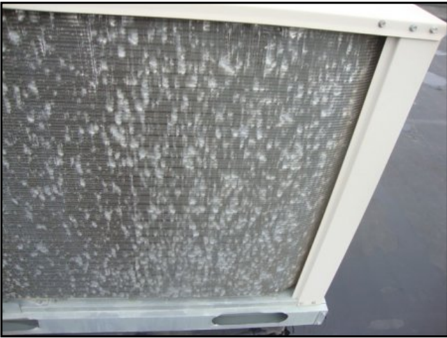
133 : HVAC - Damaged Coil
