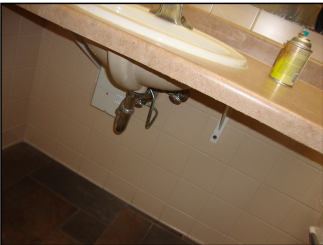
35 : Plumbing - Missing Insulation @ Sinks
