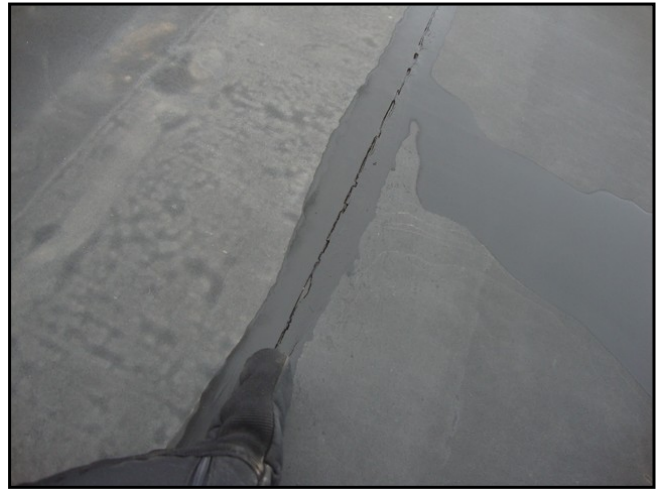
44 : Roof - Failing Seams 2
