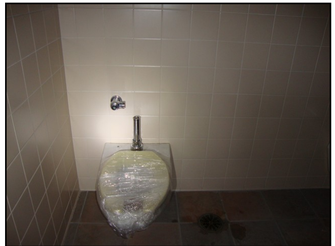
36 : Plumbing - Missing Valve @ 2nd Floor Office
