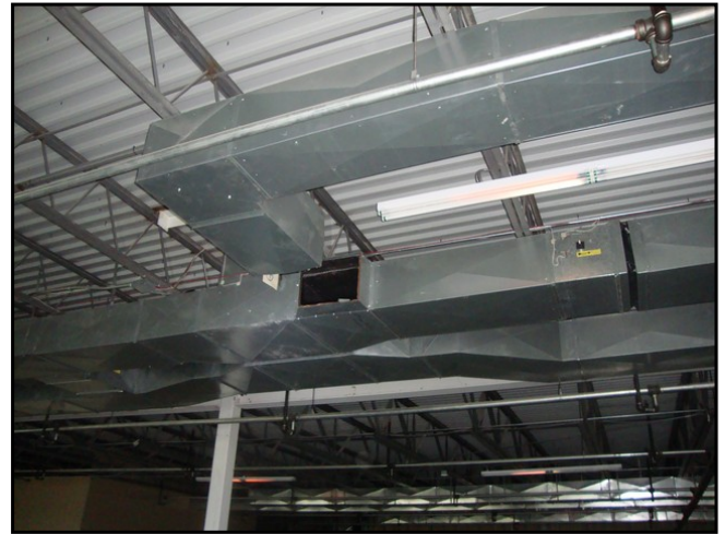
134 : HVAC - Disconnected 2nd Floor Office Duct
