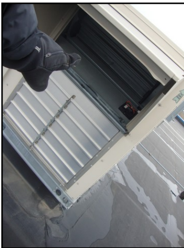
137 : HVAC - Missing Economizer Filter
