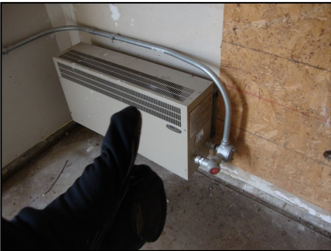
135 : HVAC - Electric Shed Heater
