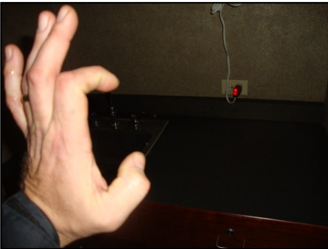
15 : Electrical - No GFCI Near Sink 1
