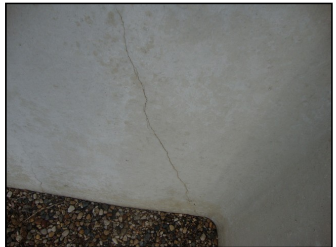
78 : Structure - Minor Cracks @ Warehouse 1
