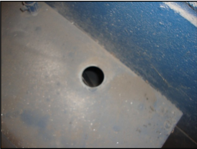
13 : Electrical - Missing Knock Out 2
