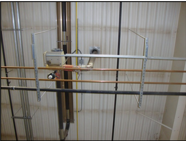
141 : HVAC - Typical Tube Heater
