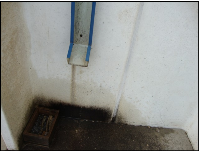
57 : Site - Missing Downspout Extension or Splash Guard
