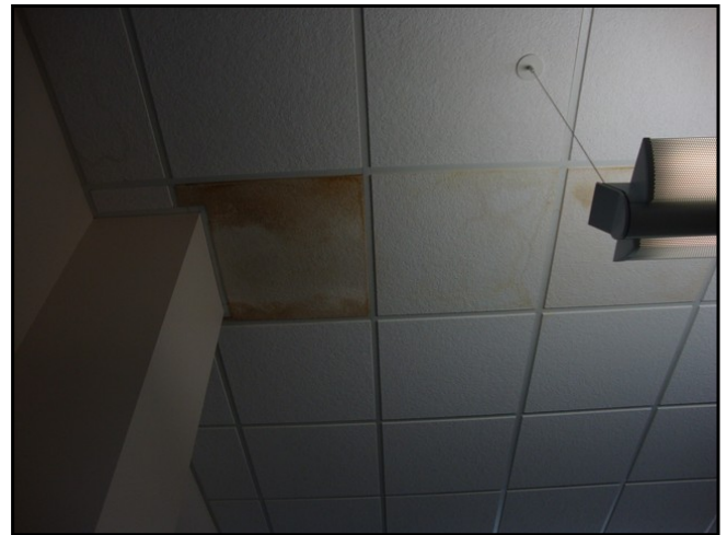
148 : Interior Defects - Office Water Damage 1
