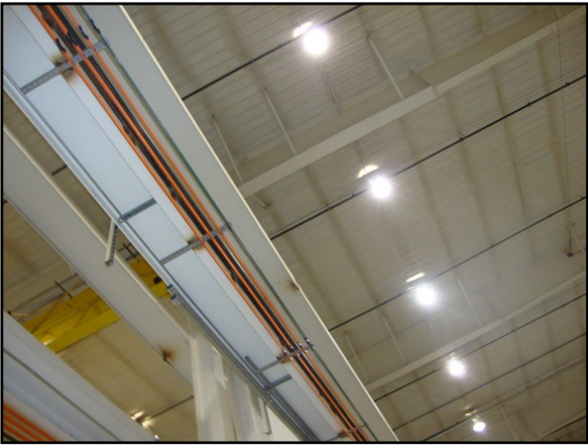
19 : Electrical - Recommend Warning Signs At Exposed Crane Feeders
