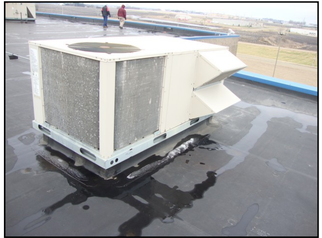
140 : HVAC - Typical RTU
