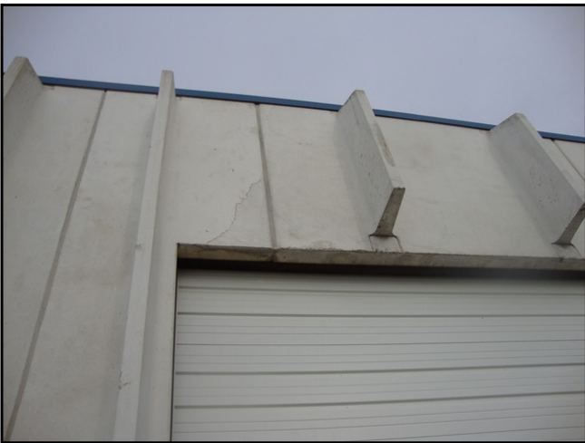
81 : Structure - Minor Cracks @ Warehouse 4
