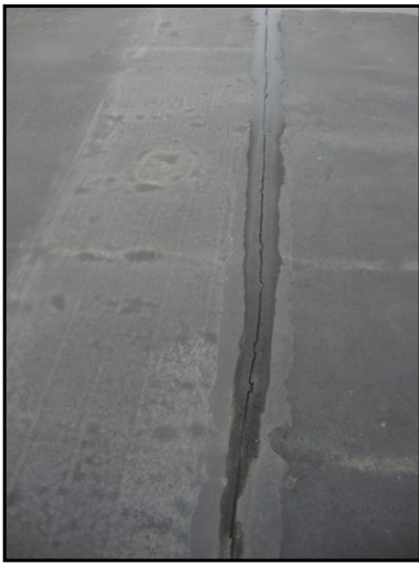
45 : Roof - Failing Seams 3
