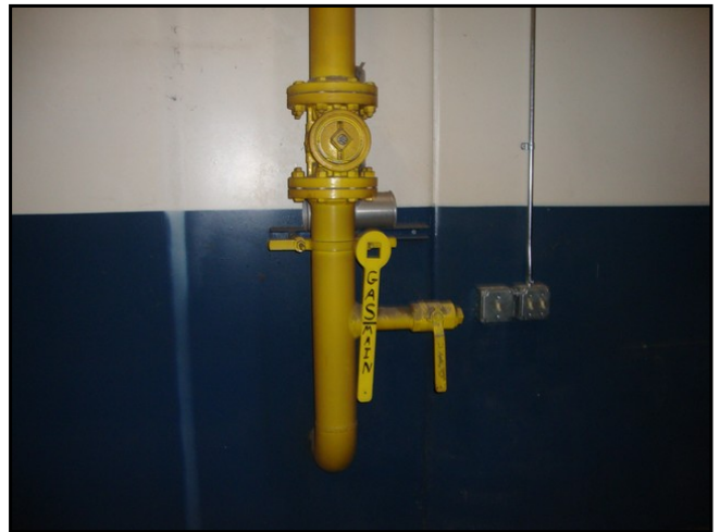
130 : Gas - Main Shut Off
