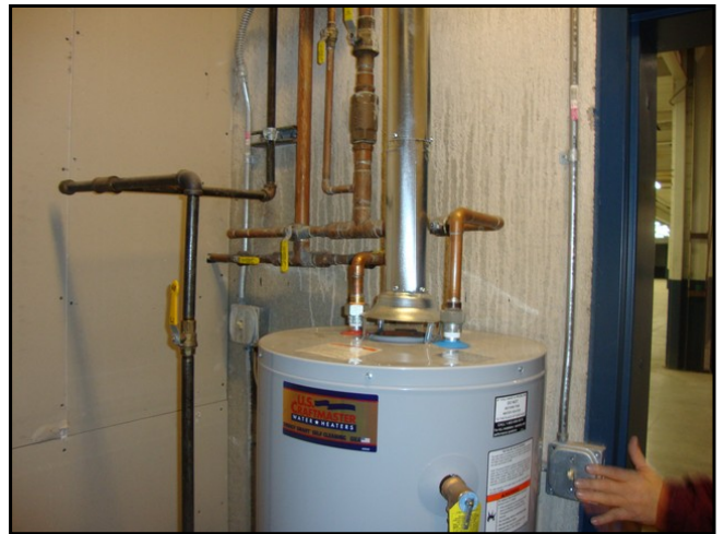
40 : Plumbing - Water Heater
