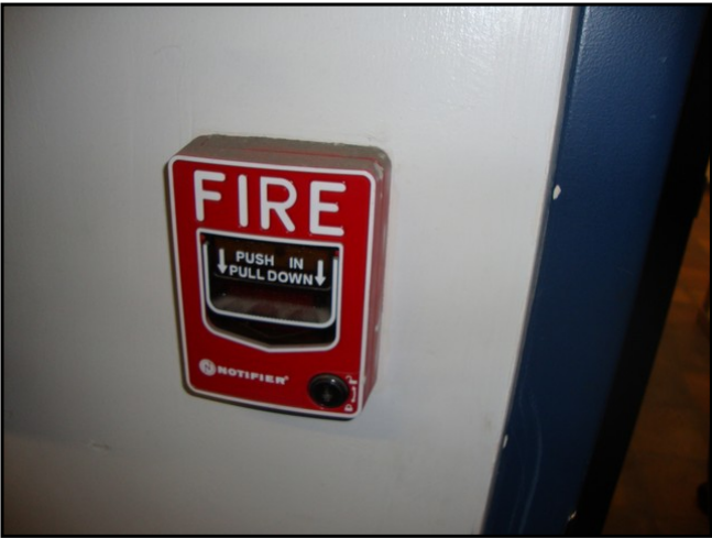
115 : Fire Protection - Pull Station
