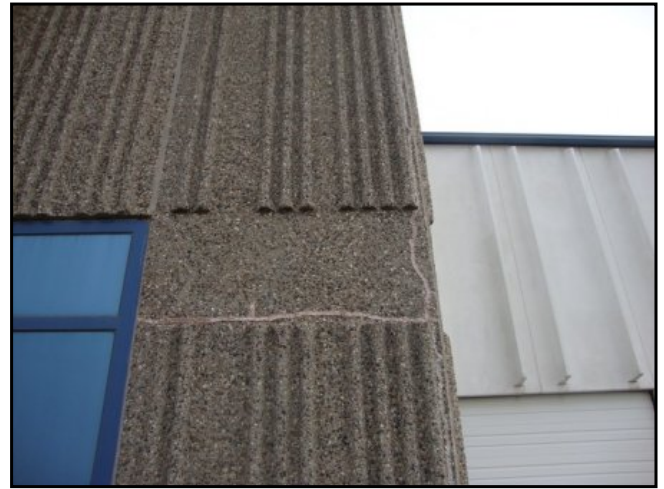
74 : Structure - Cracks Repaired With Sealant @ Office 3
