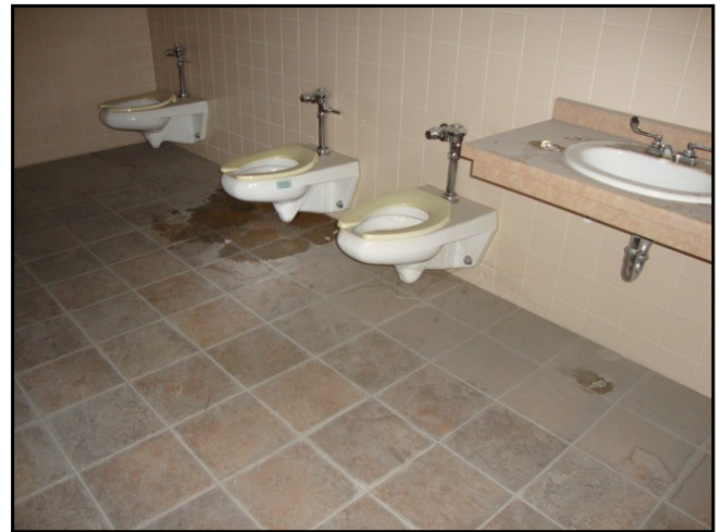
34 : Plumbing - Leak @ 2nd Floor Office 2
