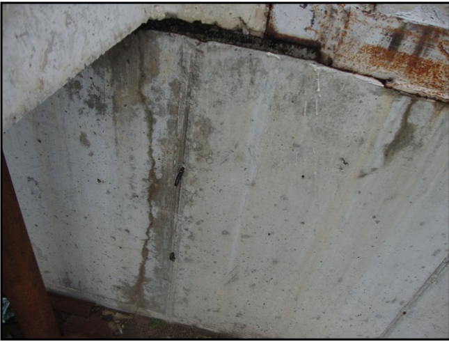
85 : Structure - Typical Cracks or Minor Damage at Dock Bays
