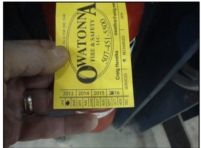
108 : Fire Protection - Extinguisher Inspection Tags Current
