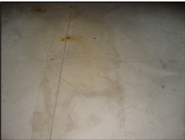
155 : Interior Defects - Patched Floor
