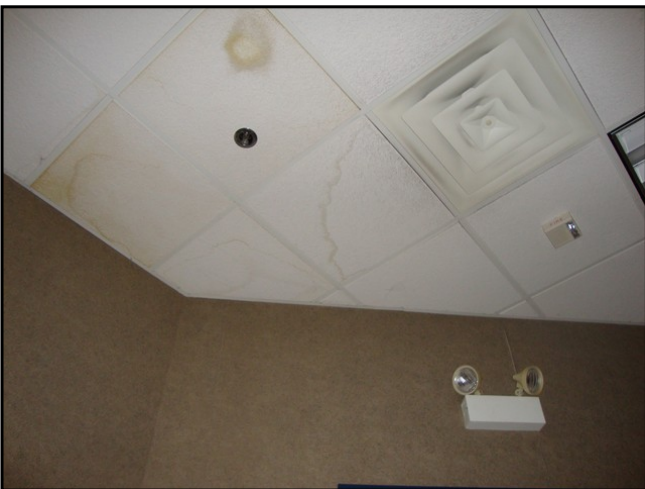
143 : Interior Defects - Hall Water Stains
