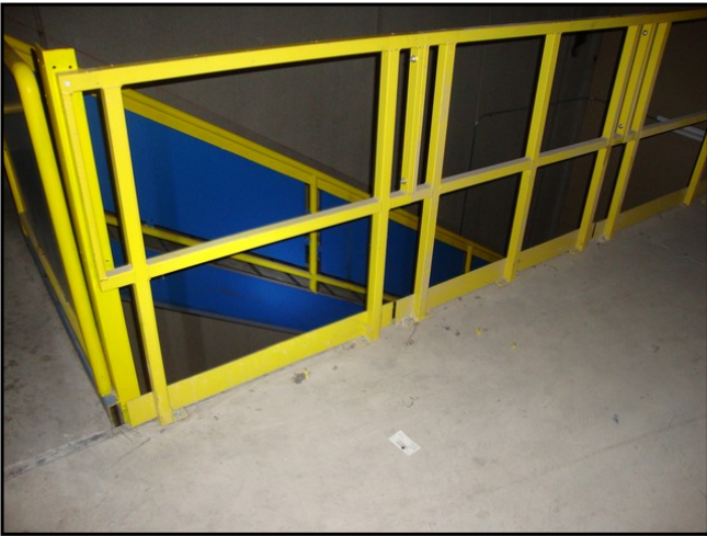
145 : Interior Defects - Missing Filler At Guard Rail 1
