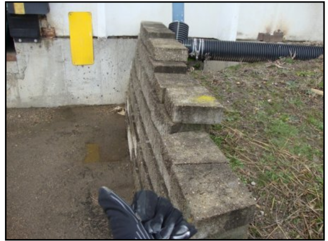
62 : Site - Retaining Wall Lateral Movement
