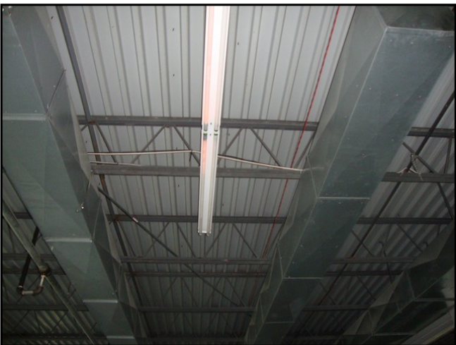
23 : Electrical - Inoperable Lights in Unfinished Office 1
