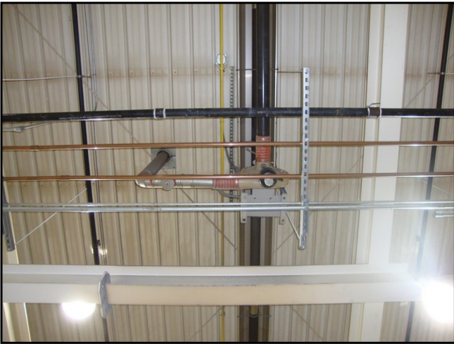
49 : Roof - Suspect Source of Leak @ Vent
