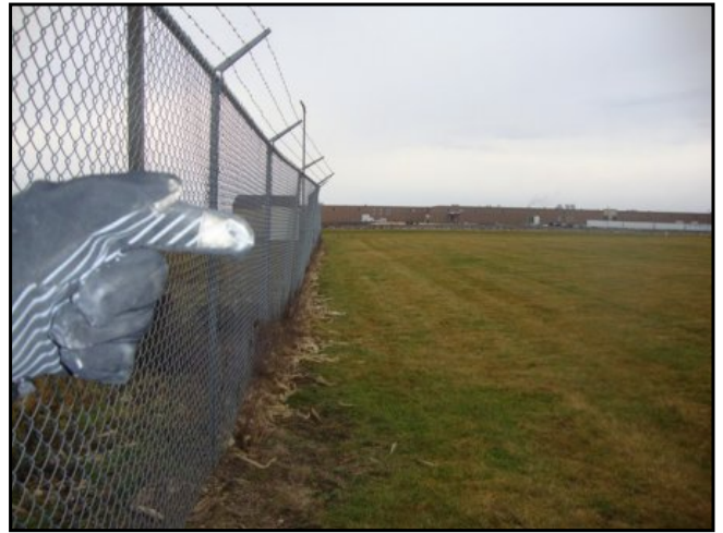
56 : Site - Minor Fence Damage
