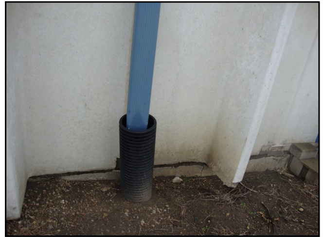
68 : Site - Storm Water Collection System 2
