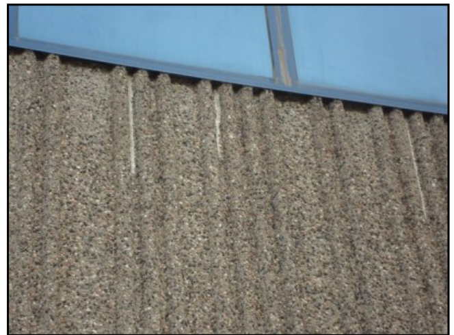
72 : Structure - Cracks Repaired With Sealant @ Office 1
