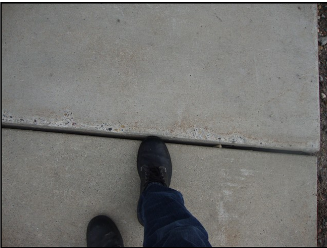
129 : Flatwork - Trip Hazard Near N13
