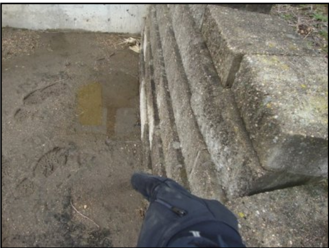
59 : Site - No Provision for Drainage at Retaining Wall
