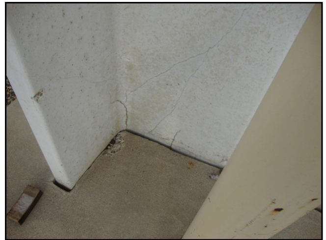
82 : Structure - Minor Cracks @ Warehouse 5
