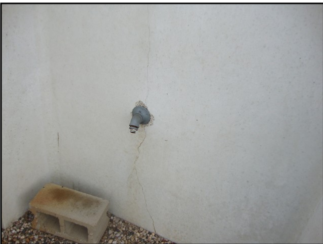
83 : Structure - Minor Cracks @ Warehouse 6
