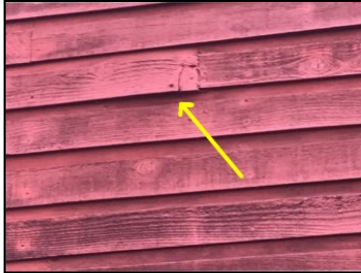
Wood siding is buckling by kitchen window.
