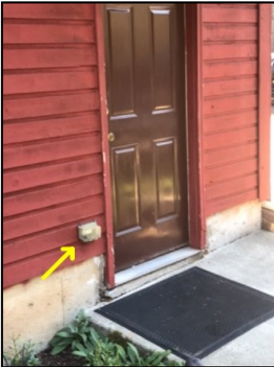
Not GFCI protected. Recommend having a licensed electrician installed one.
