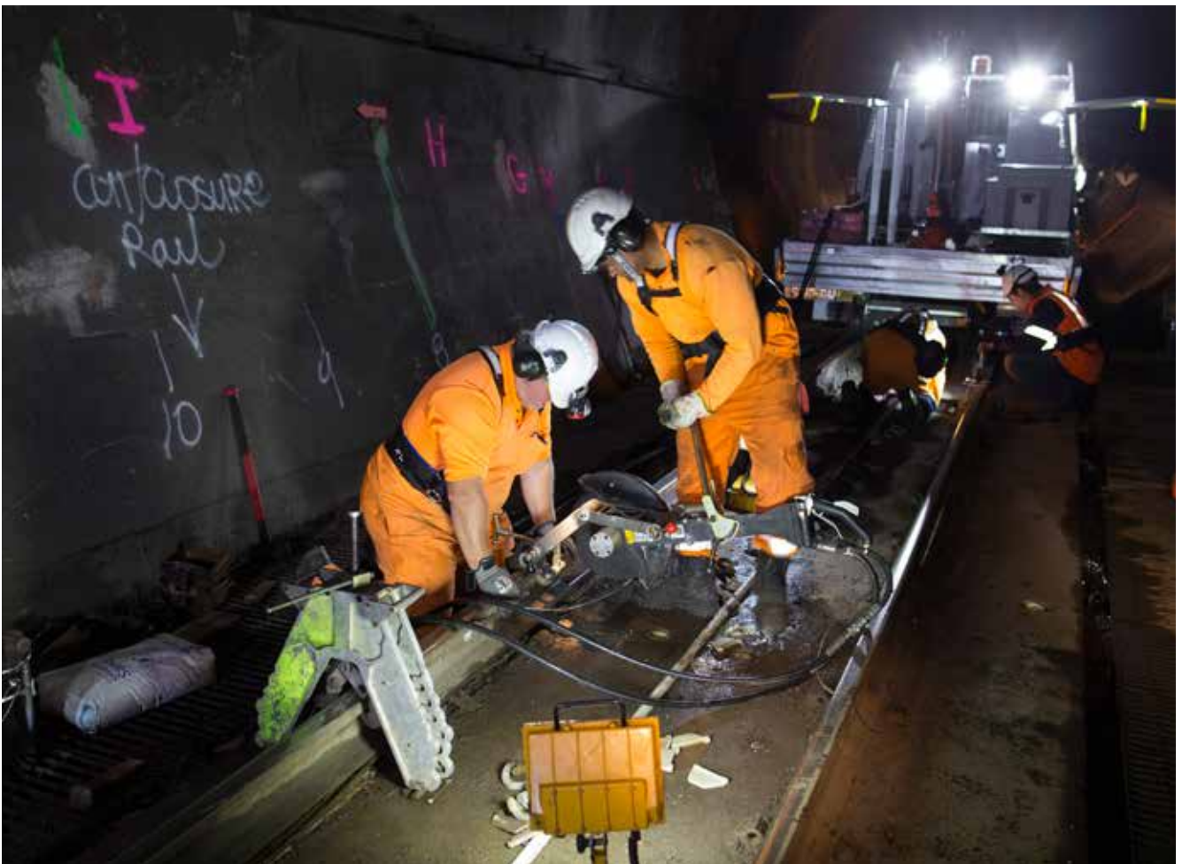
Refurbishment work being carried out in the Kaimai Tunnel in the Bay of Plenty
