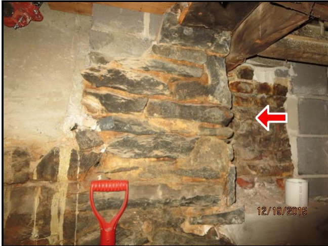
3.1 Item 1(Picture) Loose Mortar
