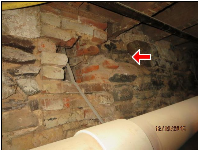
3.1 Item 3(Picture) Loose bricks
