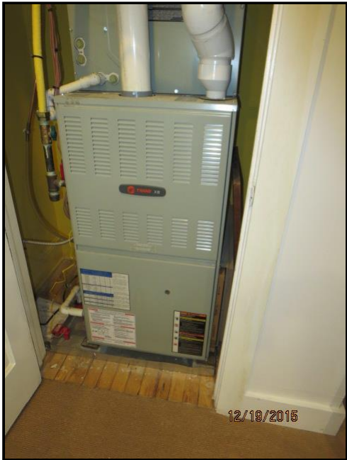
8.0 Item 3(Picture) Gas furnace
