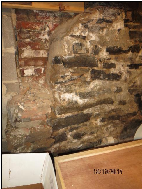
3.1 Item 7(Picture) Loose mortar
