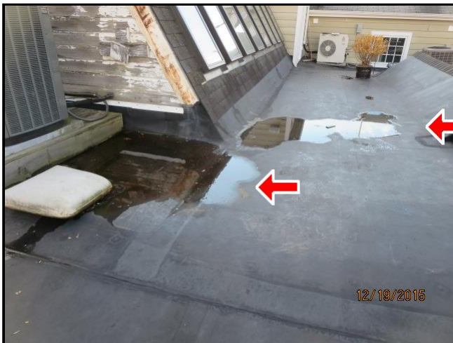
1.0 Item 1(Picture) Standing water
