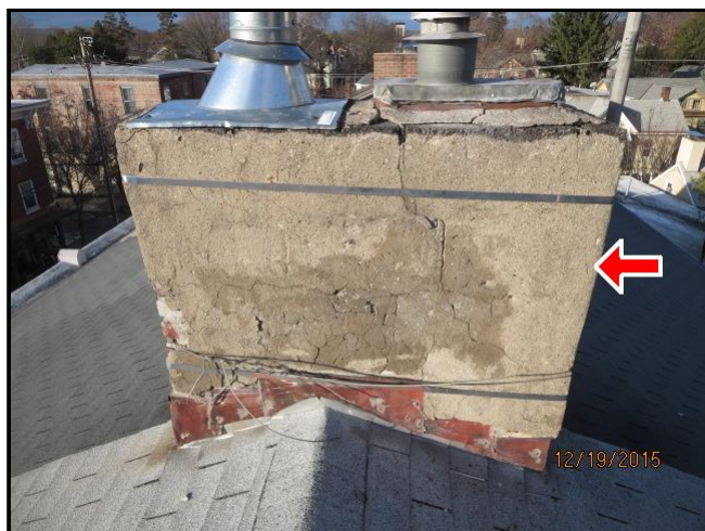
1.2 Item 1(Picture) Needs re-pointing
