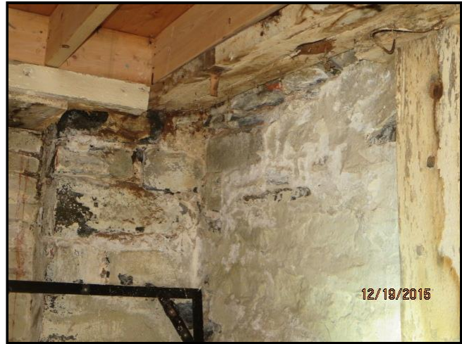
3.1 Item 6(Picture) Loose rock
