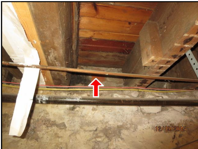
3.1 Item 8(Picture) Missing fire block
