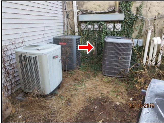
8.2 Item 1(Picture) Old unit
