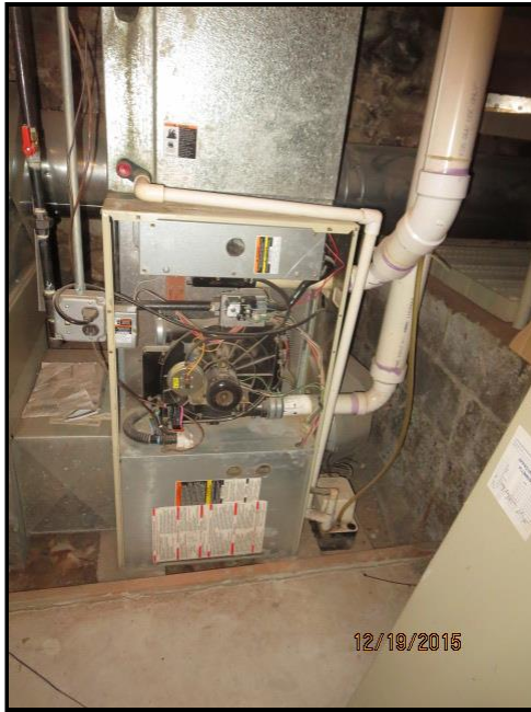
8.0 Item 2(Picture) Gas furnace
