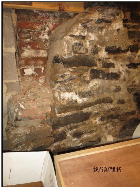
3.1 Item 7(Picture) Loose mortar
