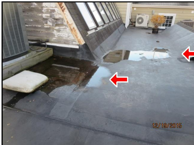
1.0 Item 1(Picture) Standing water
