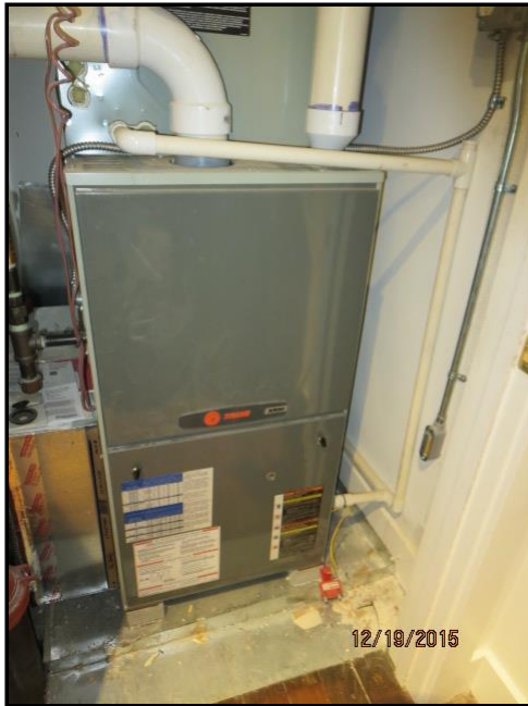
8.0 Item 4(Picture) Gas furnace
