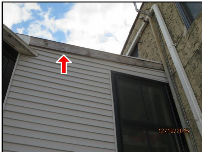
2.0 Item 1(Picture) Exposed trim
