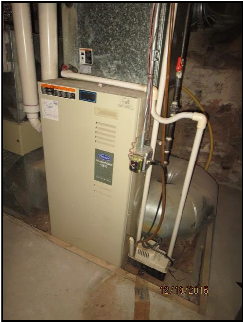
8.0 Item 1(Picture) Gas Furnace
