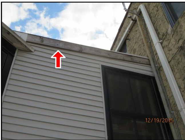
2.0 Item 1(Picture) Exposed trim
