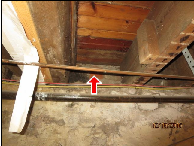
3.1 Item 8(Picture) Missing fire block
