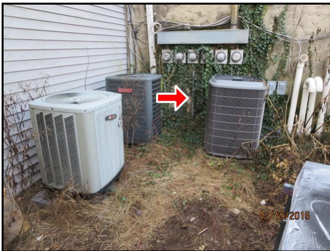
8.2 Item 1(Picture) Old unit
