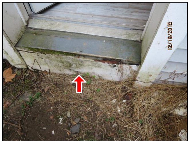
2.0 Item 2(Picture) Damaged wood
