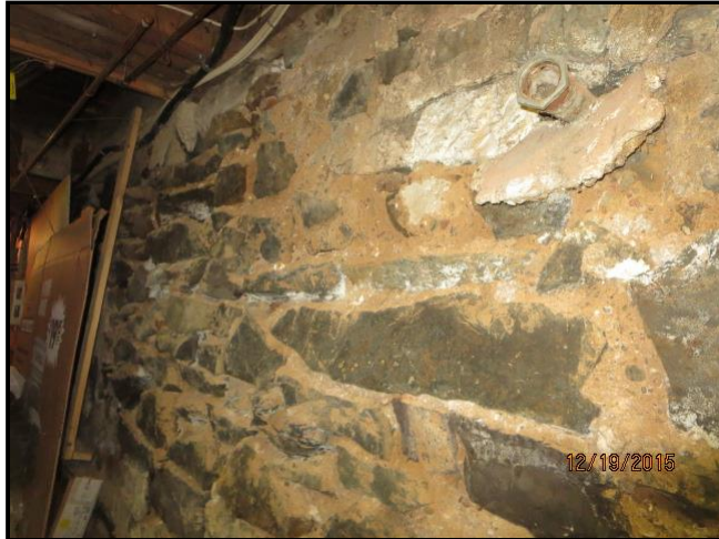
3.1 Item 5(Picture) Loose mortar
