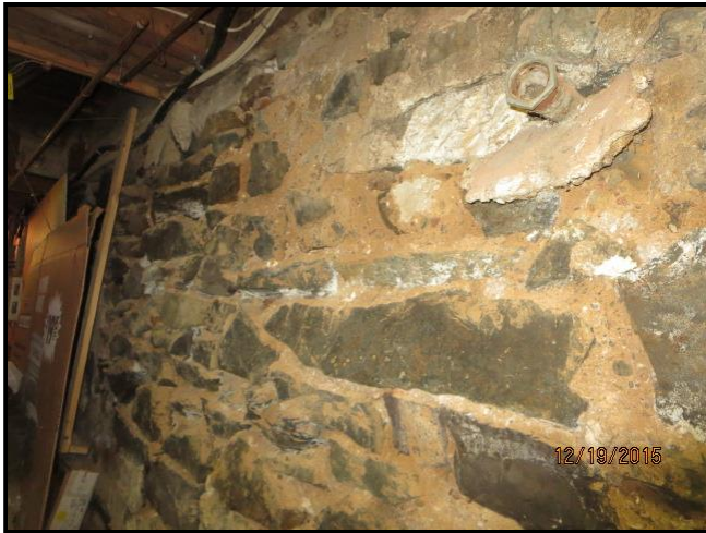
3.1 Item 5(Picture) Loose mortar
