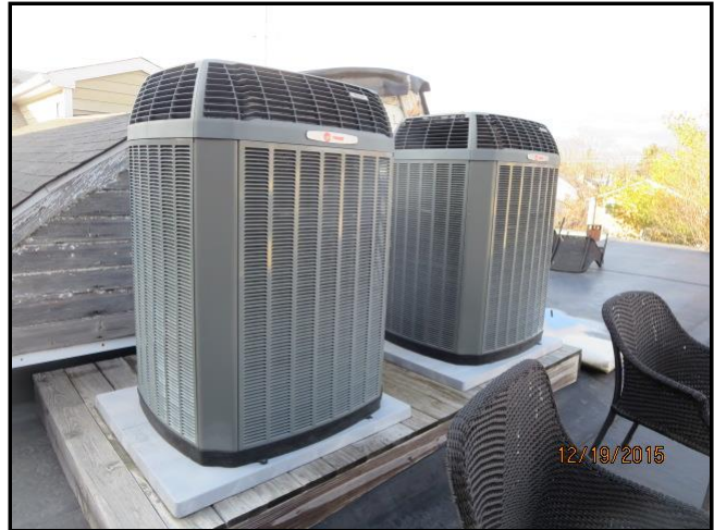
8.2 Item 2(Picture) Roof top units
