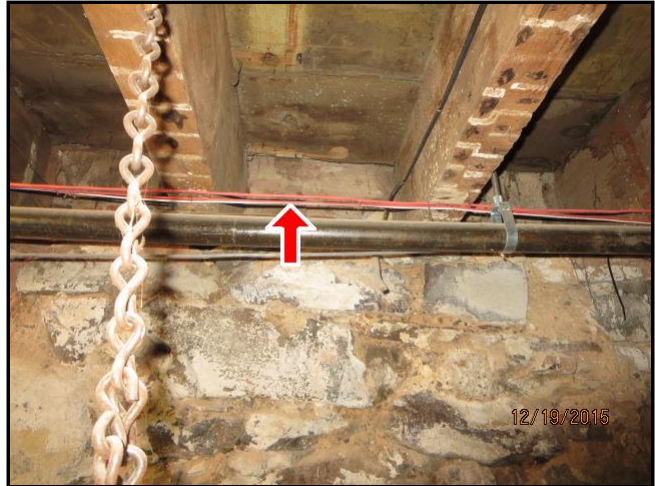
3.1 Item 9(Picture) Missing fire block
