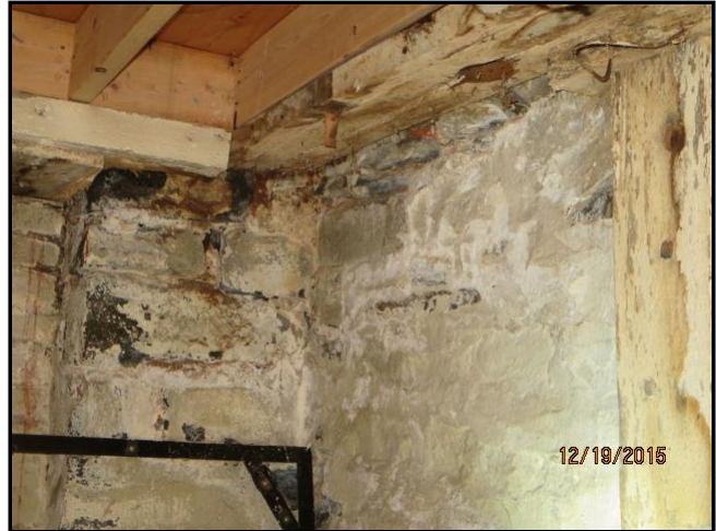
3.1 Item 6(Picture) Loose rock
