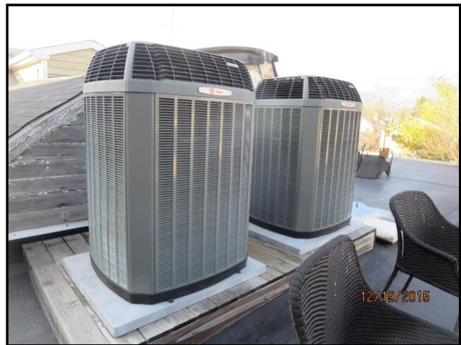
8.2 Item 2(Picture) Roof top units
