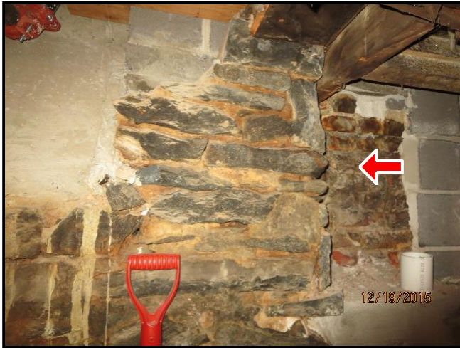
3.1 Item 1(Picture) Loose Mortar
