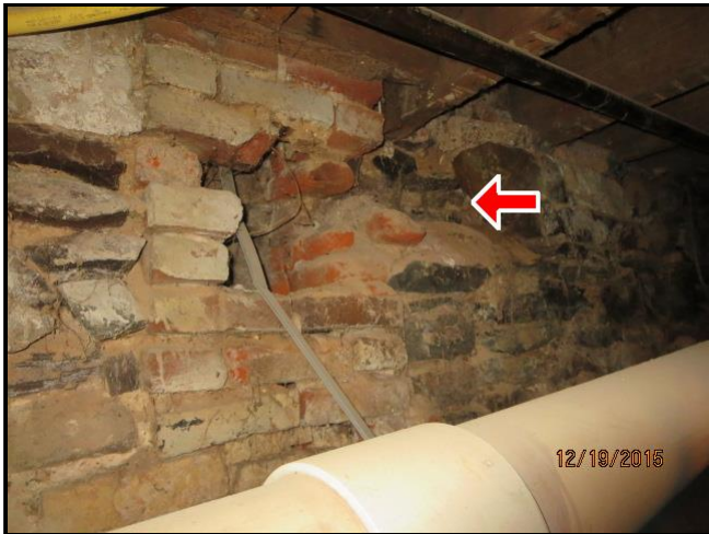
3.1 Item 3(Picture) Loose bricks
