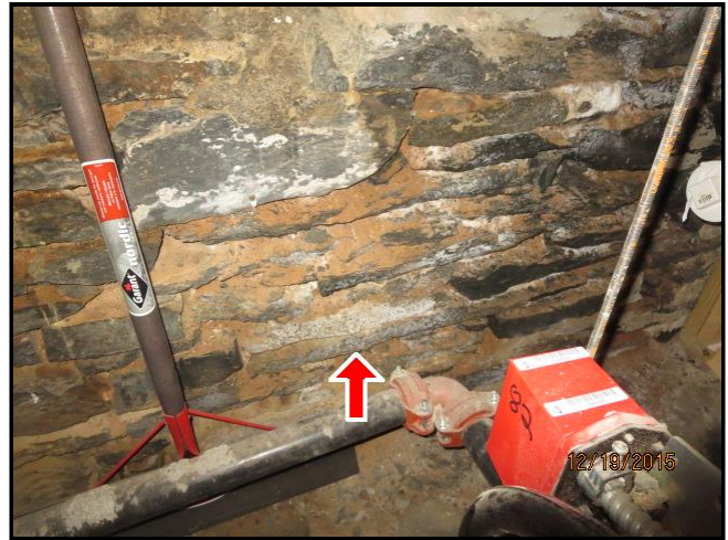
3.1 Item 2(Picture) Loose mortar
