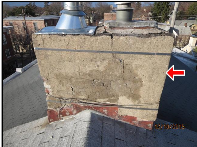
1.2 Item 1(Picture) Needs re-pointing
