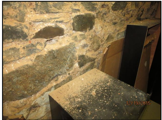
3.1 Item 4(Picture) Loose mortar
