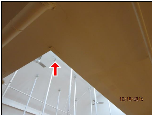
5.0.B Item 1(Picture) Water stain
