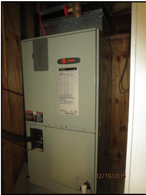
8.0 Item 5(Picture) Electric furnace
