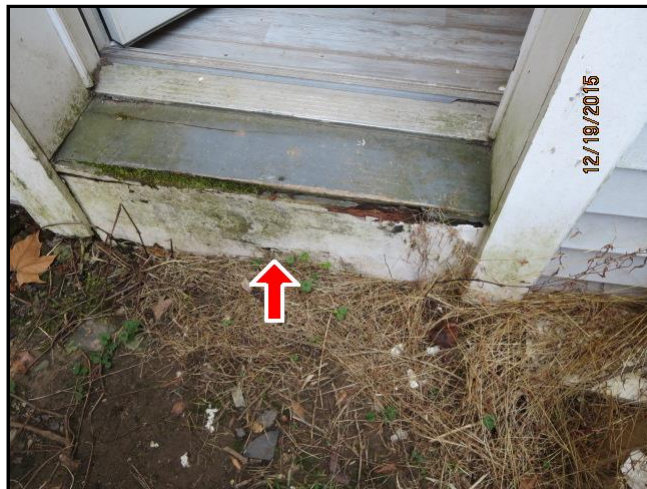
2.0 Item 2(Picture) Damaged wood
