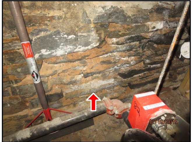
3.1 Item 2(Picture) Loose mortar
