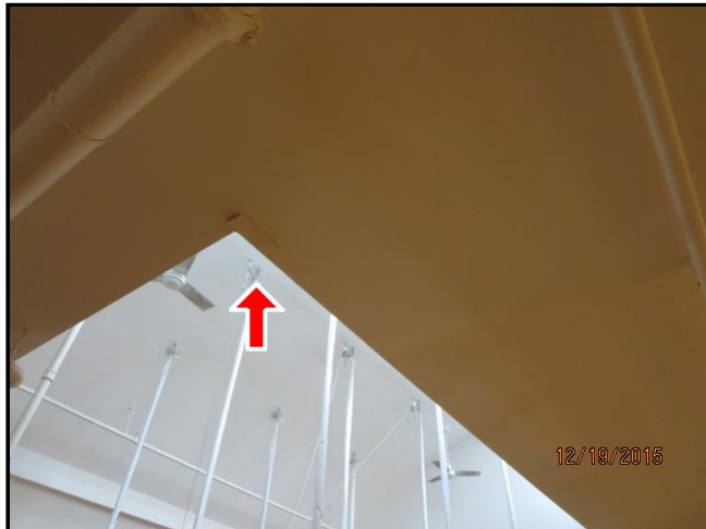
5.0.B Item 1(Picture) Water stain
