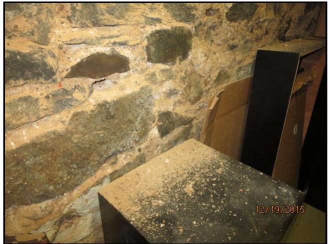
3.1 Item 4(Picture) Loose mortar
