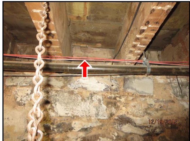
3.1 Item 9(Picture) Missing fire block
