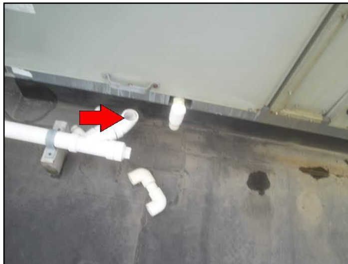
4. Missing condensate trap
