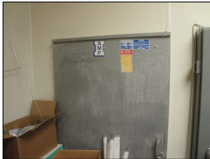
1. Storage within one meter of equipment
