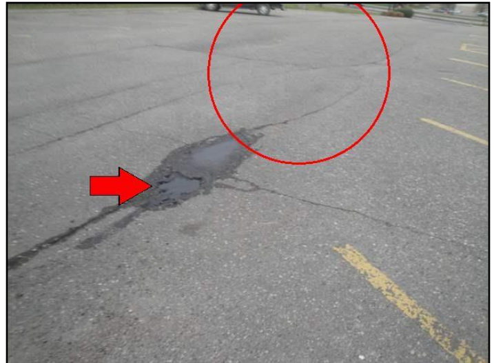
48. Parking surface in need of repair, seal...
