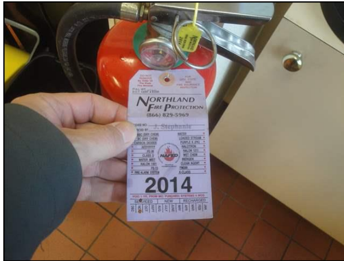
19. Fire extinguisher inspection tags were...
