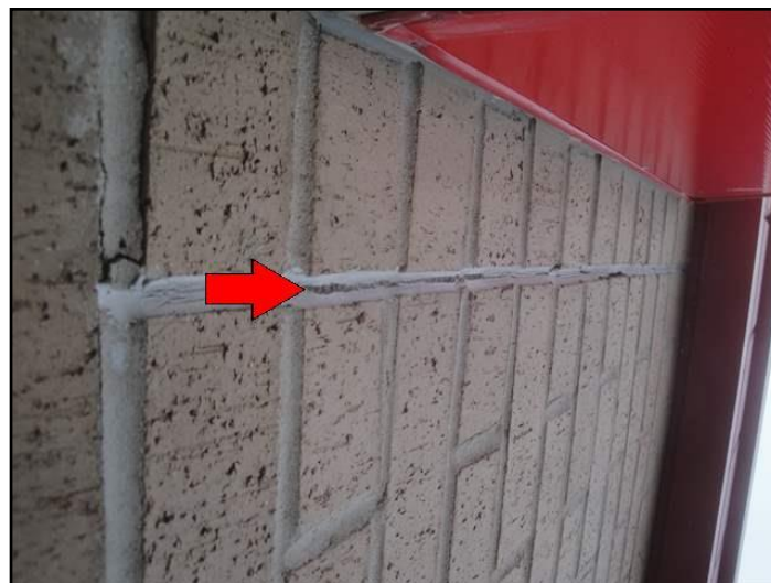
40. Deteriorated caulking wall expansion joints
