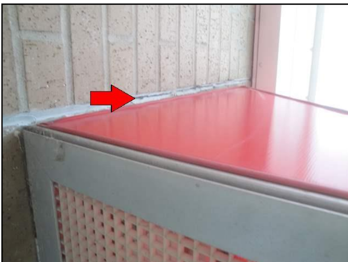
38. Deteriorated caulking wall expansion joints
