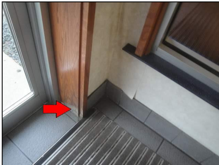
22. A water stain was noted. Refer to the...
