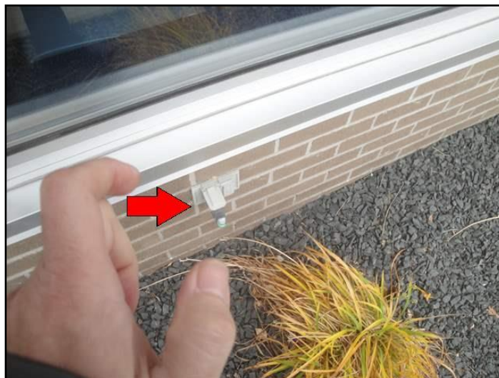
2. Electrical outlets close to a water source...
