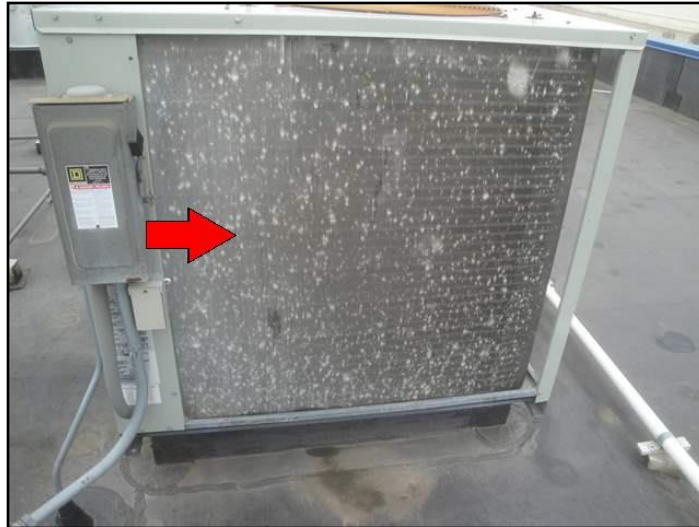
5. Condenser coil damaged / obstructed / dirty
