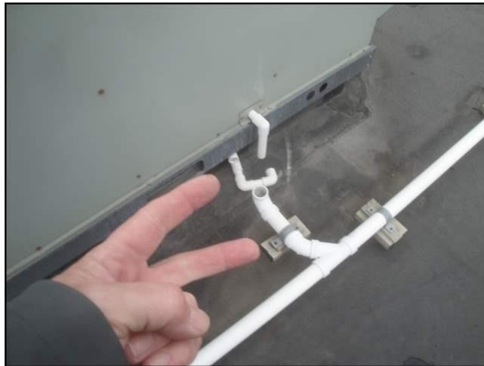
6. Missing condensate trap
