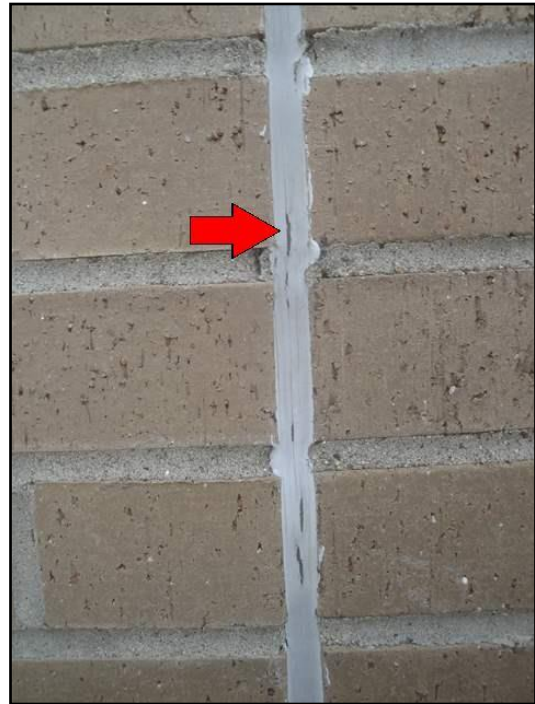
39. Deteriorated caulking wall expansion joints
