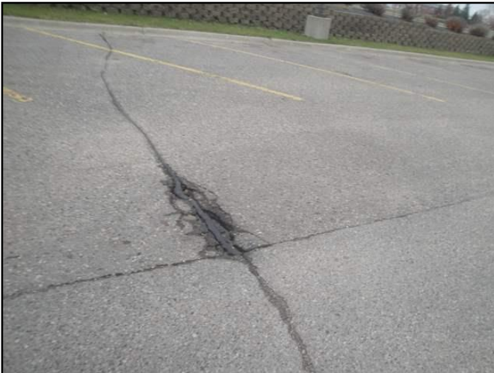
47. Parking surface in need of repair, seal...
